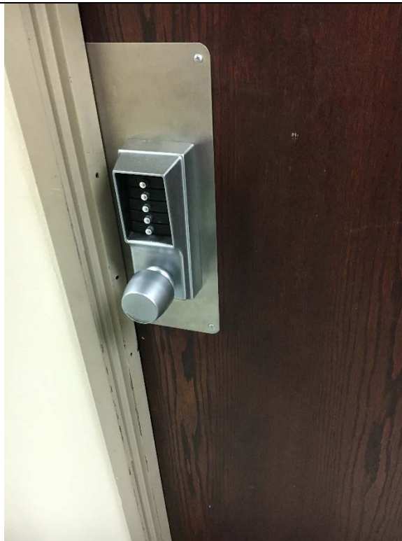
Violation 13 - Approximately 15 doors throughout the facility have door hardware that requires grasping and twisting to operate.
