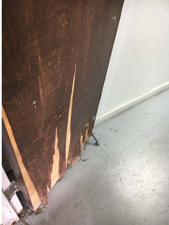
Violation 28 - Warehouse restroom door opening is only 22" wide and the door is shredded at the bottom with a door stop.
