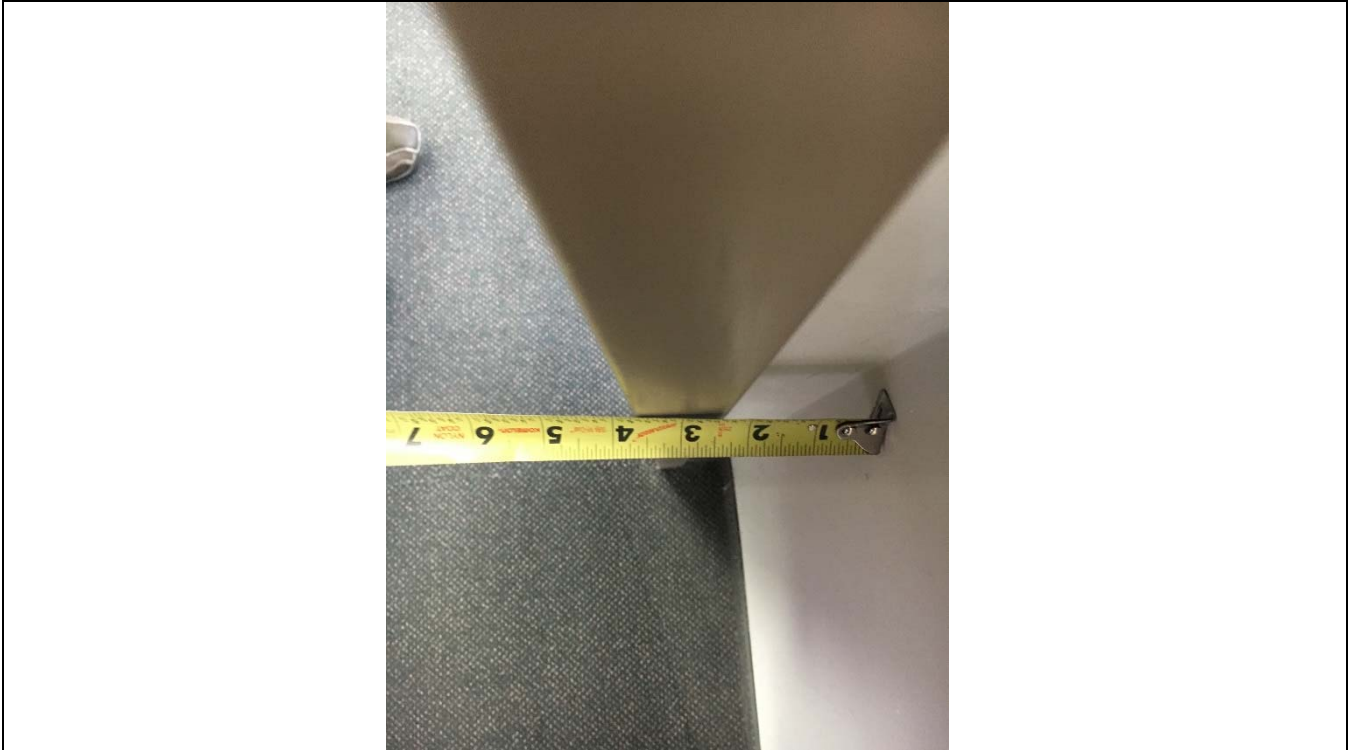
Violation 15 - There are approximately 8 doors throughout the building (including private offices) that do not have a minimum of 18" maneuvering clearance on the pull side.
