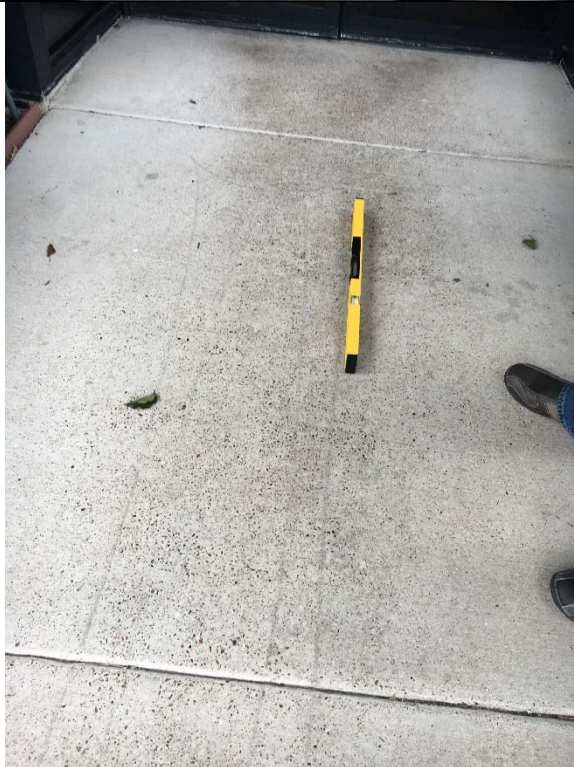
Violation 7 - The sidewalk leading up to the side entrance from the runway area has a 10.7% running slope.
