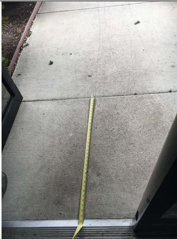
Violation 6 - There is only a 33-1/2" deep level landing/maneuvering clearance at the side door that leads to the runway area. The maneuvering clearance at this door should be a minimum of 60" deep.
