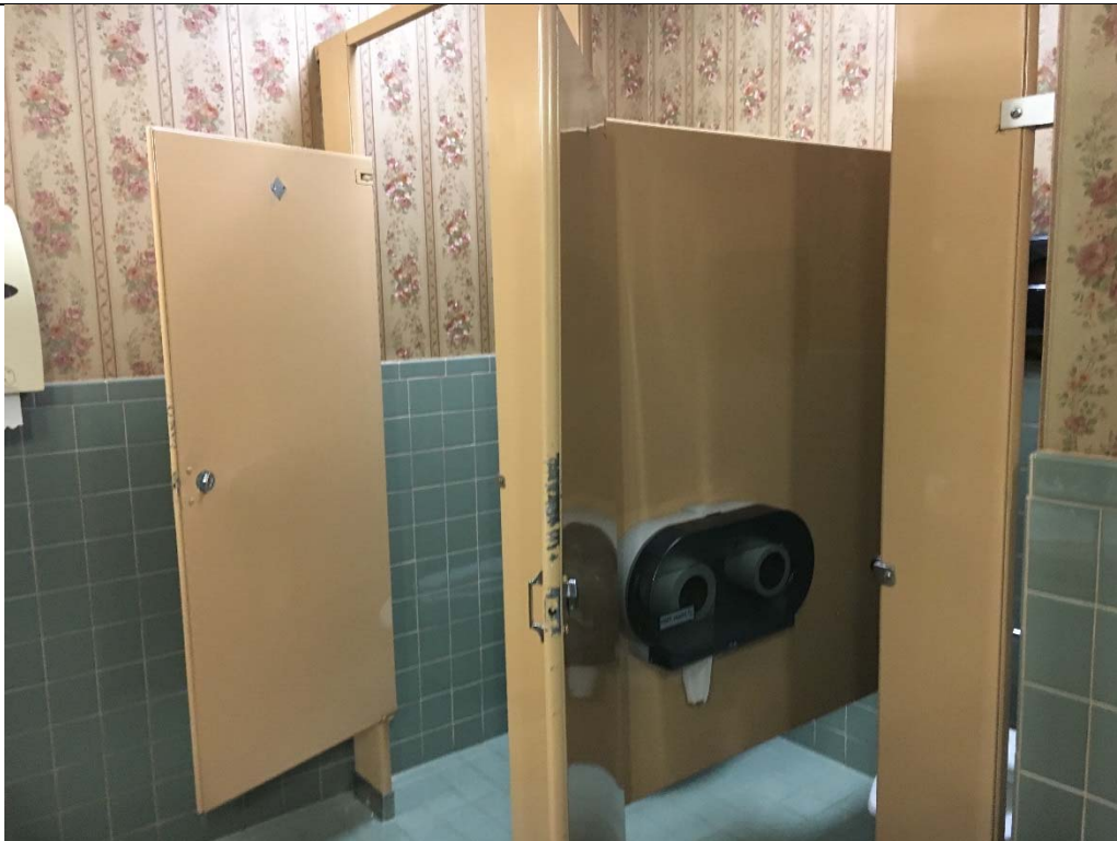
Violation 26 - Second Floor Women's room - Does not have an accessible stall provided.
