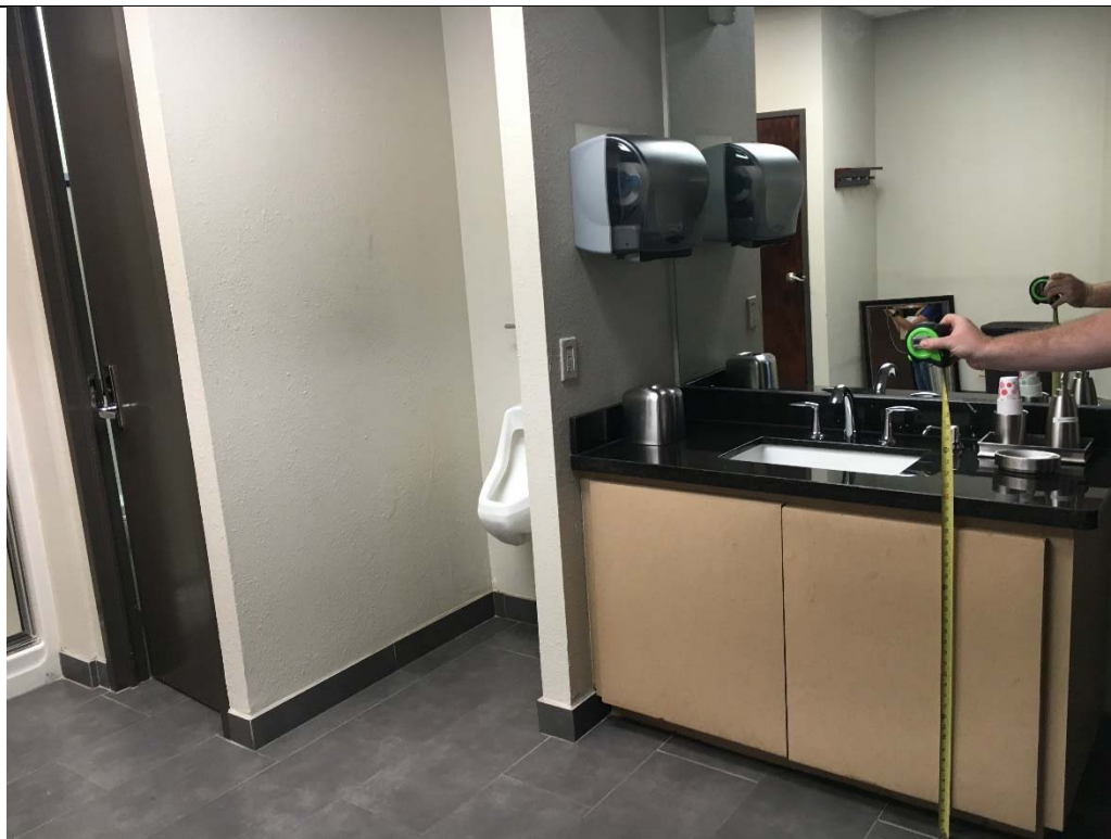
Violation 18 - The lavatory in the lounge restroom does not have the required toe and knee clearance provided.
