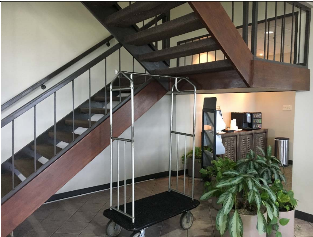
Violation 4 - There is no accessible route leading to the second floor.
