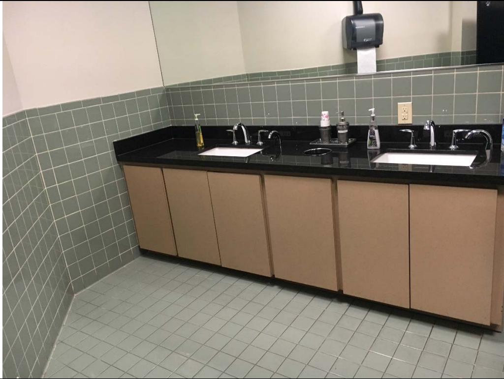
Violation 21 - First Floor Men's room - Lavatory does not have the required toe and knee clearance provided.
