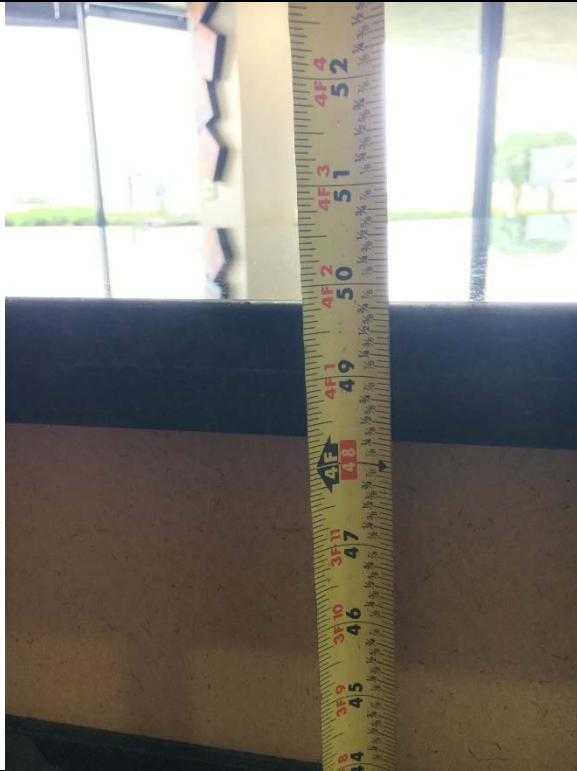
Violation 12 - The information desk is at 49-3/4" to the top where a maximum of 36" is required.
