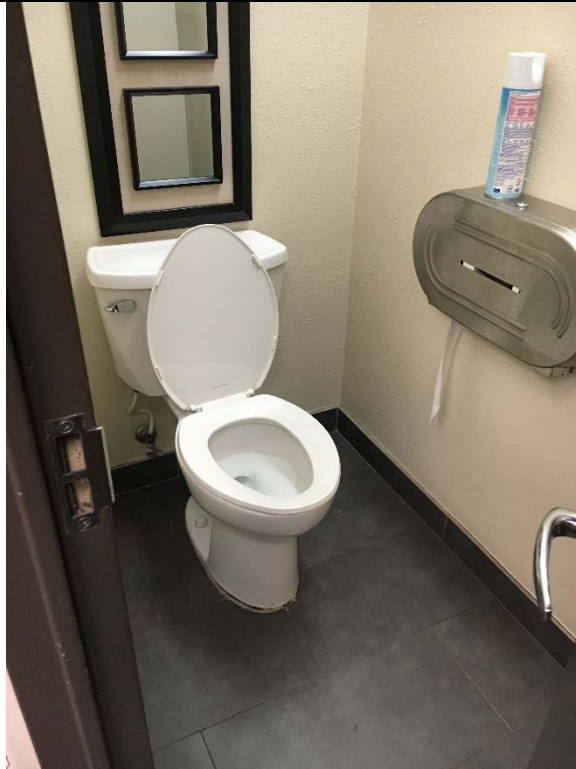
Violation 19 - The lounge restroom does not have an accessible stall provided.
