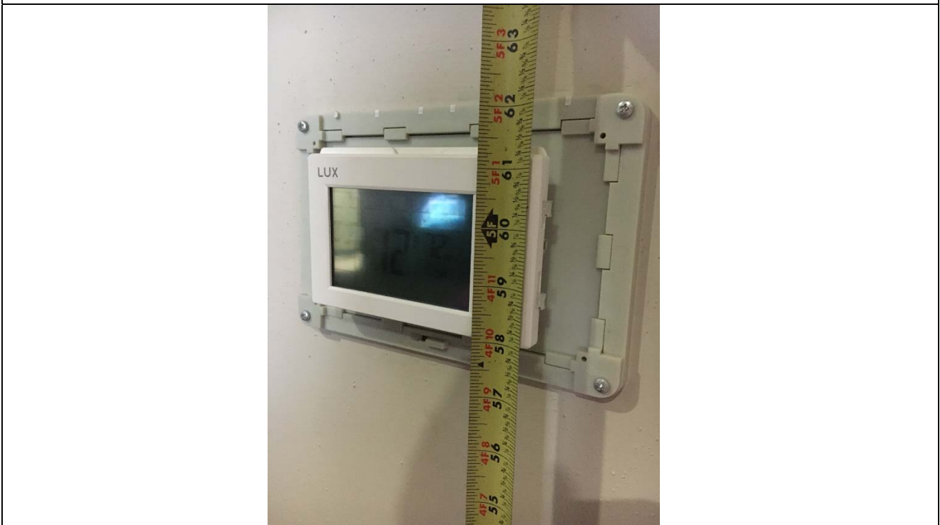
Violation 16 - The controls for the thermostat provided in the lounge area are at 60" above finished floor.
