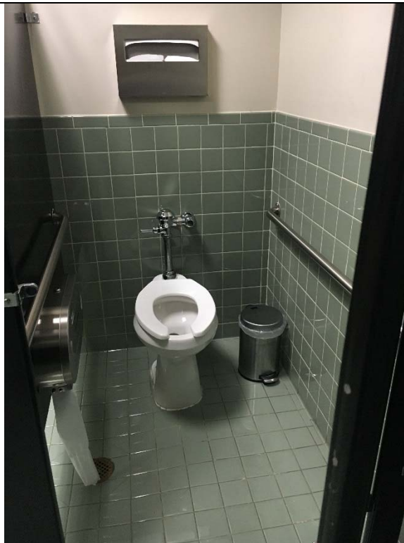
Violation 20 - First Floor Men's room - Does not have an accessible stall provided.
