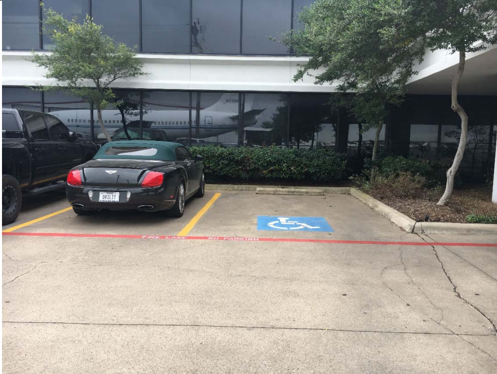
Violation 1 - Only one accessible parking space is provided where two are required and one of the two is required to be van accessible.
