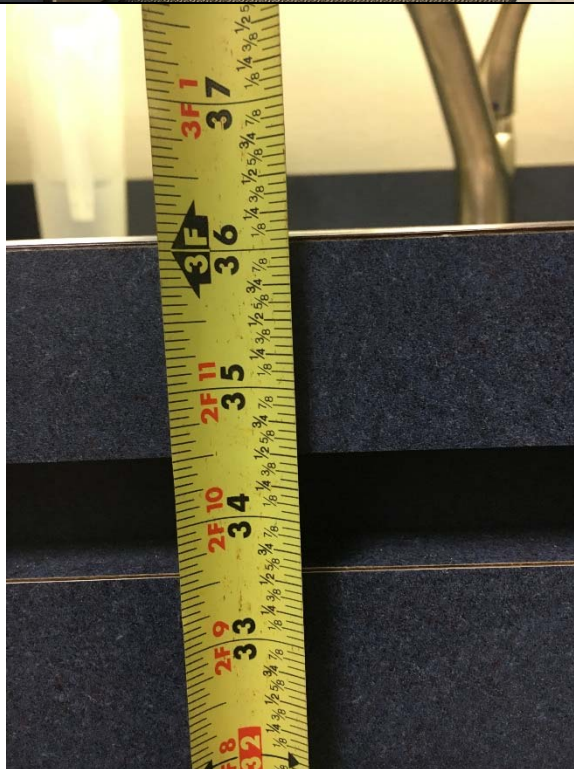
Violation 37 - The counter in the 2nd floor break room in the AmeriStar office is 36-1/8" high where a maximum height of 34" is required.
