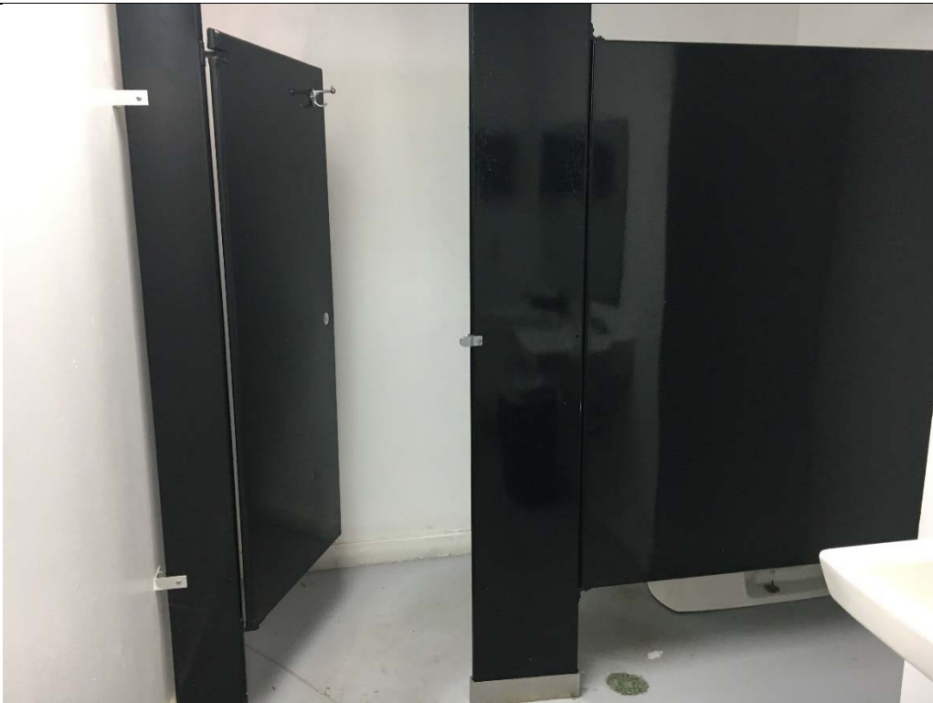
Violation 29 - The warehouse restroom does not have an accessible stall.
