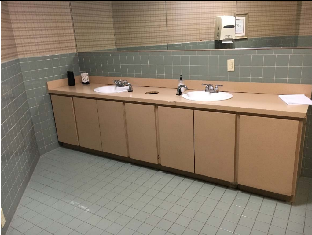
Violation 25 - Second Floor Men's room - Lavatory does not have the required toe and knee clearance provided.
