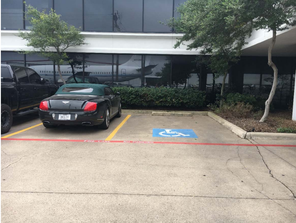
Violation 3 – There is no accessible parking signage provided.
