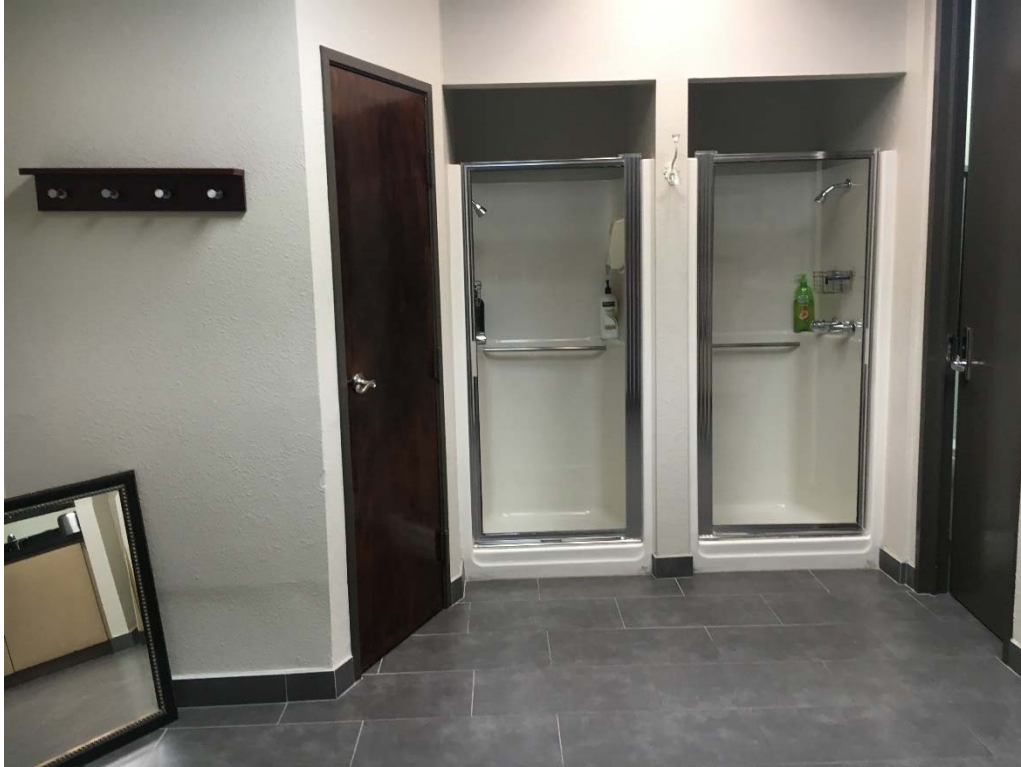
Violation 17 - There are two showers in the lounge restroom, neither of which are compliant.
