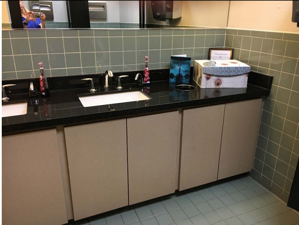
Violation 23 - First Floor Women's room - Lavatory does not have the required toe and knee clearance provided.
