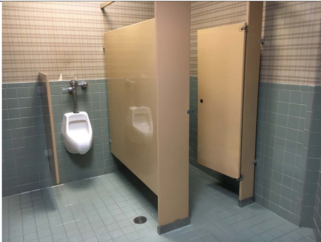
Violation 24 - Second Floor Men's room - Does not have an accessible stall provided.
