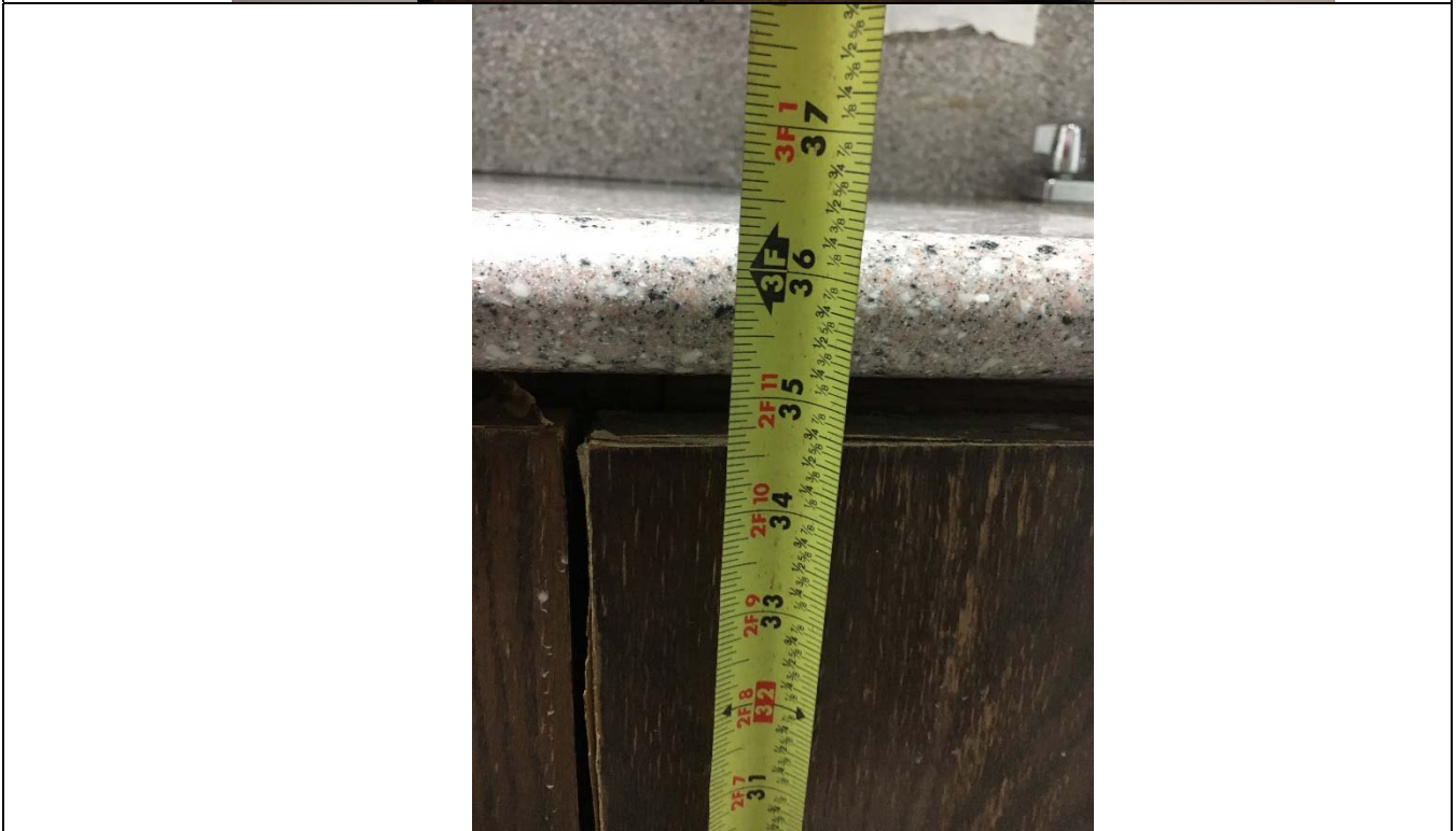
Violation 34 - The counter in the second floor break room is at 36-3/8" high where 34" maximum is required.
