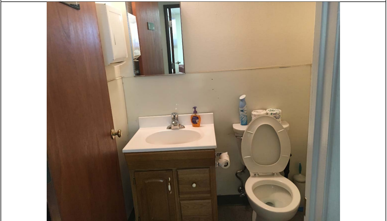
Violation 8 - The Men's restroom is too small and does not have the required turning radius provided.
