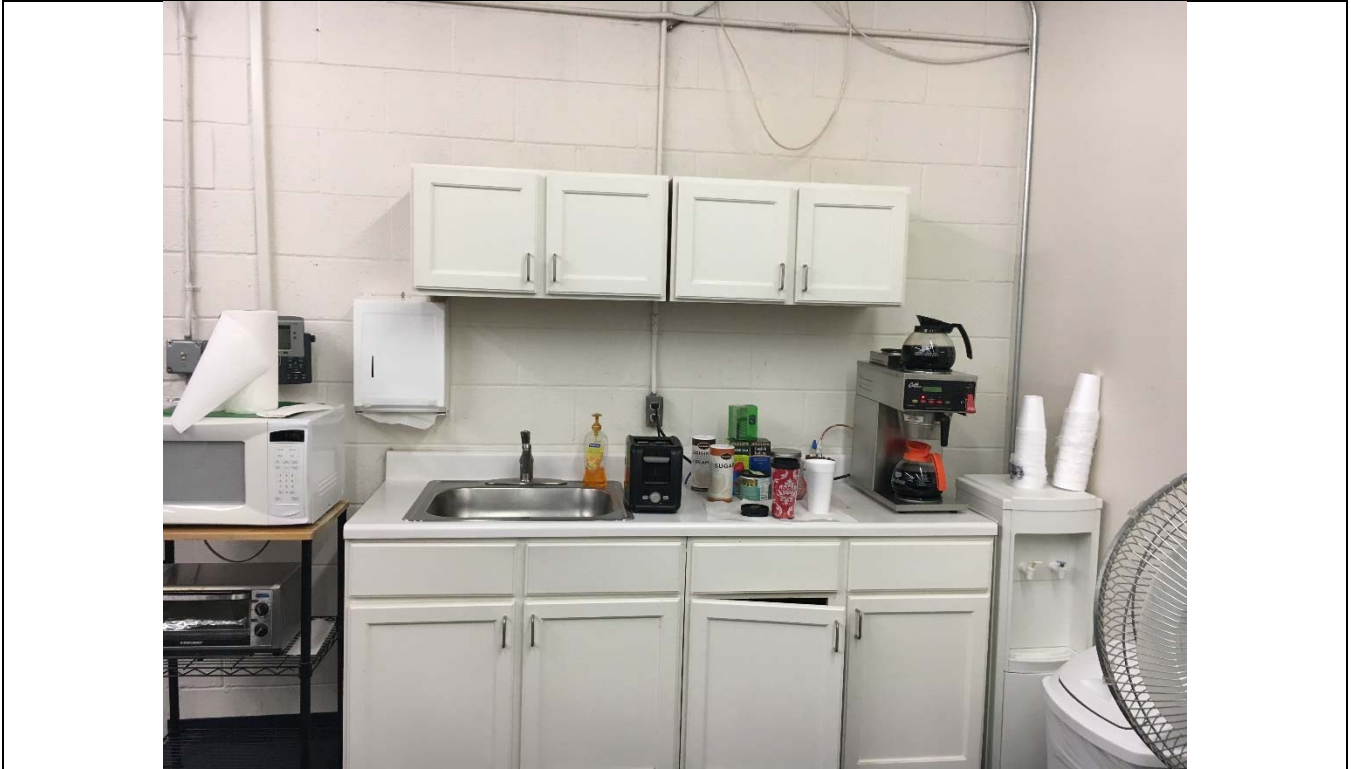
Violation 11 - The breakroom sink is at 35-1/2" high where 34" maximum is required.
