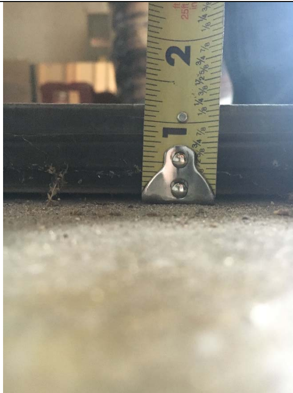
Violation 6 - The storage room in the warehouse has a 1-3/16" step to enter.
