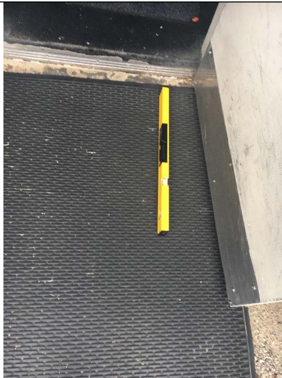
Violation 6 - The landing at the main entrance into the building has a 4% slope running up to it.
