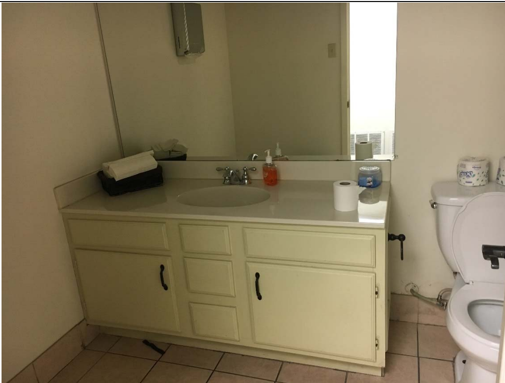
Violation 16 - The Men's restroom on the second floor is too small and does not have the required turning radius provided.
