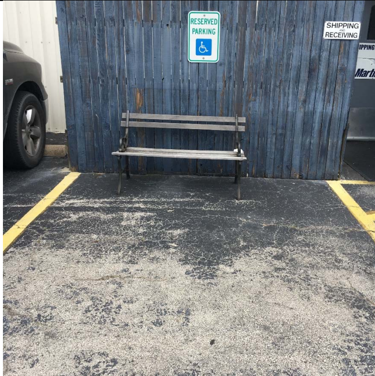
Violation 1 - The left accessible space has a bench sitting in it blocking access for a vehicle to park.
