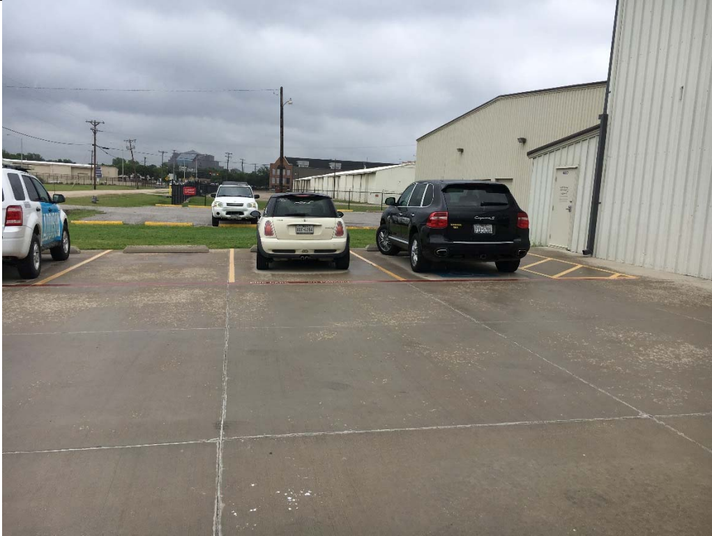
Violation 1 - There is an accessible parking space, but no signage is provided.
