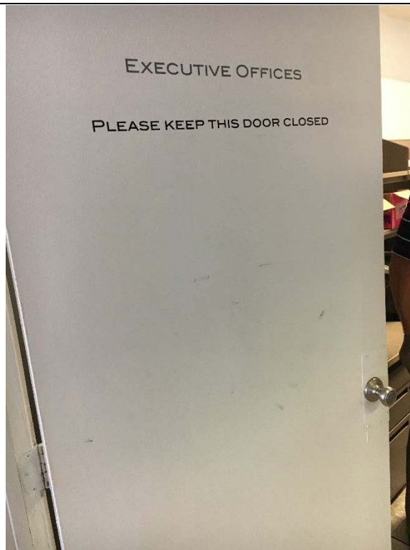
Violation 2 - The door into the Executive Offices has knob style door hardware requiring grasping and twisting to operate.
