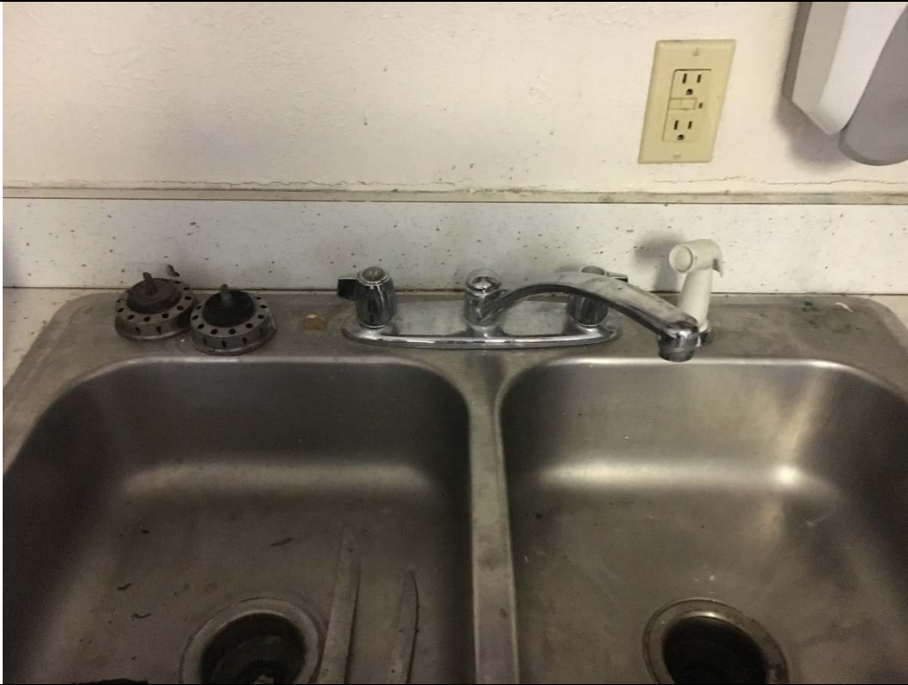
Violation 22 - Breakroom sink faucets require grasping and twisting to operate.
