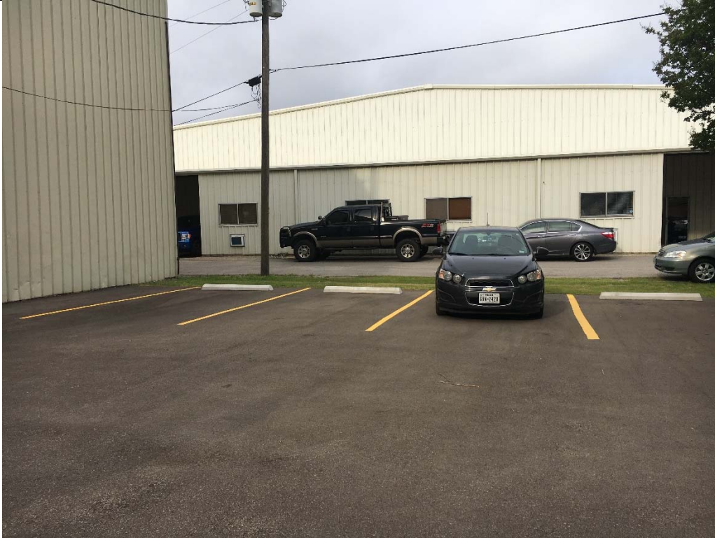
Violation 1 - Four parking spaces serve this building, none of which are accessible.
