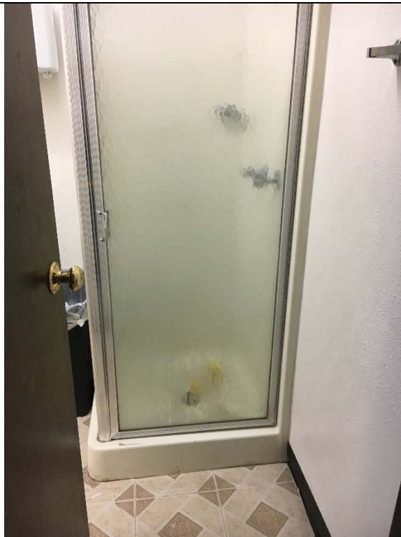
Violation 20 - There is a shower provided in the restroom that has no accessible features.
