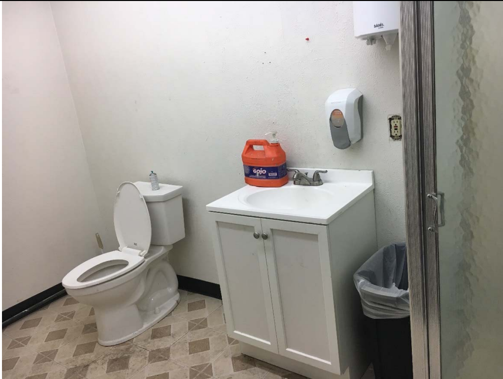
Violation 19 - The restroom does not include any accessible features and the room is not large enough to accommodate accessible fixtures and wheelchair turning space.
