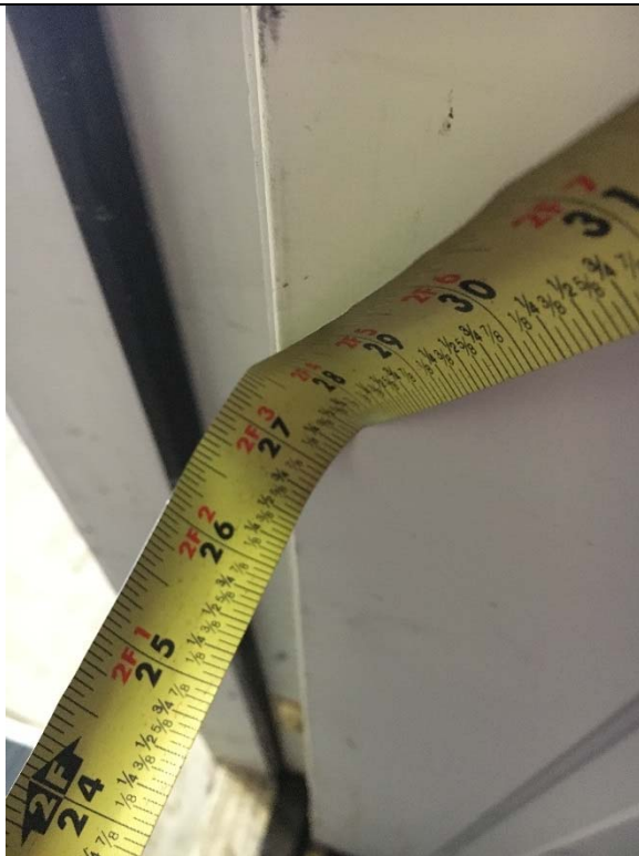
Violation 9 - The entrance door into the main portion of the office only has a 27" wide opening.
