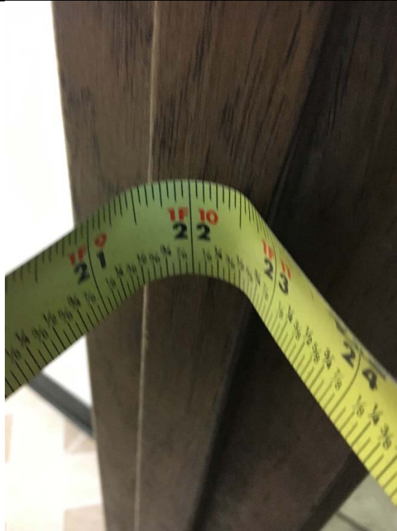
Violation 17 - The restroom door only provides 22" clear width where 32" minimum is required.
