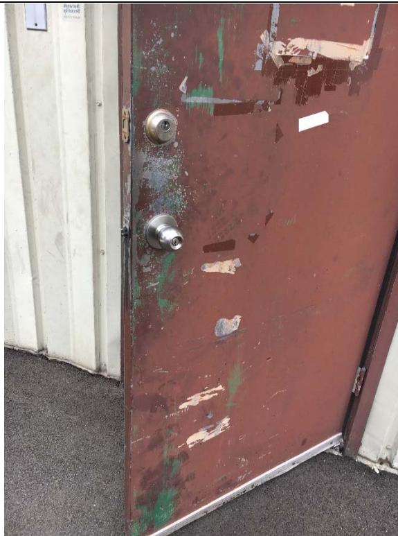
Violation 2 - The main entrance door into the building has knob door hardware requiring grasping and twisting to operate.
