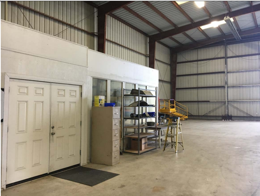
Violation 4 - The entrance door into the storage portion of the office pod has knob style door hardware requiring grasping and twisting to operate.
