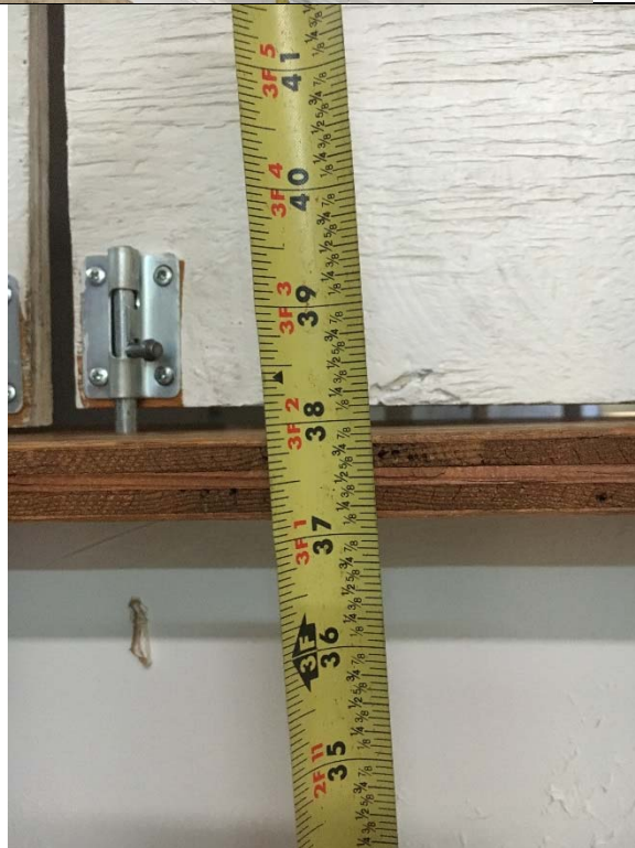
Violation 14 - There is a counter that is 38" to the top where 36" is the maximum allowed.
