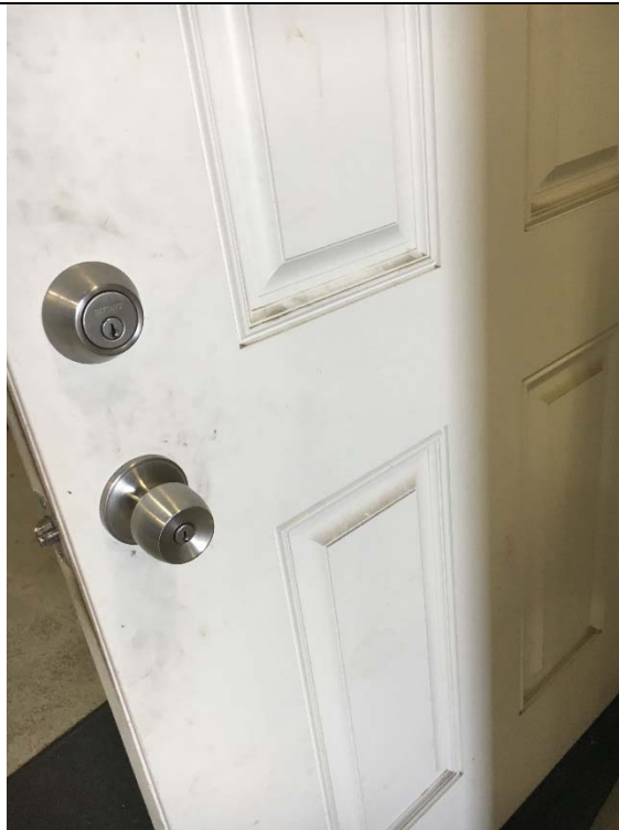
Violation 7 - The entrance into the main portion of the office pod has door hardware that requires grasping and twisting to operate.
