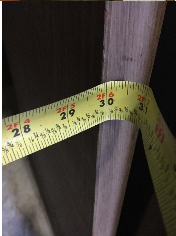
Violation 5 - The entrance door into the storage portion of the office pod only has a 30" opening.
