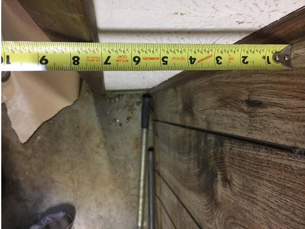
Violation 6 - The door exiting from the storage portion of the office pod only has a 8-1/2" maneuvering clearance on the pull side.
