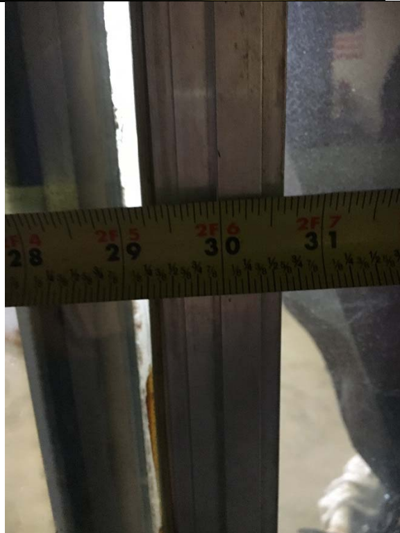
Violation 13 - Sliding glass doors exiting the storage room only have a 30" opening.
