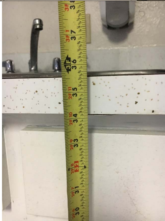
Violation 21 - The break room sink is 35-3/4" high where 34" maximum is required.
