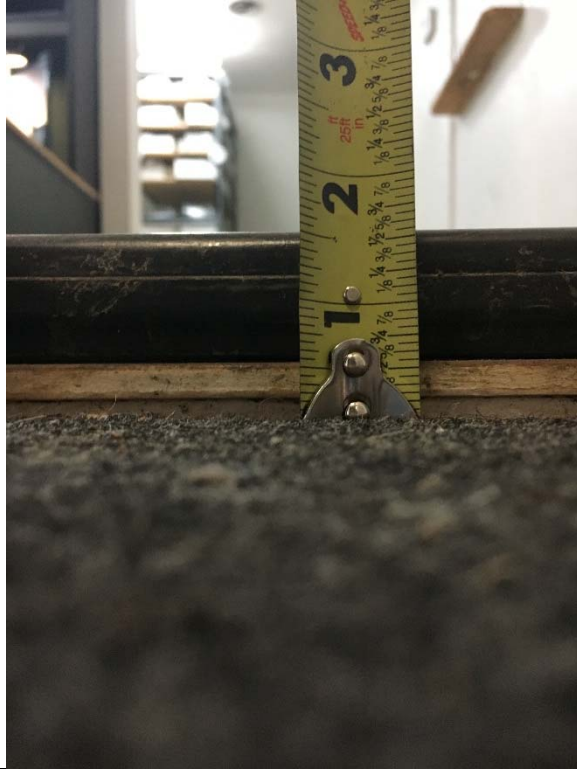
Violation 8 - The entrance into the main portion of the office pod requires a 1-1/2" step up to enter.
