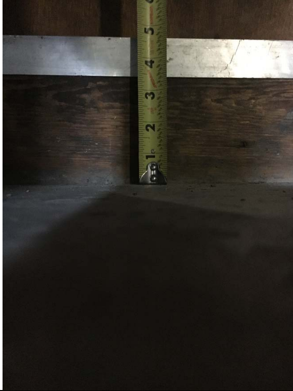
Violation 5 - There is a 5" step up to enter the office pod.
