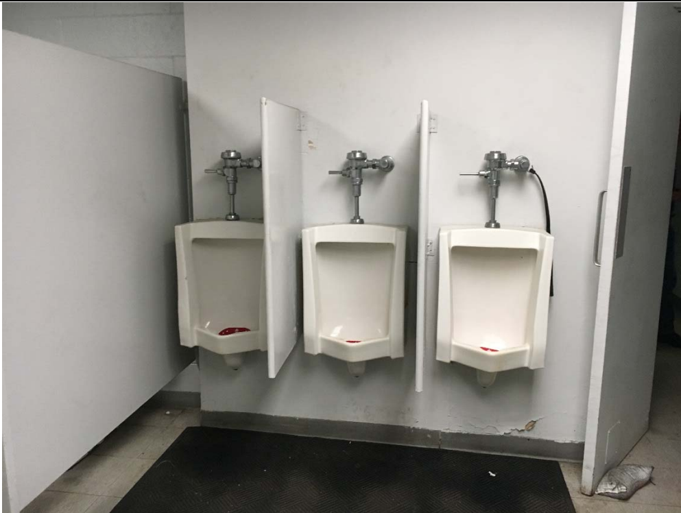
Violation 6 - Men's Restroom: There are 3 urinals, none of which are compliant.
