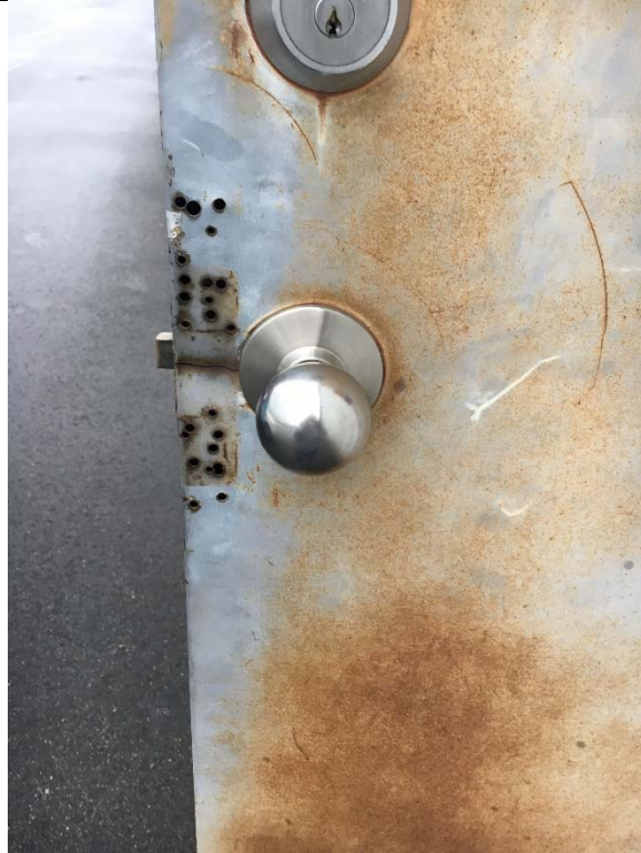
Violation 1 - Entrance door has knob hardware requiring grasping and twisting to operate.
