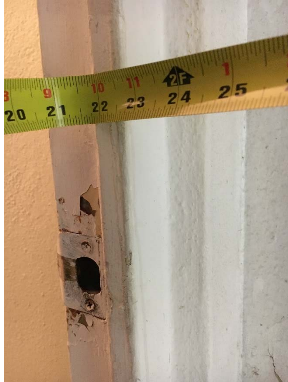
Violation 10 - Women's Restroom: Door opening is only 22" wide.
