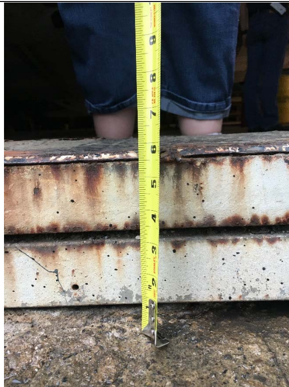
Violation 2 - There is a 5-3/16" step up to enter the building.
