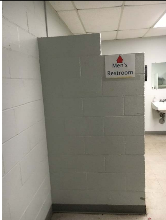
Violation 3 - Men's Restroom: Signage is not compliant. It is a piece of paper mounted inside the restroom with no Braille or tactile characters.
