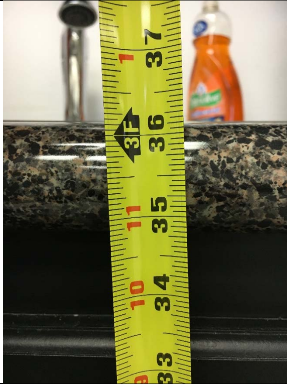
Violation 12 - The counter in the breakroom is at 36" above finished floor.
