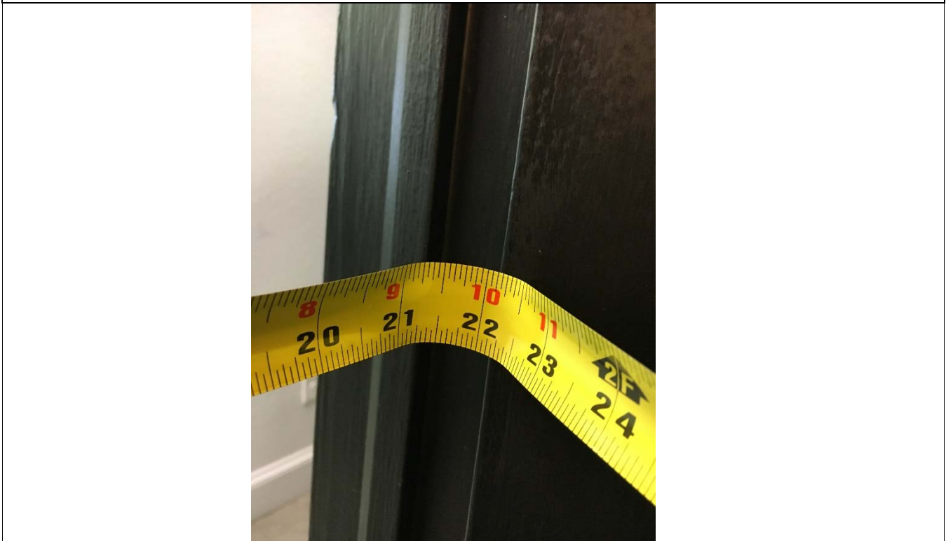
Violation 9 - Men's and Women's Restrooms: Doors are only 22" wide.
