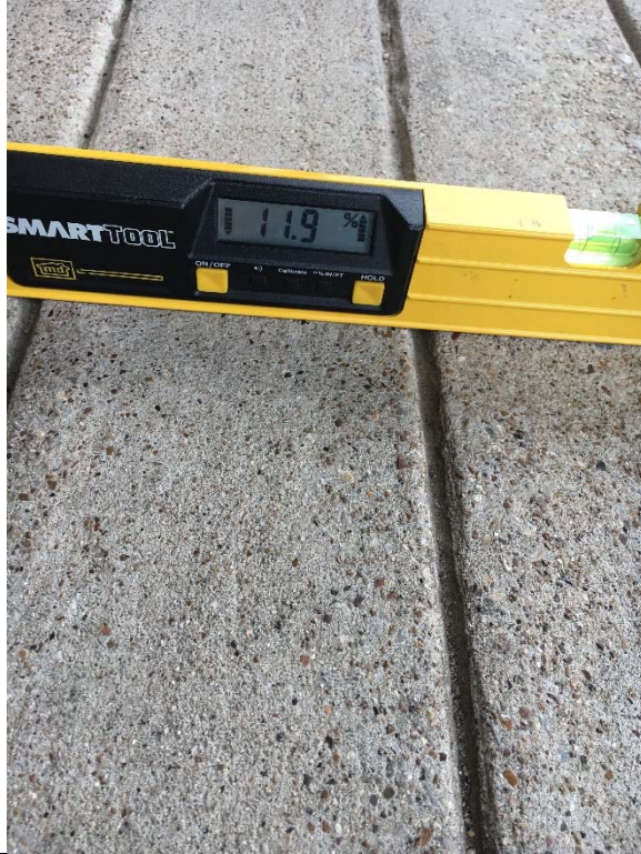
Violation 1 -The entrance into Hanger #2 has a 11.9% slope at the door.
