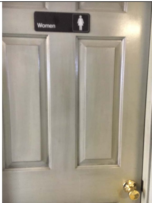
Violation 4 - Restroom doors have knob hardware requiring grasping and twisting to operate.
