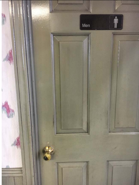
Violation 3 - Restroom signage is mounted on the door.
