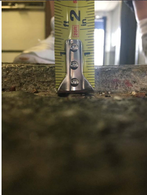
Violation 2 - The entrance into the office area from the warehouse has a 5/8" change in level.
