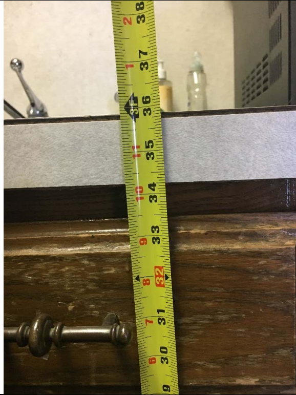
Violation 8 - The sink in the break rea is 35-13/16" high where 34" maximum is required.
