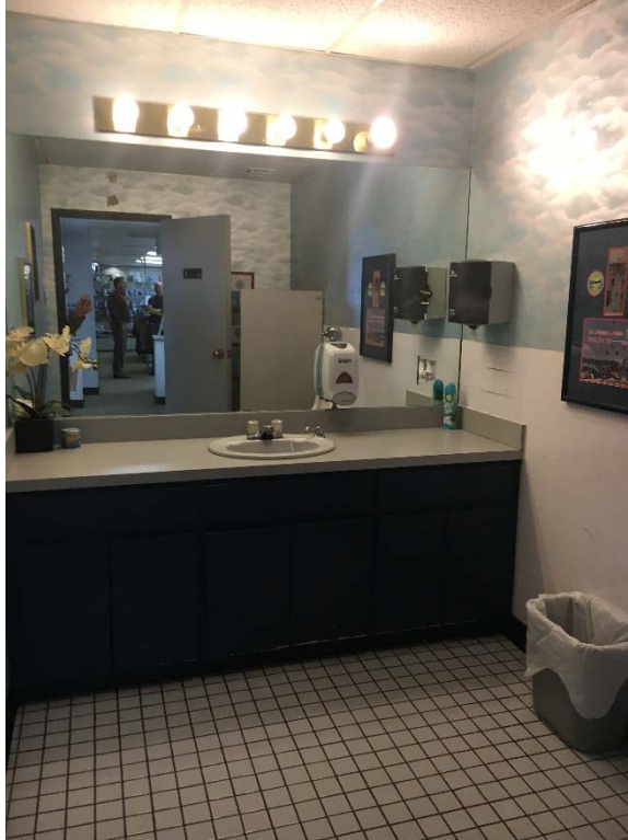
Violation 15 - Men's Room: The lavatory does not have the required knee clearance provided.
