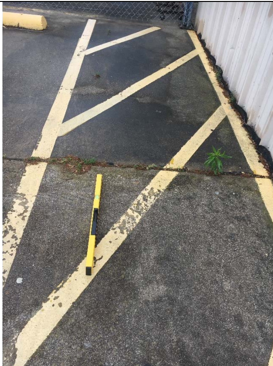
Violation 3 - The expansion joint that runs from the parking space through the access aisle has grass growing up through it.
