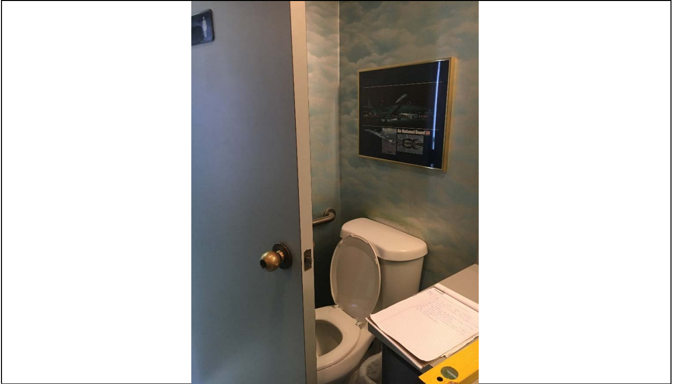
Violation 19 - Women's Room: The lavatory encroaches on the required clear floor space width for the water closet.
