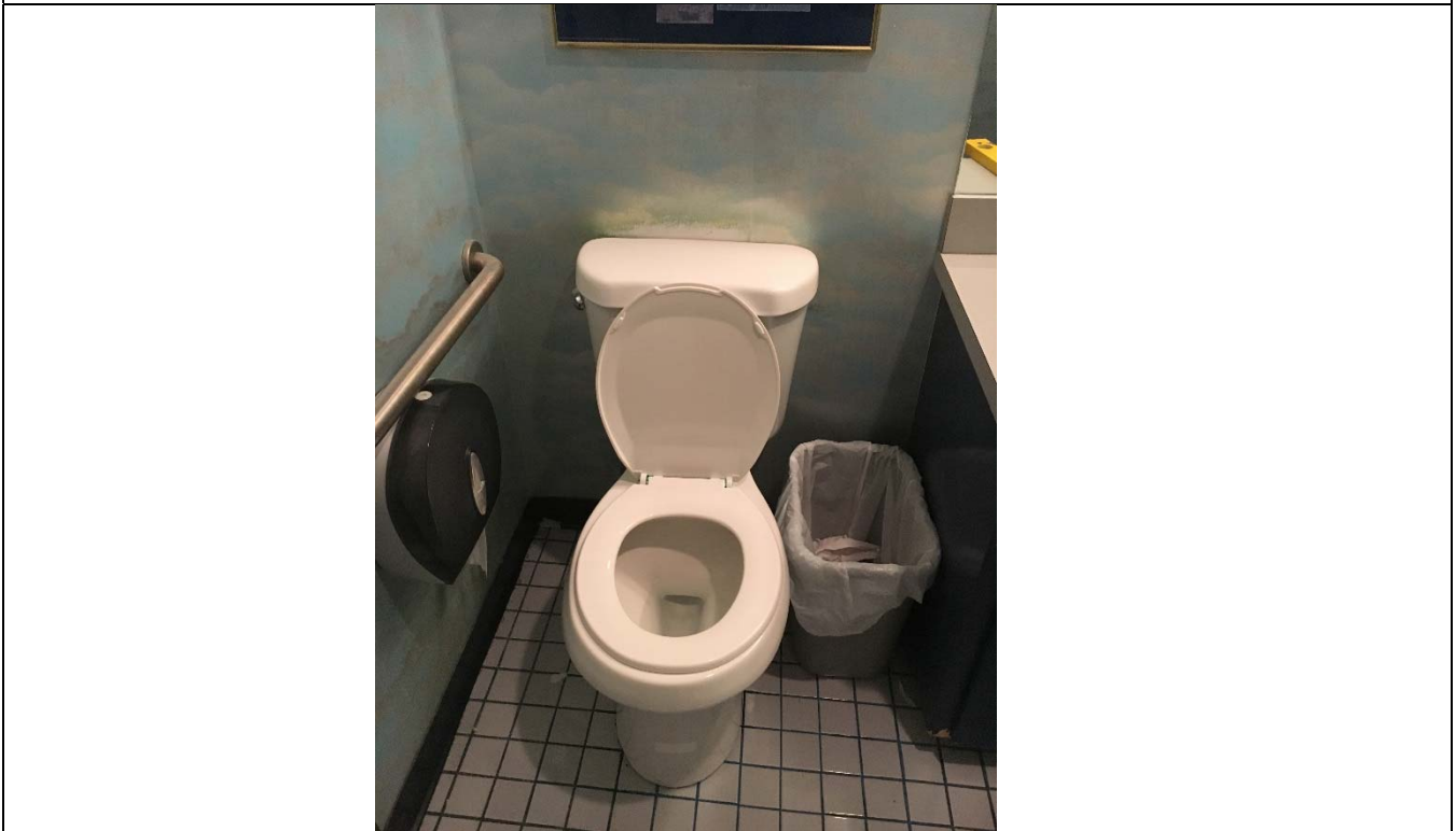
Violation 20 - Women's Room: Flush control is on the closed side of the water closet.
