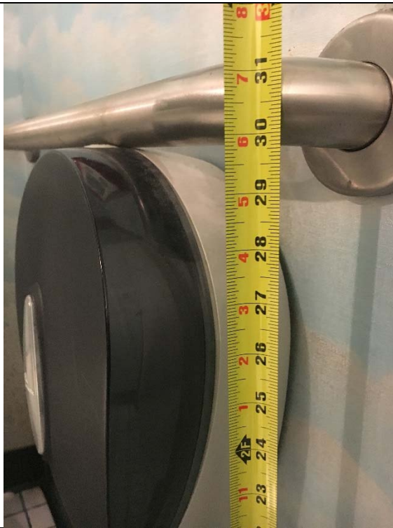
Violation 14 - Men's Room: Only a side grab bar is provided where both side and rear grab bars are required to be provided.
