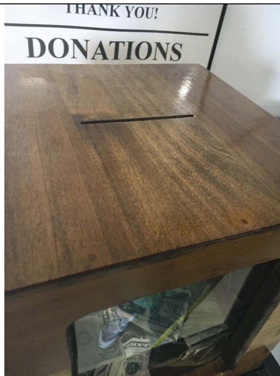
Violation 25 - The top of the donation box is at 56" above finished floor.
