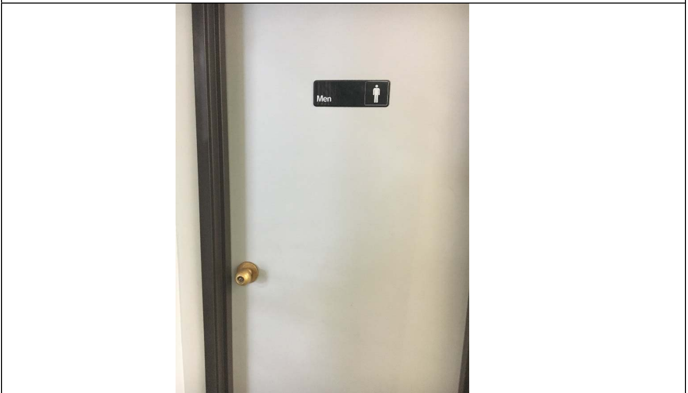
Violation 11 - Men's Room: Signage is mounted on the door and does not have Braille or tactile characters.
