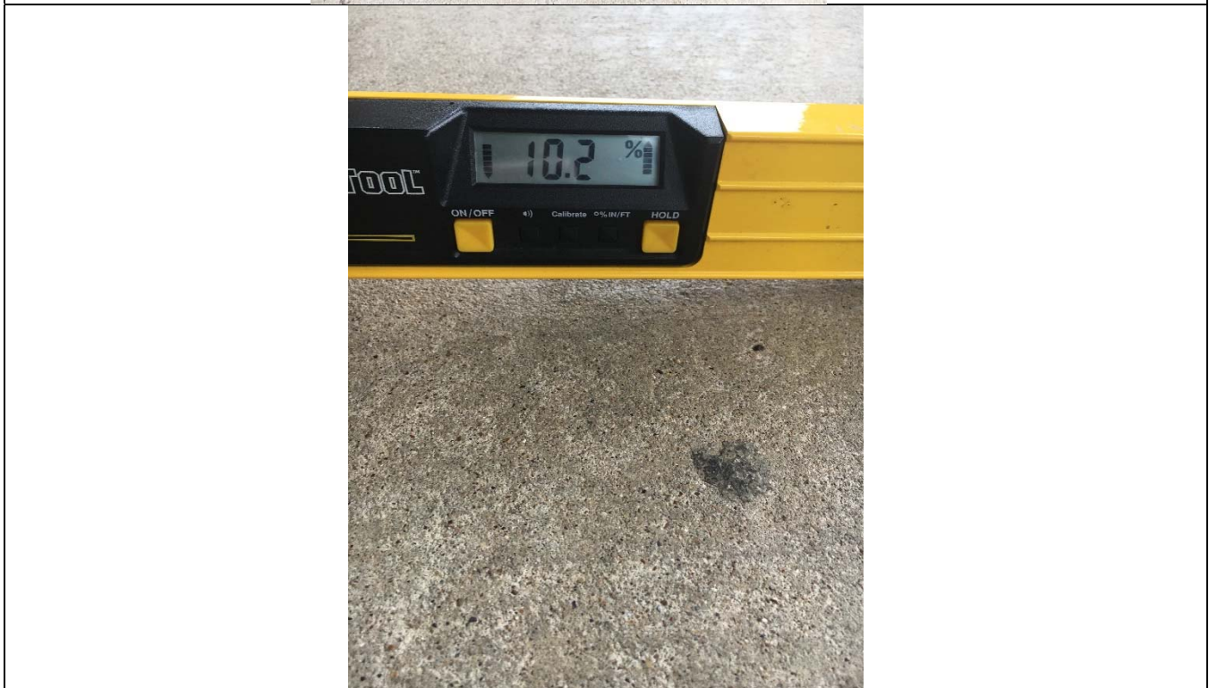
Violation 7 - There is a 10.2% slope at the main entrance door.
