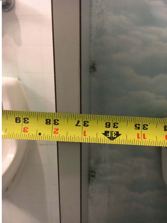
Violation 13 - Men's Room: Water closet's required clear floor width is blocked by the urinal screen and the urinal.
