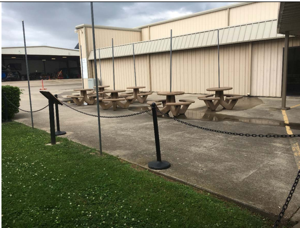
Violation 26 - There are no accessible picnic tables provided.
