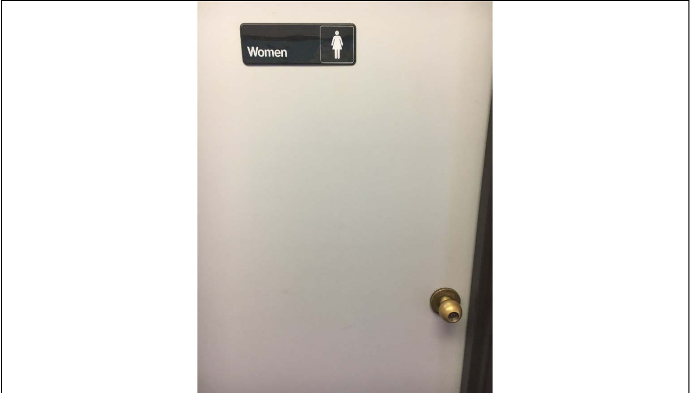
Violation 17 - Women's Room: Signage is mounted on the door.
