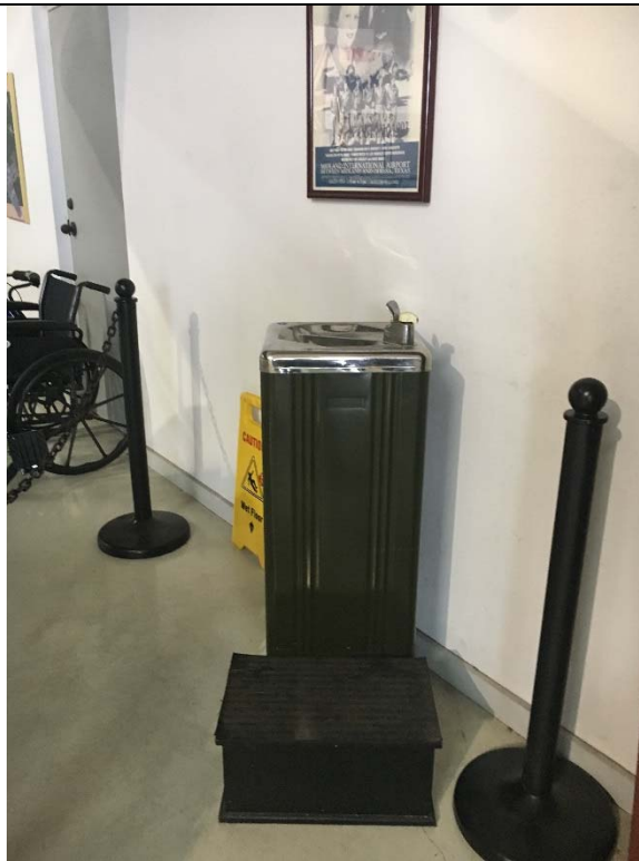
Violation 24 - There is only one drinking fountain provided in the hangar area and it is not compliant.
