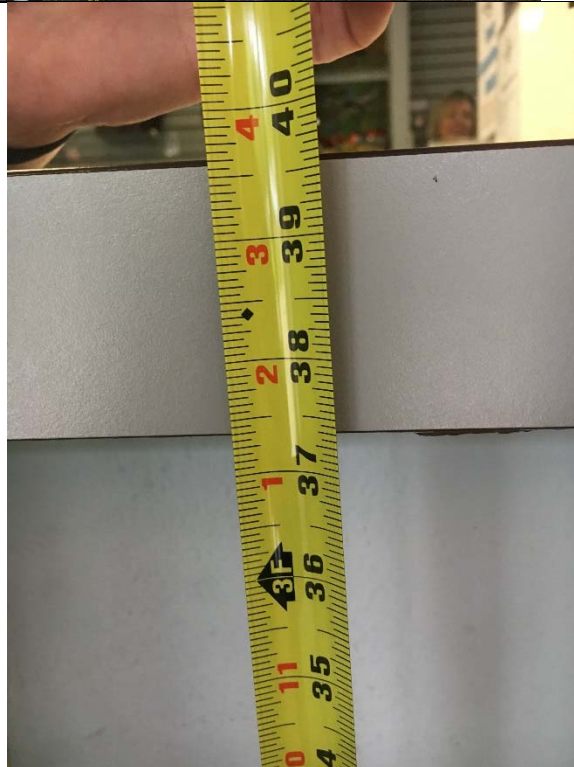
Violation 9 - The front desk is 39-9/16" to the top of the counter.
