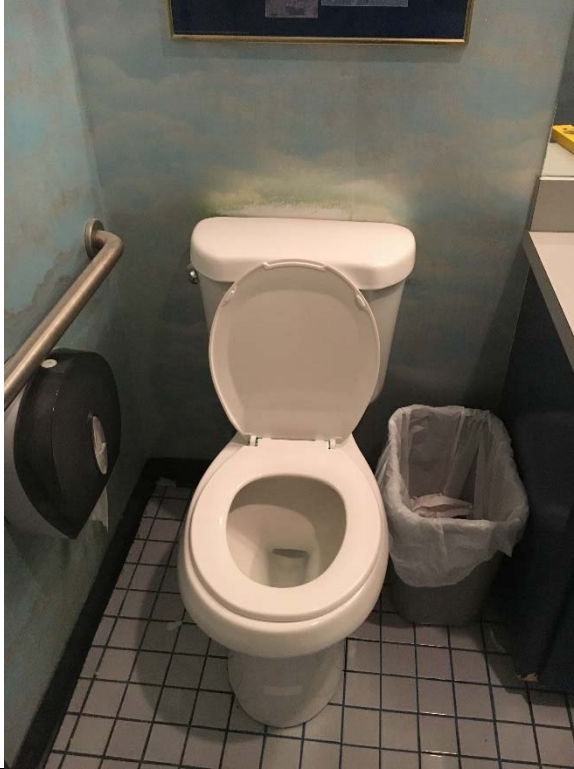
Violation 21 - Women's Room: Only a side grab bar is provided where both side and rear grab bars are required to be provided.
