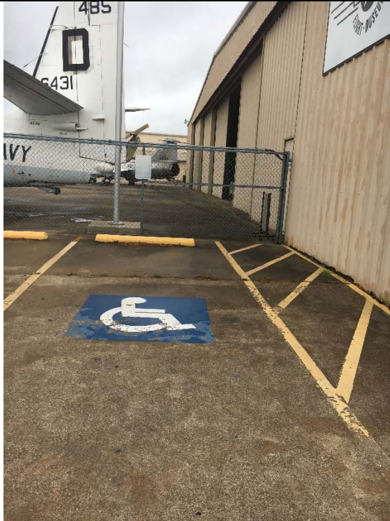
Violation 2 - The accessible parking space is required to van accessible.
