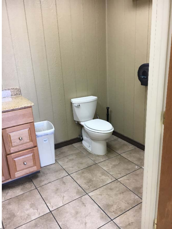
Violation 5 – There are no grab bars provided.
