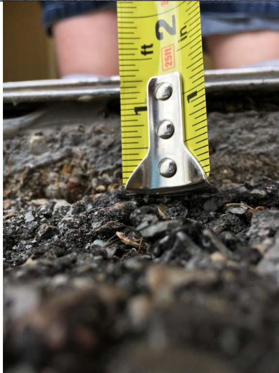
Violation 1 - There is a 1-1/4" threshold at the entrance door.
