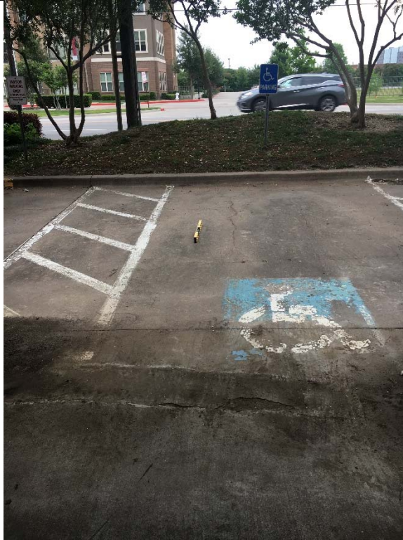
Violation 1 - The accessible parking space on the left facing the street has a running slope of 3.1%.
