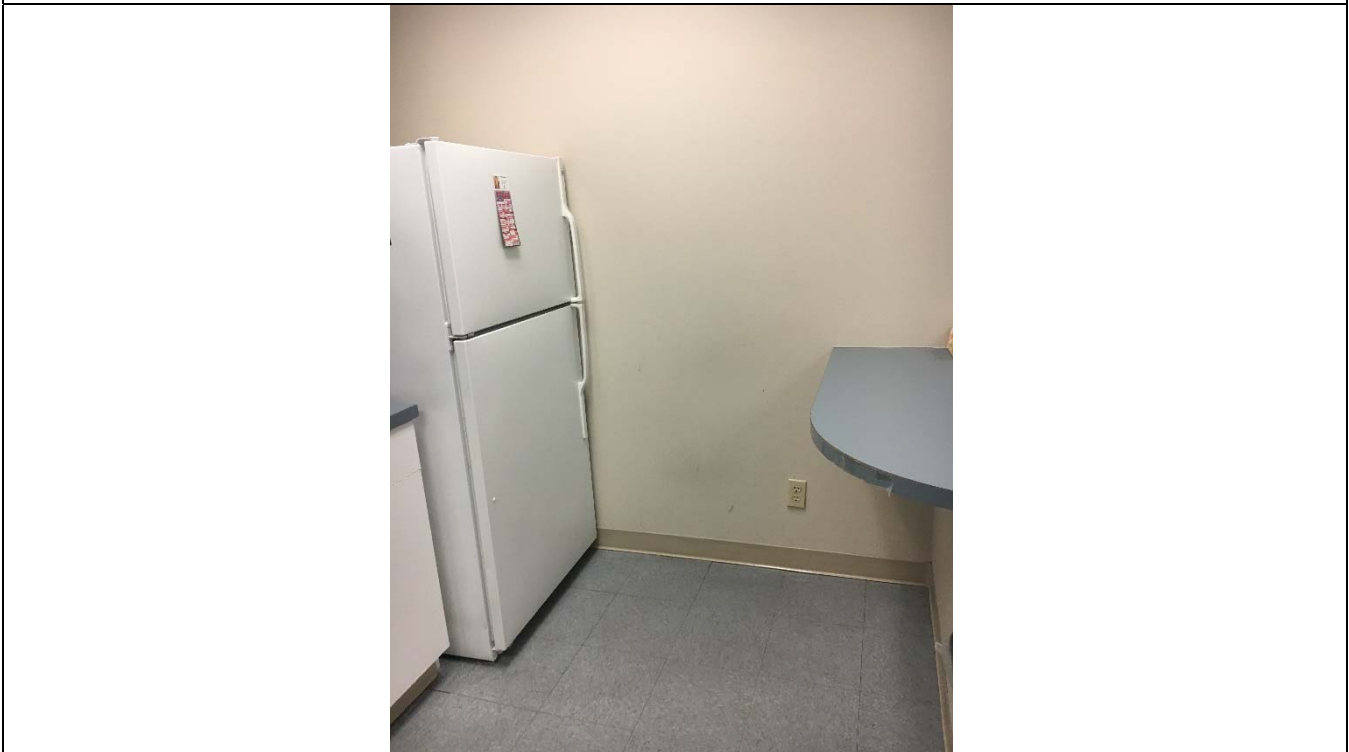
Violation 23 - The counter in front of the refrigerator reduces the required clear floor space and maneuvering clearance required for use of the refrigerator down to 38".
