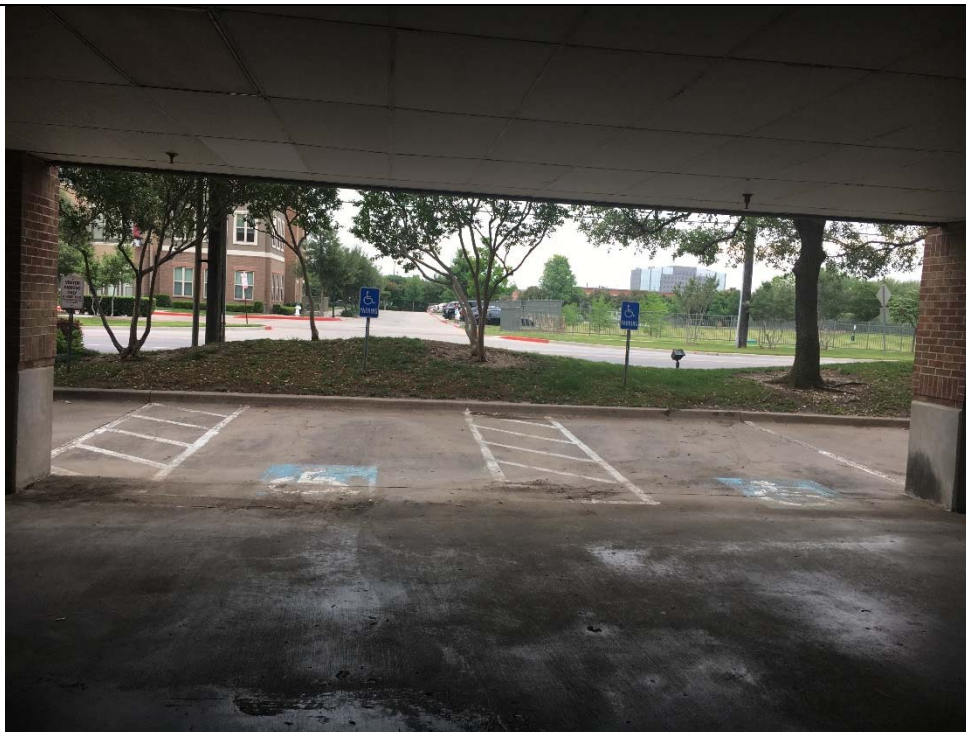
Violation 2 - The both access aisles facing the street are only 47" wide where a minimum 60" wide access aisle is required. Neither accessible parking space is wide enough to accommodate a van accessible space.
