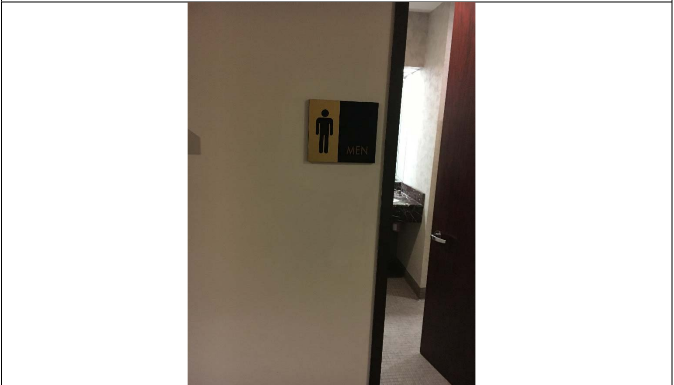
Violation 17 - Men's Restroom - Entry door requires more than 5lbs to open.
