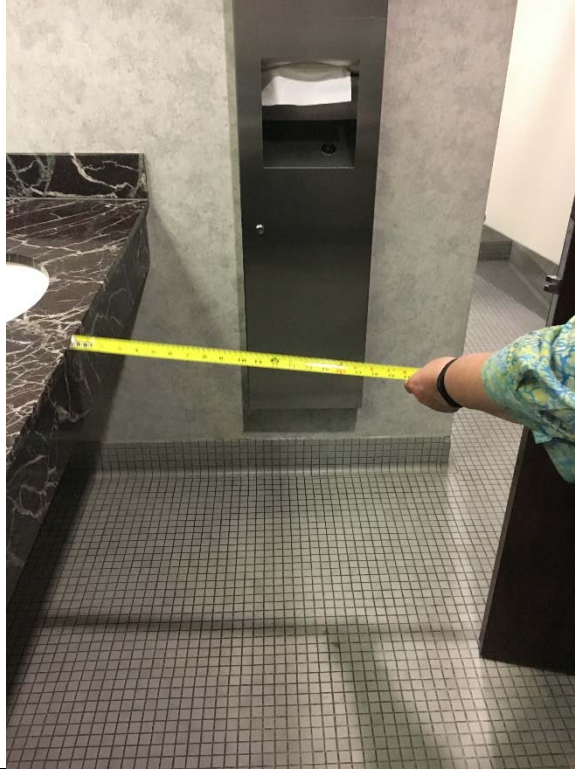
Violation 13 – Women's Restroom - The distance between the door and the lavatory is only 29". A minimum of 48" maneuvering clearance is required.
