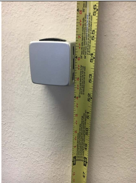
Violation 9 - The thermostat control in the hallway is mounted with the highest operable part at 54-5/8" above finished floor where 48" high maximum is required.
