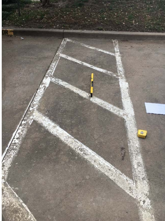
Violation 3 - The left access aisle facing the street has a running slope of 2.3%.
