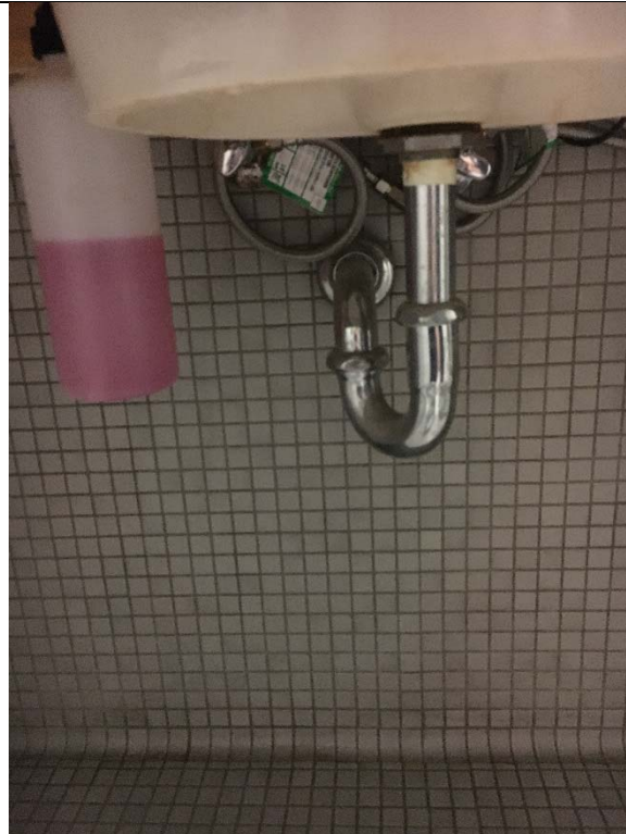
Violation 14 - Women's Restroom - Pipes under the lavatory are not wrapped.
