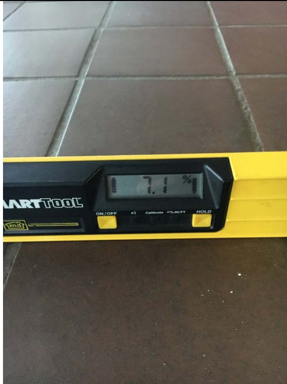
Violation 8 - The landing at the main entrance to the building has a running slope of 7.1%.
