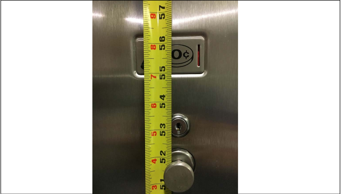
Violation 16 - Women's Restroom - The feminine product dispenser is mounted with the highest operable part at 55-1/2" above finished floor and requires grasping to operate.
