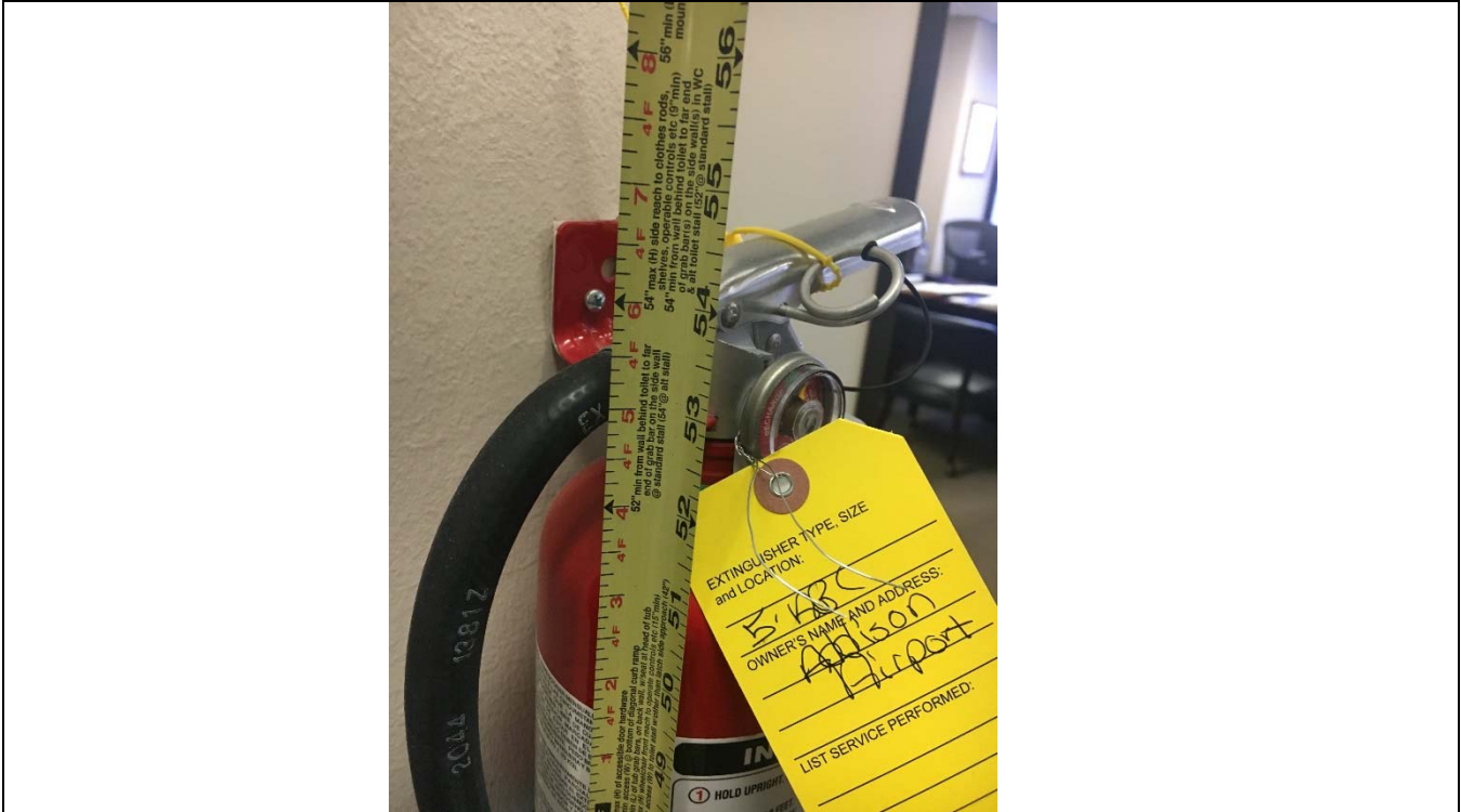
Violation 10 - The fire extinguisher provided in the hallway is mounted with the highest operable part at 54" above finished floor where 48" high maximum is allowed.
