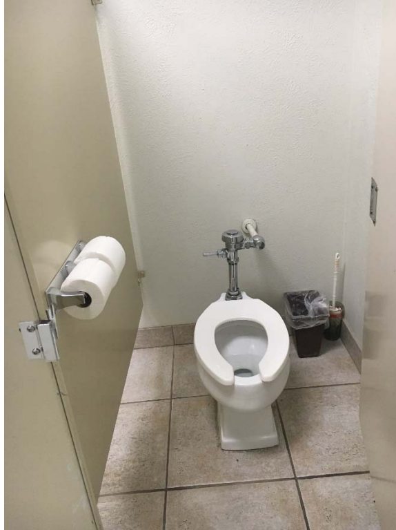
Violation 24 - Women's Restroom first floor of 4310 - Does not have an accessible stall provided.
