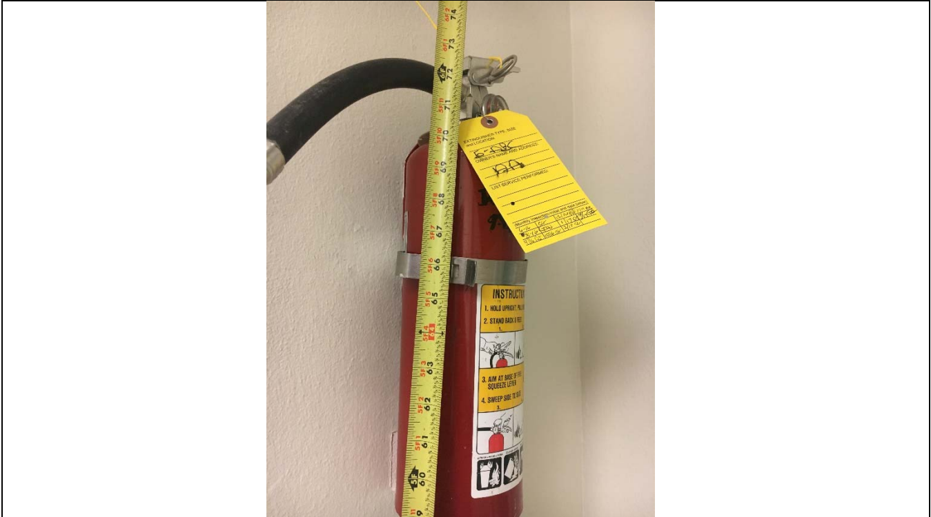
Violation 12 - The Fire extinguishers throughout the facility are mounted where the highest operable part is between 63-1/2"-72" above finished floor.
