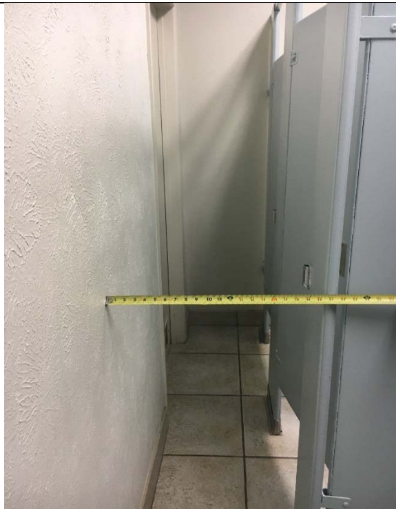
Violation 29 - Men's Restroom first floor on 4310 - The path leading to the stalls is only 20-1/2" wide.
