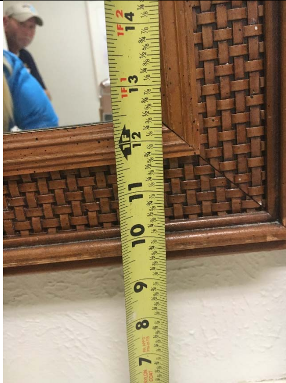
Violation 26 - Women's Restroom first floor of 4310 - The mirror is mounted at 43" above finished floor.
