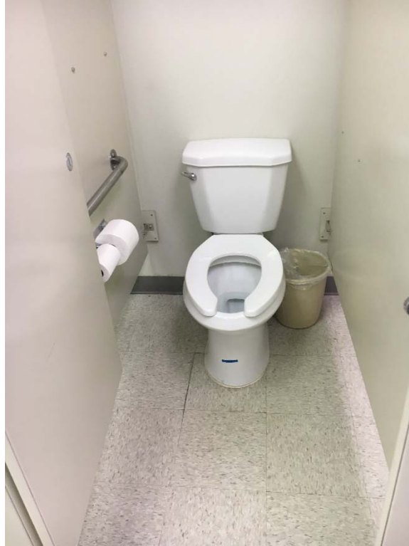
Violation 34 - Women's Restroom second floor of 4310 - Does not have an accessible stall provided.
