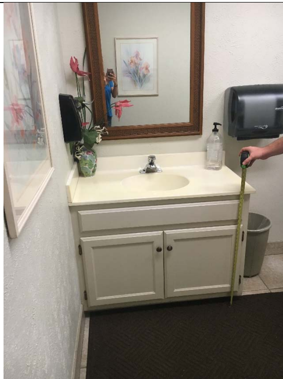
Violation 25 - Women's Restroom first floor of 4310 - There is a cabinet beneath the lavatory blocking the required knee clearance.
