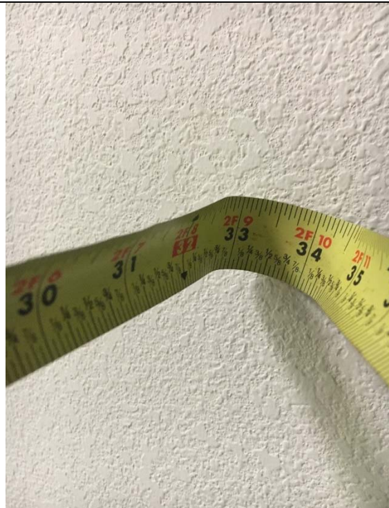
Violation 38 - Men's Restroom second floor of 4310 - The opening leading into the restroom is only 33-1/2" wide.
