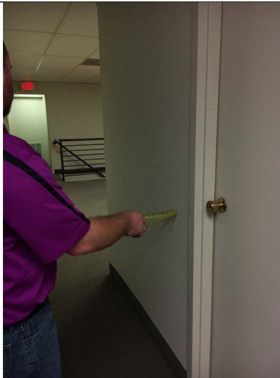
Violation 48 - The hallway leading into the breakroom is only 33" wide.
