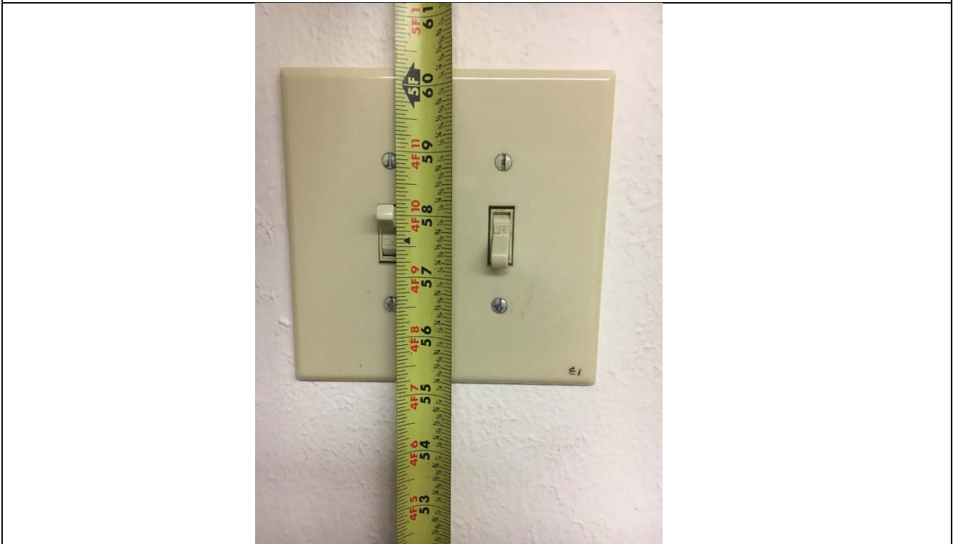
Violation 13 - Light switches from 49"-58"aff to the highest operable part.
