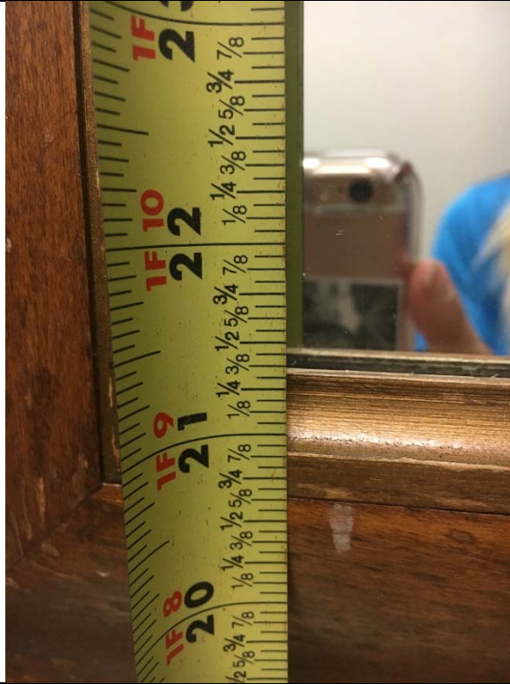
Violation 32 - Men's Restroom first floor of 4310 - The mirror is mounted at 53" above finished floor.
