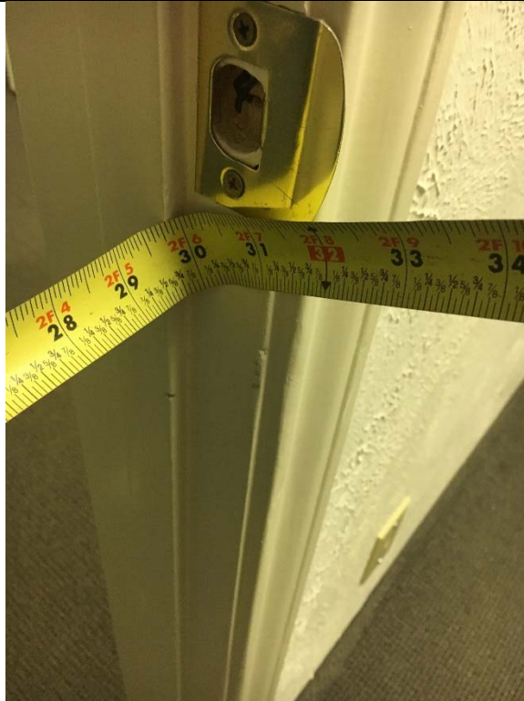
Violation 19 - There are 2 office doors on the 2nd floor that have openings that are less than the required 32" minimum wide.
