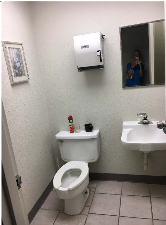
Violation 44 - Women's Restroom first floor of 4308 - Toilet room is not large enough to accommodate a wheelchair turning space.
