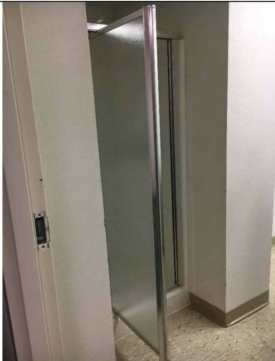
Violation 42 - There is a shower provided in the shower room on the 4310 side on the 2nd floor that has no compliant features.
