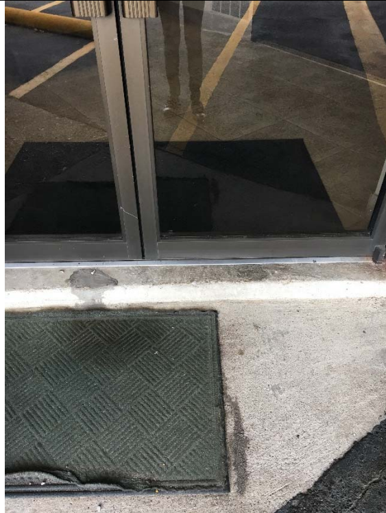
Violation 5 - There is a level change as well as an unsecured mat at the entrance to 4308.
