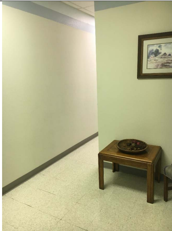
Violation 33 - Women's Restroom second floor of 4310 - The opening leading into the restroom is only 30" wide.
