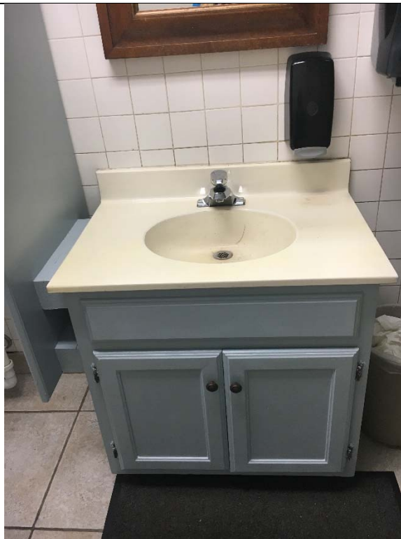
Violation 31 - Men's Restroom first floor of 4310 - There is a cabinet beneath the lavatory blocking the required knee clearance.
