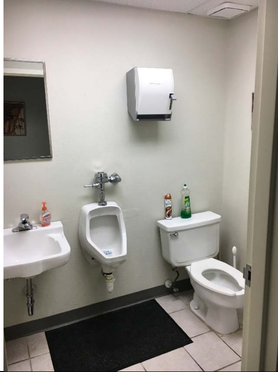
Violation 43 - Men's Restroom first floor of 4308 - Toilet room is not large enough to accommodate a wheelchair turning space.
