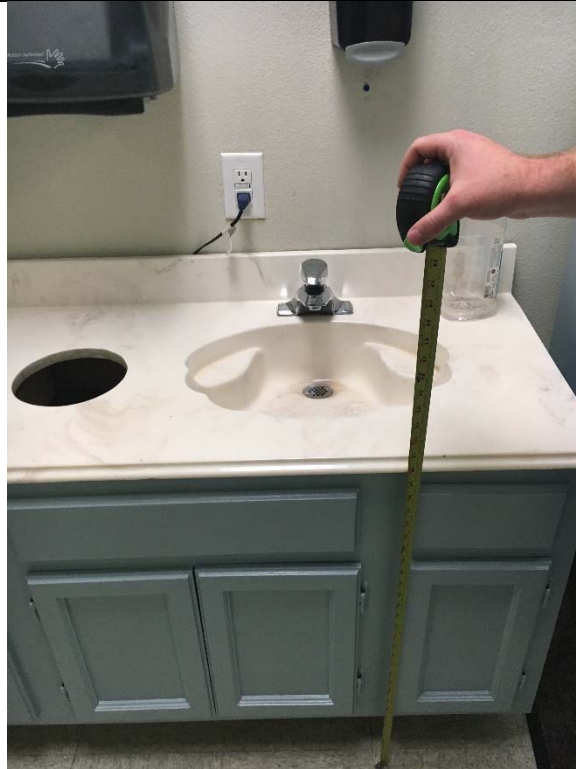
Violation 41 - Men's Restroom second floor of 4310 - There is a cabinet beneath the lavatory blocking the required knee clearance.
