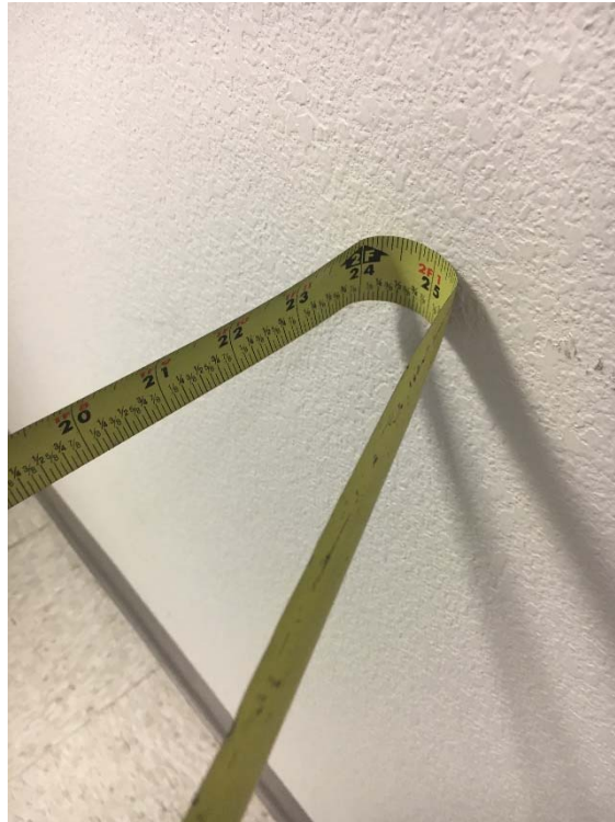
Violation 39 - Men's Restroom second floor of 4310 - The path leading to the stalls is only 25" wide between the stalls and the wall.
