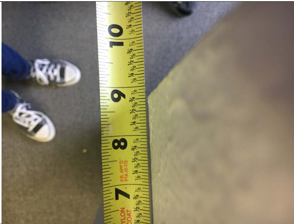
Violation 20 - There is one office door on the 2nd floor that does not have the minimum 18" maneuvering clearance on the pull side.
