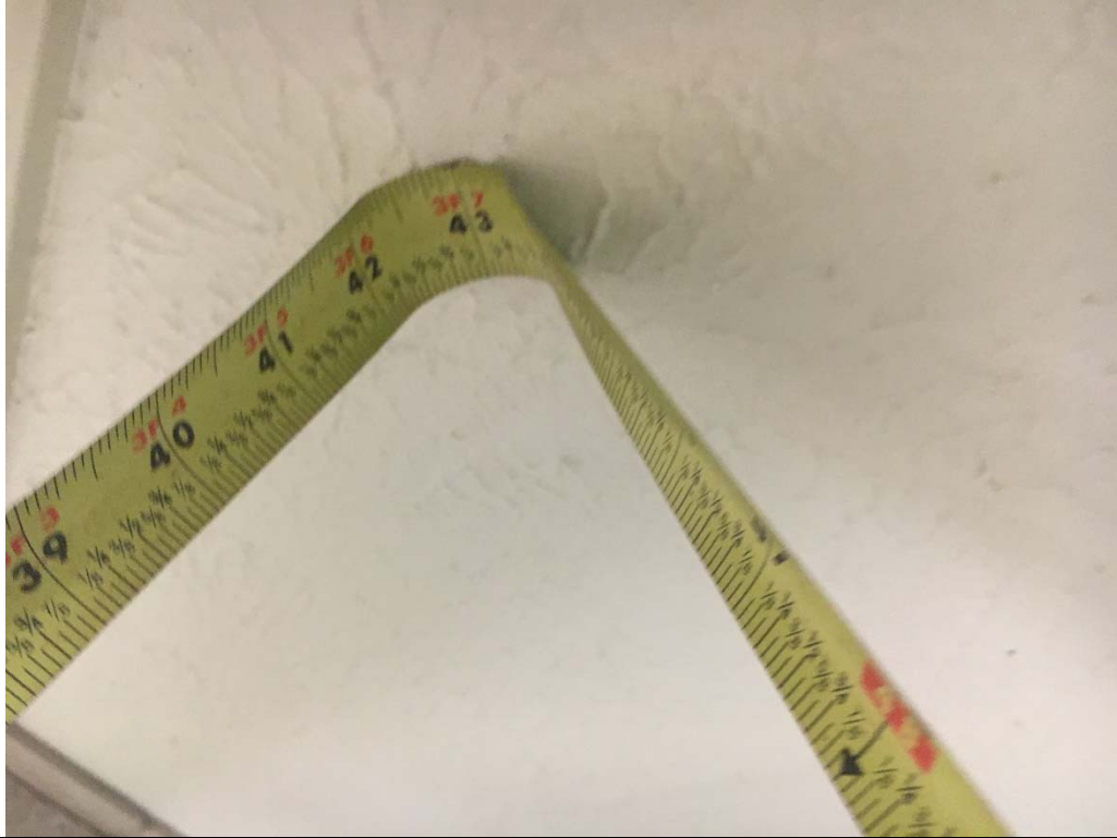
Violation 28 - Men's Restroom first floor of 4310 - Entrance door maneuvering clearance is only 43" deep on the pull side where a 48" deep maneuvering clearance is required.
