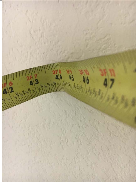
Violation 37 - Men's Restroom second floor of 4310 - The maneuvering clearance on pull side of the door is only 44" deep.
