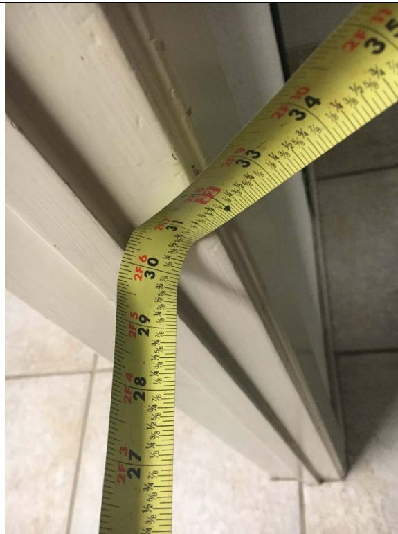
Violation 27 - Men's Restroom first floor of 4310 - Entrance door is only 31" wide.
