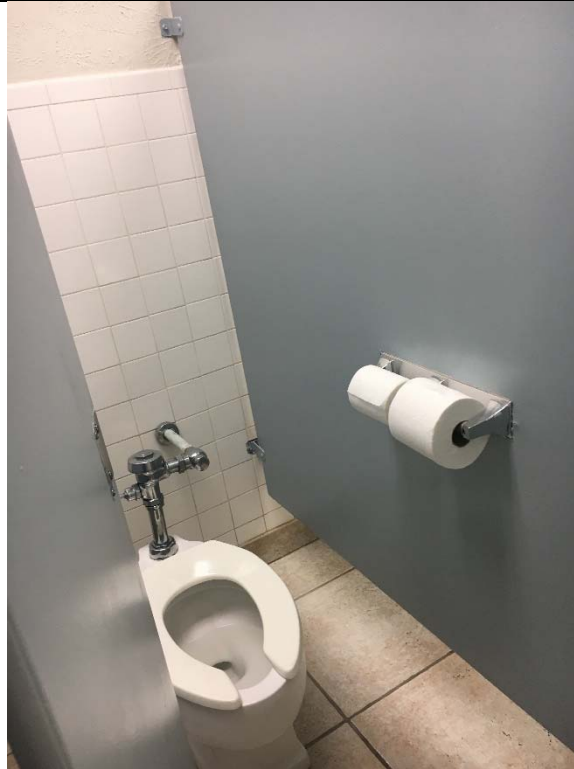
Violation 30 - Men's Restroom first floor of 4310 - Does not have an accessible stall provided.
