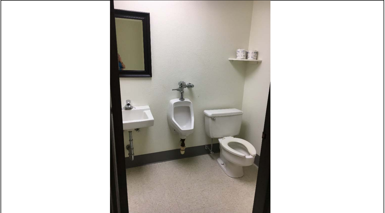
Violation 45 - Men's Restroom second floor of 4308 - Toilet room is not large enough to accommodate a wheelchair turning space.
