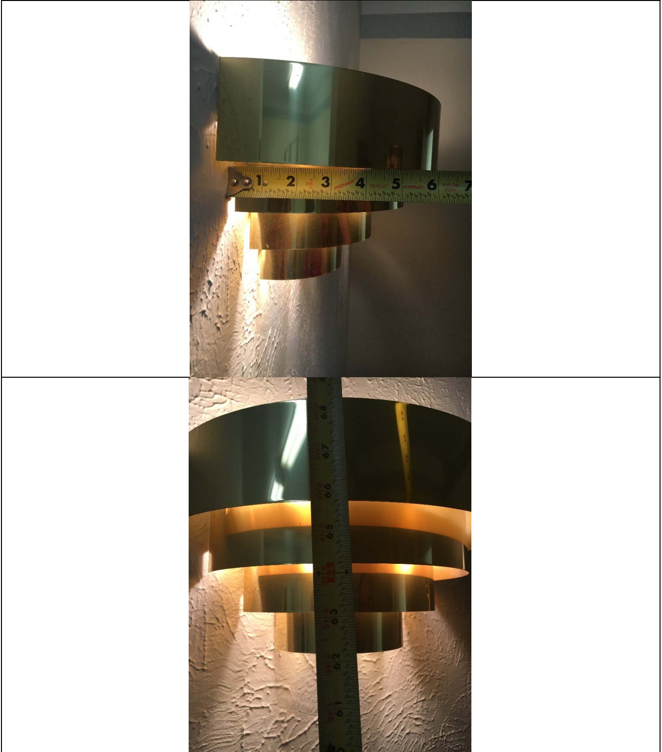
Violation 15 - There is a light fixture in the hallway that protrudes 6" into the path of travel at 62-3/16" above finished floor.
