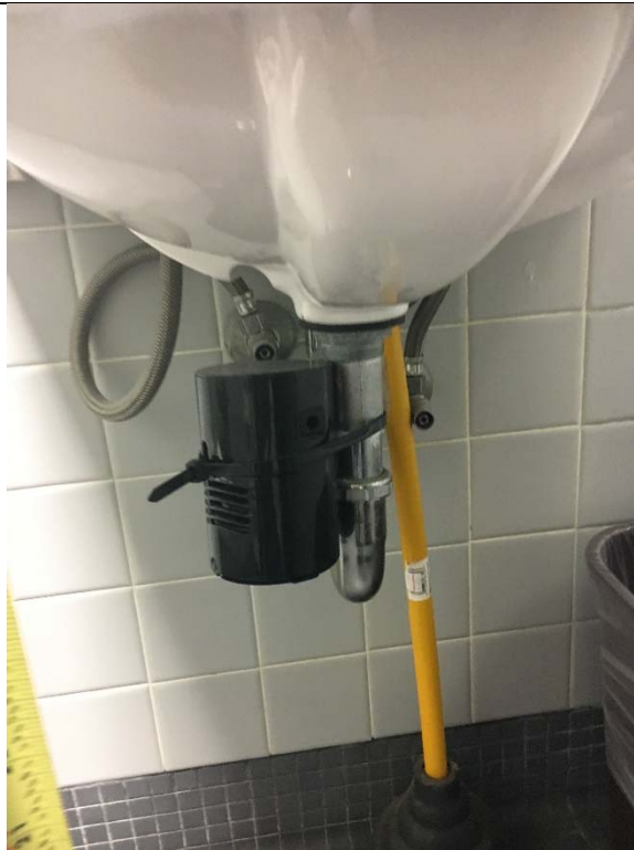
Violation 23 - Single user restroom on the 2nd floor - The lavatory pipes are not wrapped.
