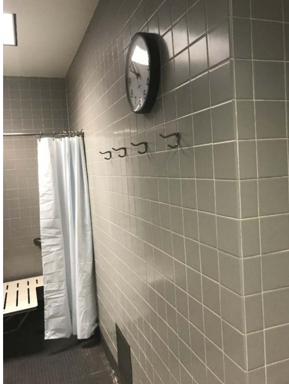
Violation 40 - Men's Locker Room - Coat hooks are mounted at 68" to the highest operable part, 48" maximum is required.
