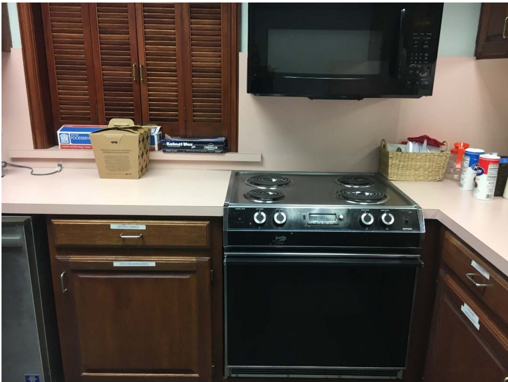
Violation 48 - The microwave in the 2nd floor break room is mounted over the stove and out of the required reach range.
