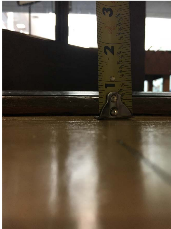
Violation 50 - There is an 11/16" change in level to enter the gymnasium.
