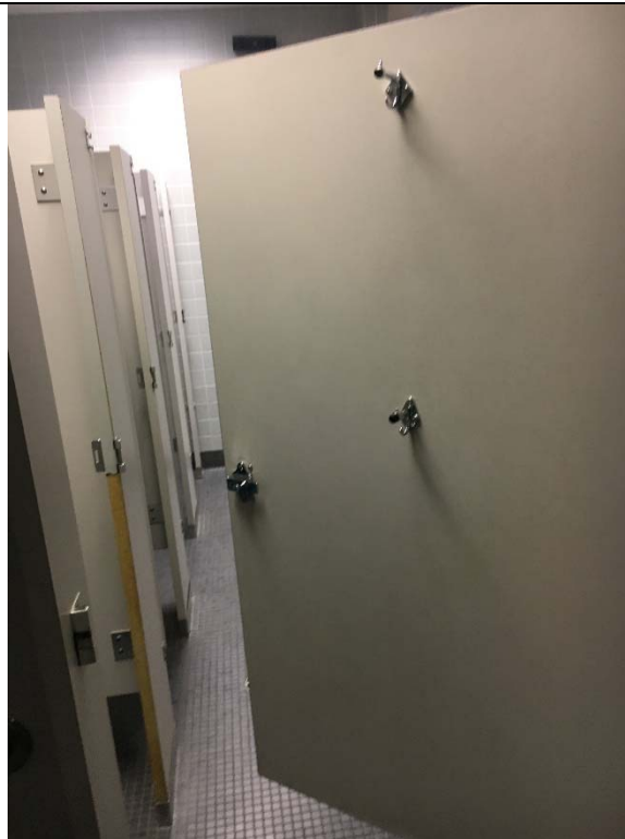
Violation 35 - Women's Locker Room - Accessible toilet compartment door is not self-closing.
