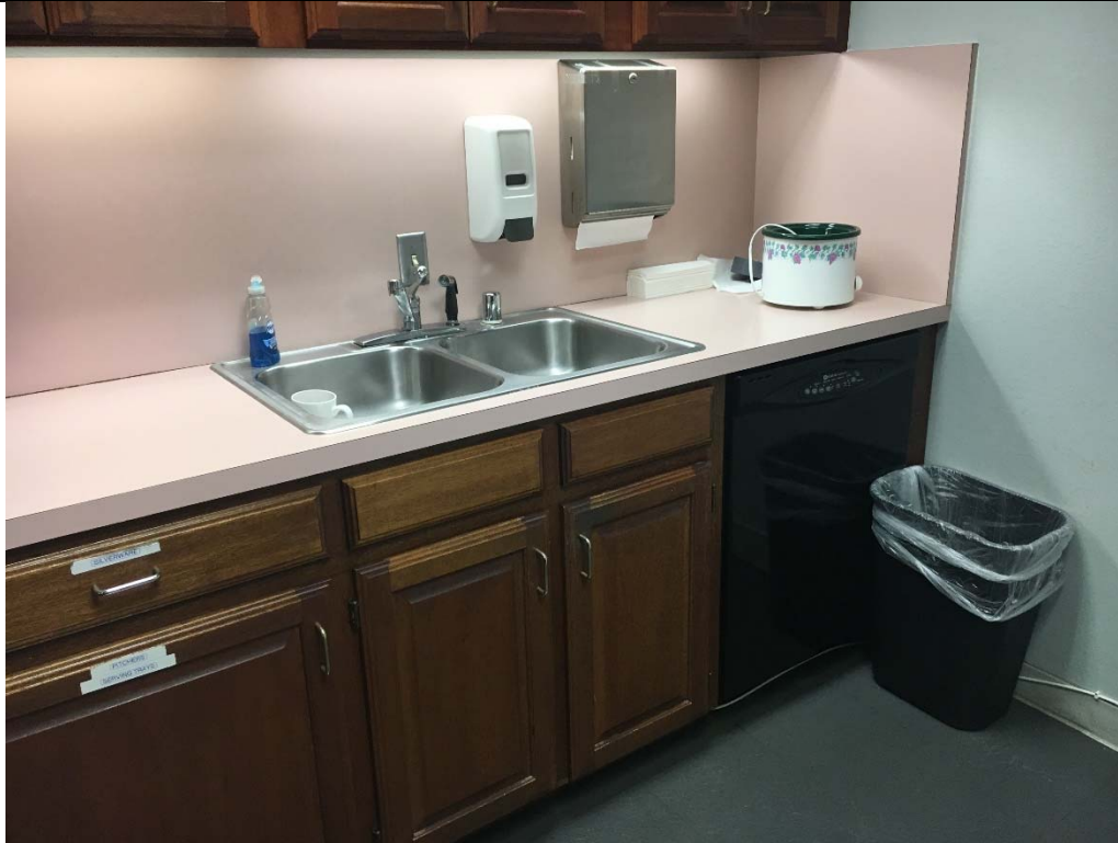
Violation 47 - The sink in the 2nd floor break room is at 36 1/4" with no knee clearance provided.
