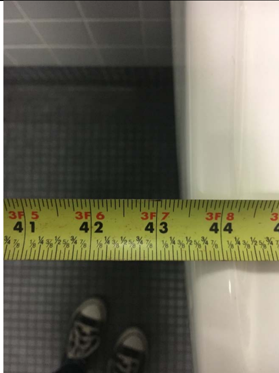
Violation 22 - Single user restroom on 2nd floor - The lavatory encroaches into the required clear floor width of the water closet.
