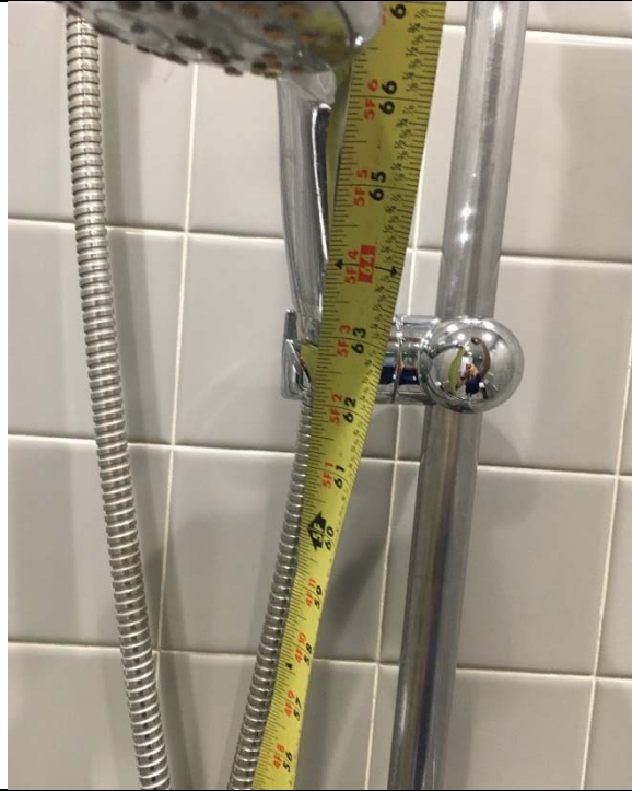
Violation 32 - Women's Locker Room - The shower head is mounted at 63" where a maximum of 48" is required.
