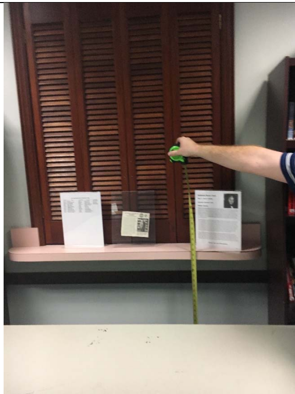
Violation 51 - The counter in the conference room is at 39-3/4", where a maximum of 36" is required.
