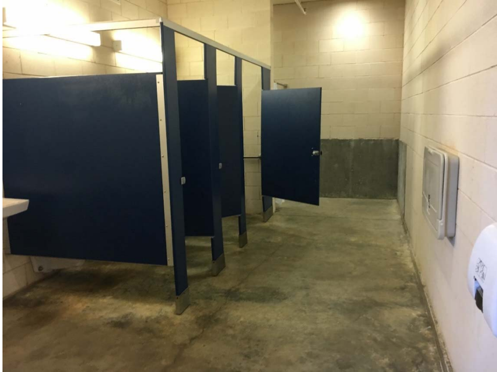
Violation 43 - Men's and Women's restrooms in the exterior pool area - Accessible stall doors are not self-closing.
