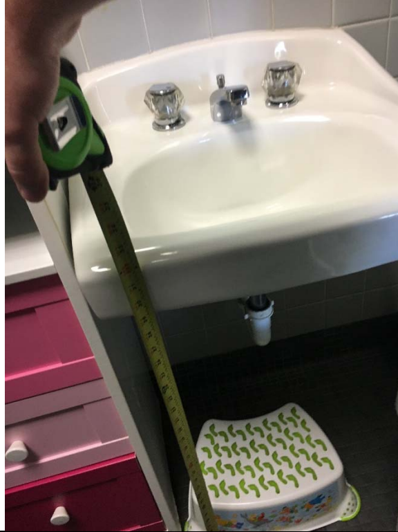
Violation 17 - The lavatory in the child care restroom lavatory pipes are not protected.
