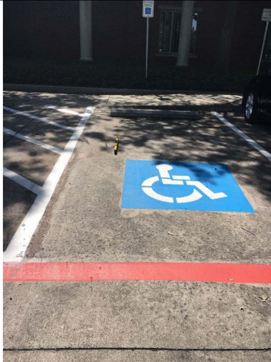
Violation 1 - The far right accessible parking space in the front lot (closest to the main door) has a running slope of 3.2%.
