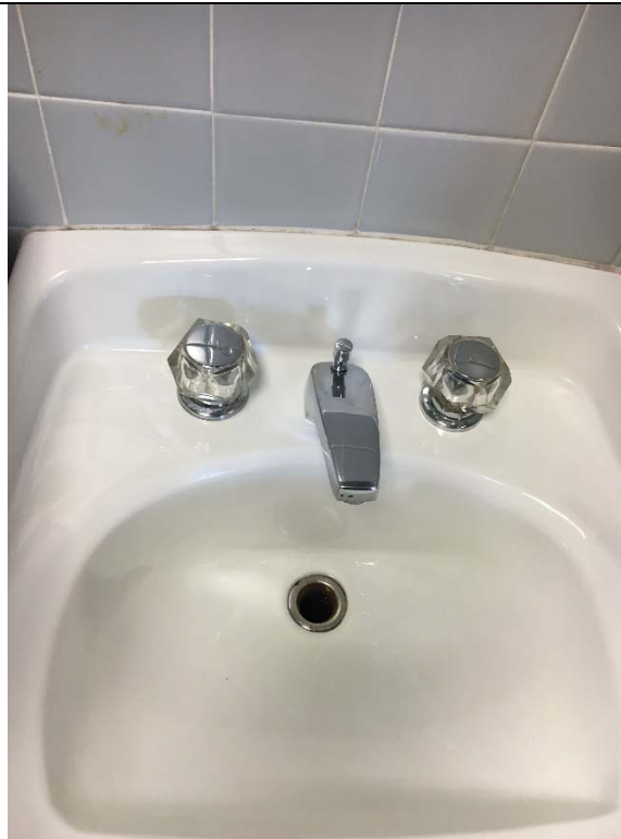
Violation 18 - The lavatory in the child care restroom lavatory has knob style handles requiring grasping and twisting to operate.
