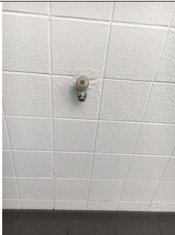
Violation 62 - The control for the hose in the indoor pool area requires tight grasping and twisting to operate.
