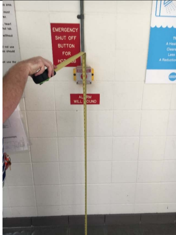
Violation 61 - The emergency shut off bottom at the indoor pool is mounted at 50", where a maximum of 48" is required.
