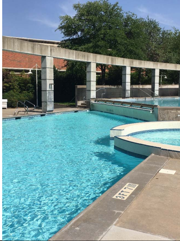
Violation 57 - There is no accessible means of entry into the exterior pool.
