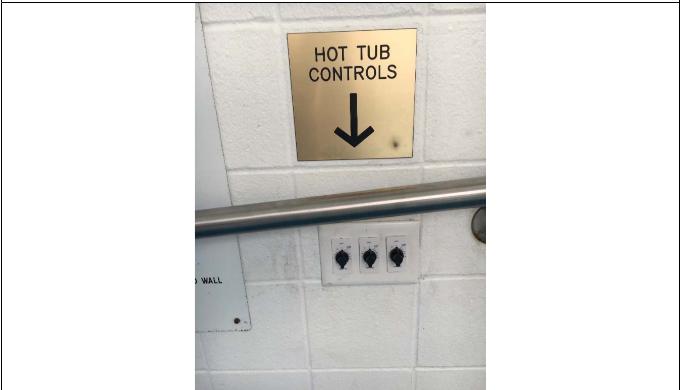
Violation 60 - The controls for the hot tub located at the indoor pool area are located on the ramp and not served by a level clear floor space.
