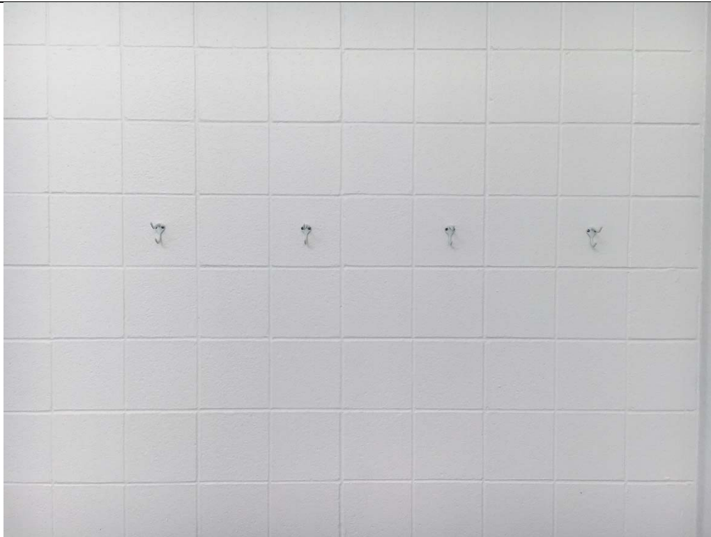
Violation 58 - Coat hooks provided at the indoor pool area are at 61" where a maximum of 48" is required.
