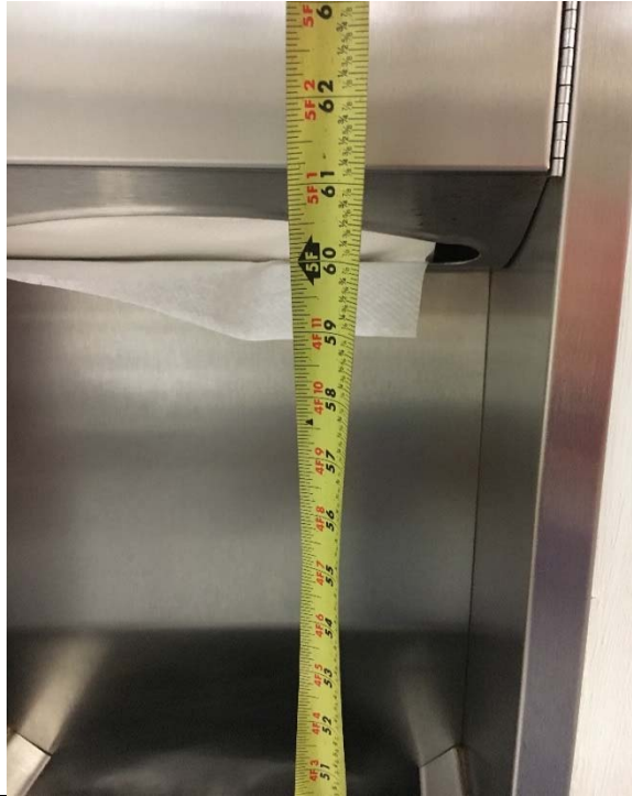
Violation 34 - Women's Locker Room - Paper towel dispenser's operable part is at 60" where a maximum of 48" is required.
