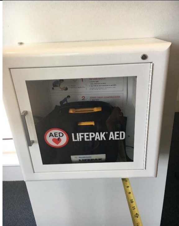
Violation 15 - The Lifepak AED case located in the 2nd floor exercise room protrudes into the path of travel 7" at 27".
