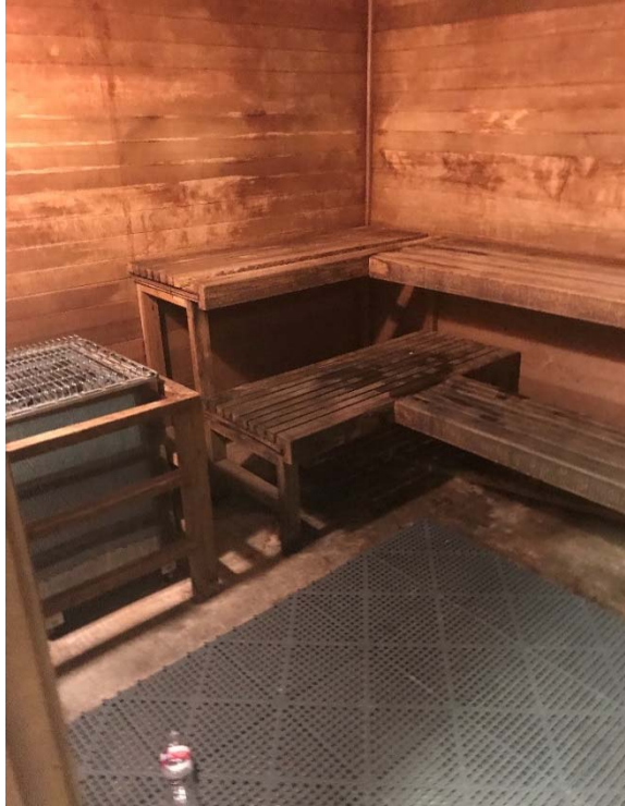
Violation 38 - Men's Locker Room - The sauna and steam rooms do not have accessible benches provided.
