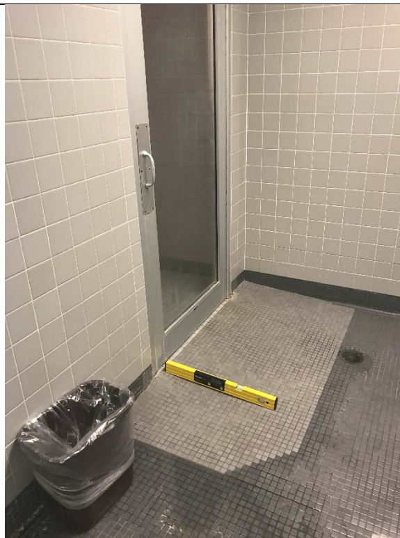
Violation 37 - Men's Locker Room - There is a 5.7% slope leading into the sauna, there is no level landing provided.
