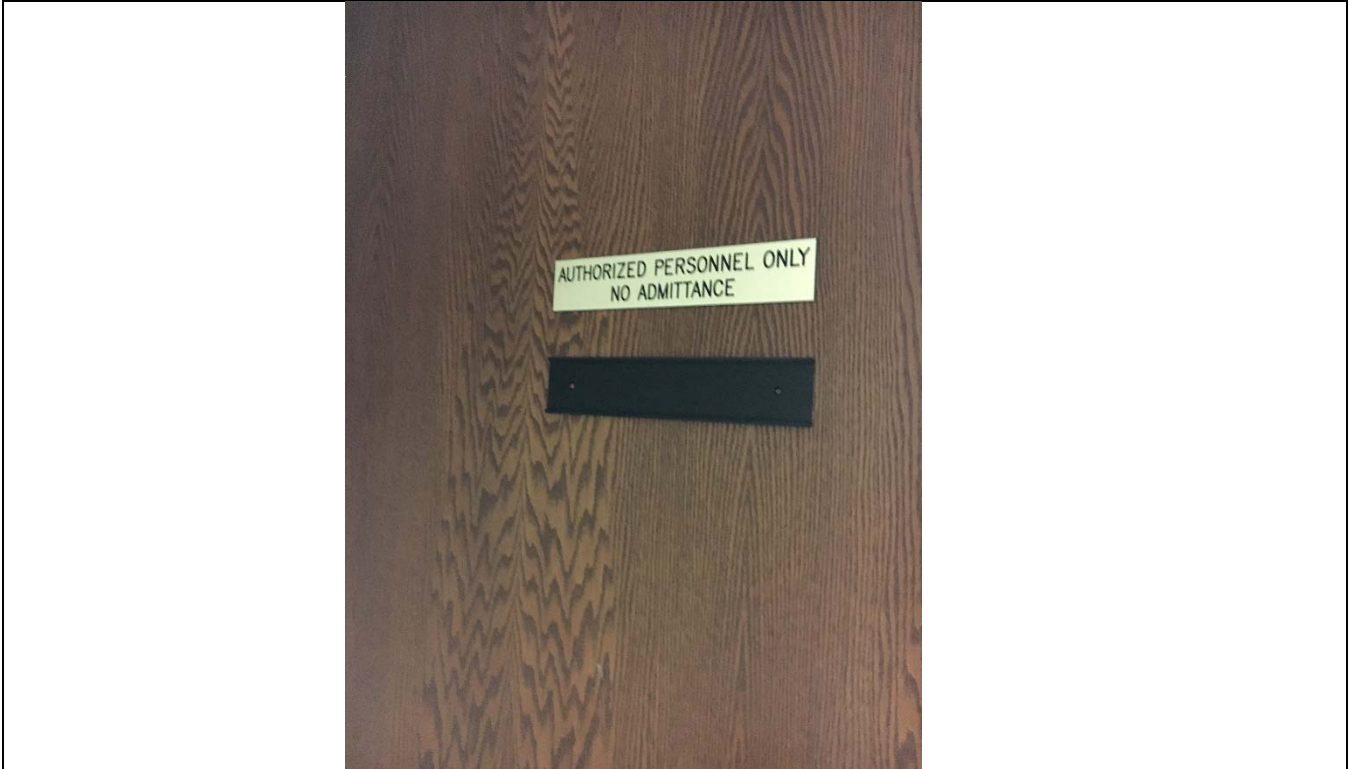
Violation 13 - Signage is mounted on the door and is not compliant.
