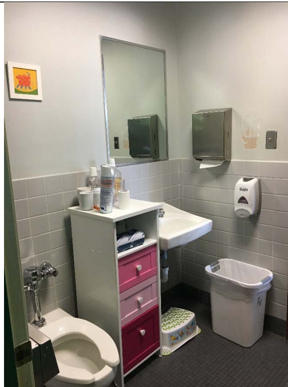
Violation 16 - The water closet in the child care restroom does not have the required clear floor space provided. Additionally, the flush control is on the closed side.
