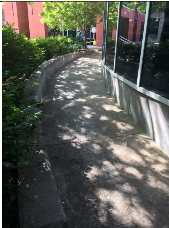
Violation 2 - The ramp leading to the exterior upper pool area and the exterior restrooms has a 5.4% running slope with no handrails.
