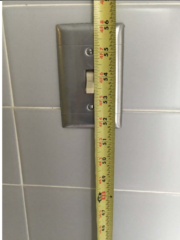
Violation 36 - Women's Locker Room - Light switch is mounted at 54".
