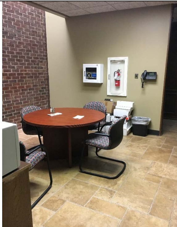
Violation 29 - The phone in the break room is a protruding object and is mounted with the highest operable part above 48".
