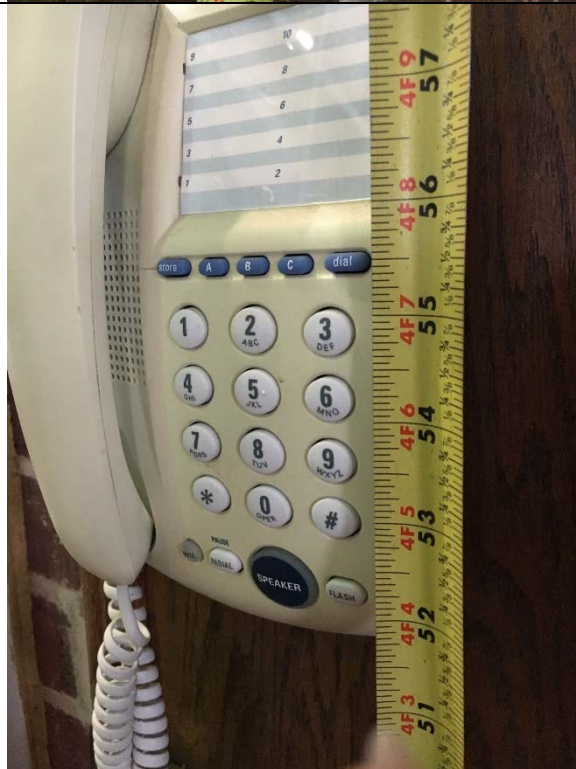
Violation 6 - The assistance phone (55.5") and push button (49") provided in the entrance vestibule are mounted above the 48" maximum reach range requirement.
