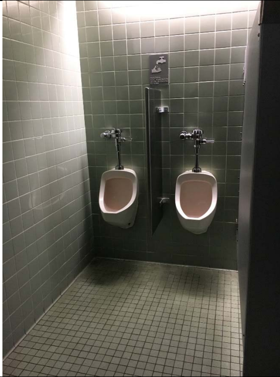
Violation 25 - Men's shower room does not have any accessible urinals.
