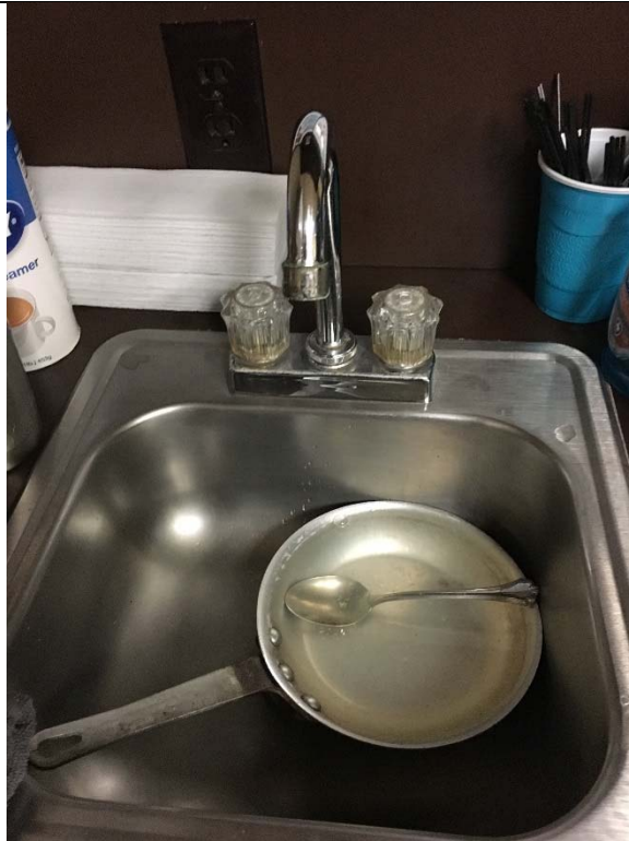
Violation 31 - The break room sink controls require grasping and twisting to operate.
