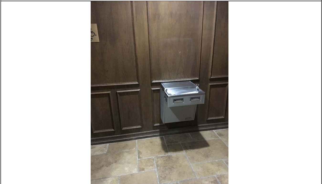
Violation 36 - Outside the restrooms, there is only one drinking fountain provided, two are required.
