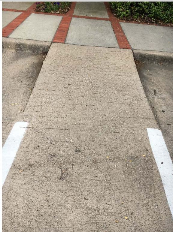
Violation 2 - There is a built up curb ramp protruding into the access aisle at the front of the building.
