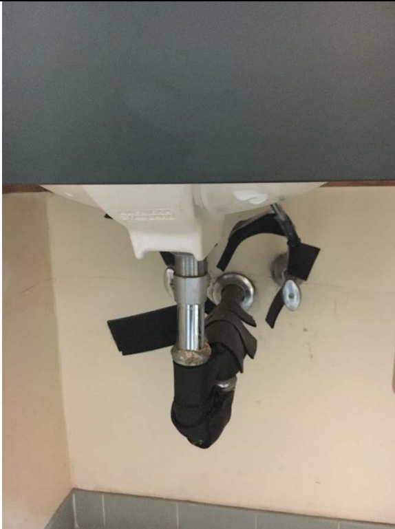
Violation 23 - Men's & Women's restrooms lavatory pipes are not protected from contact.
