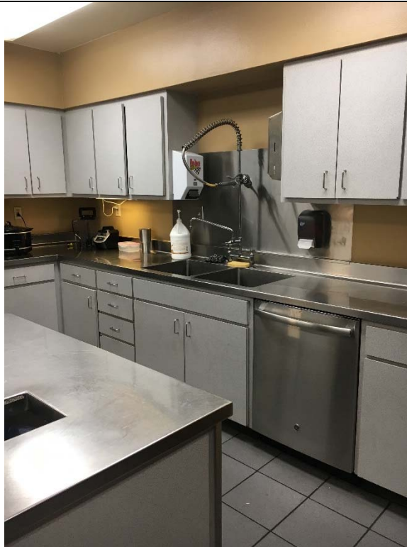
Violation 33 - The sink in the kitchen is not complaint. It has no knee clearance and is at 35 3/4".
