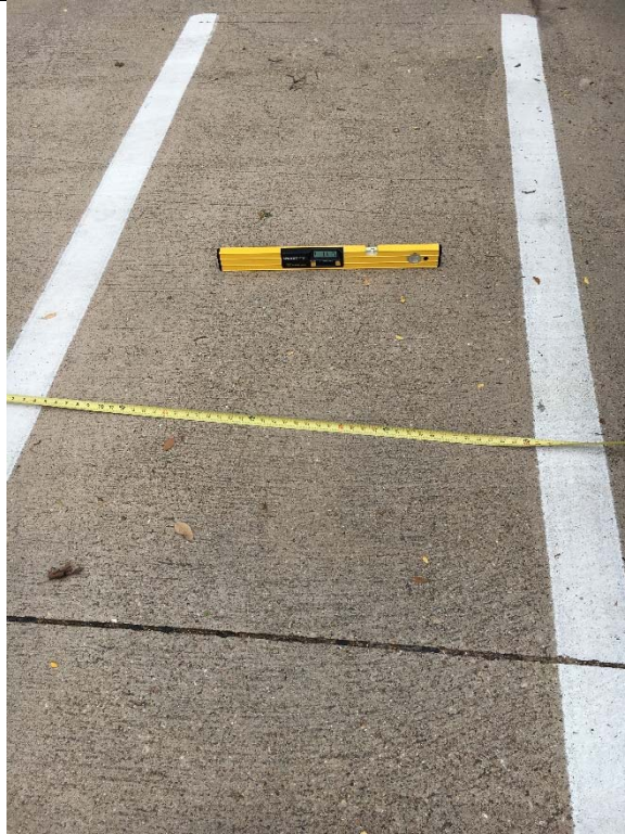
Violation 1 - The access aisle serving the front accessible parking space is only 52" wide.
