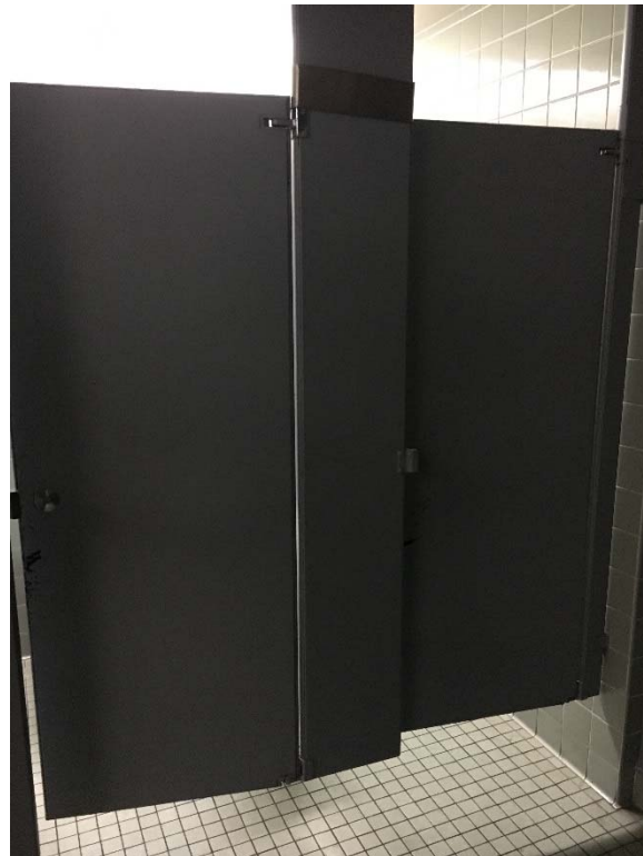
Violation 24 - Men's shower room does not have an accessible toilet compartment.
