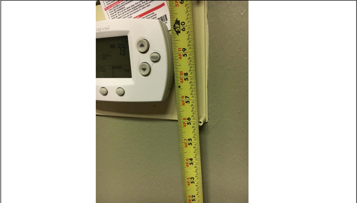
Violation 35 - The thermostat is mounted with the highest operable part at 59.5" where a maximum reach range is 48".
