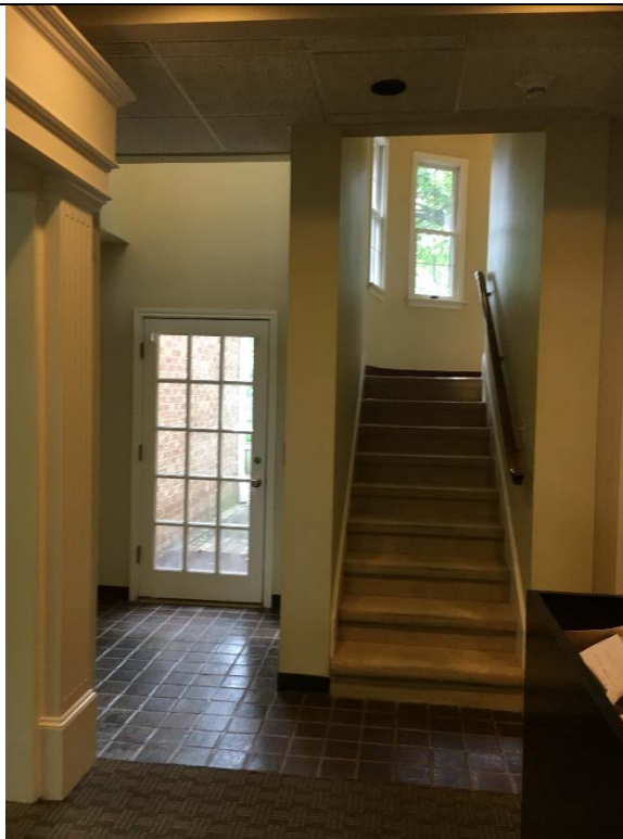
Violation 4 - There is no elevator serving this building, therefore there is no access to the 2nd floor.
