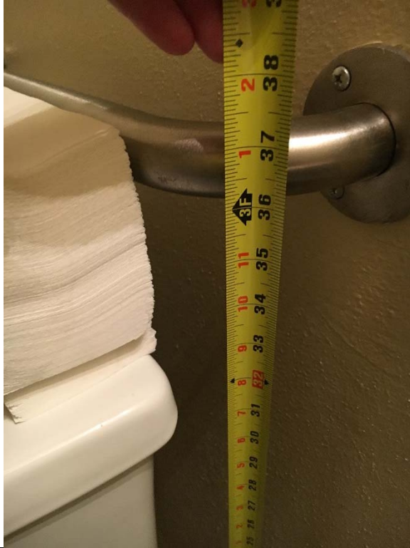
Violation 20 - Men's Restroom: The rear grab bar is mounted too high at 37" above finished floor.
