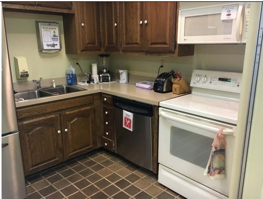
Violation 23 - The microwave is mounted above 48" to the highest operable part.
