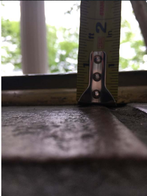
Violation 6 - The threshold at the entrance door is greater than 1/2".
