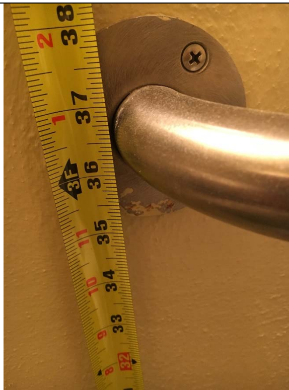
Violation 15 - Women's Restroom: The rear grab bar is mounted too high at 37" above finished floor.
