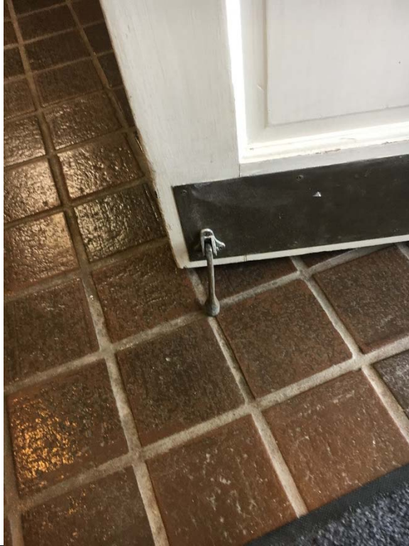
Violation 7 - The entrance door has a door stop at the bottom, therefore, the bottom 10" of the door does not have a smooth surface.
