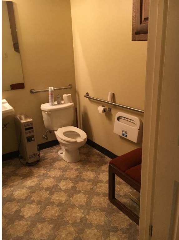
Violation 14 - Women's Restroom: The rear grab bar is only 24" long.
