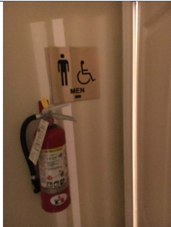
Violation 17 - Men's Restroom: Signage is mounted on the wall next to the hinge side of the door.
