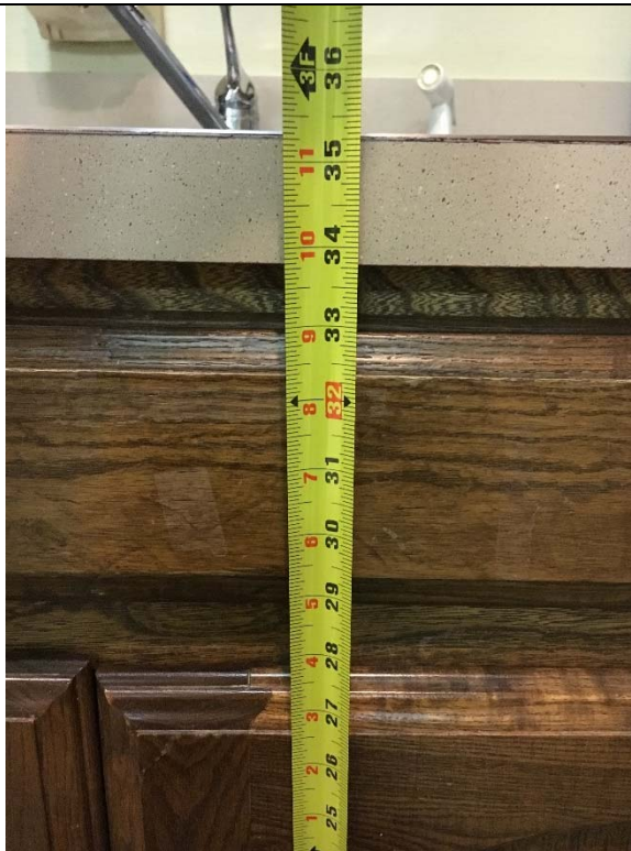
Violation 21 - The sink is mounted higher than 34" above finished floor.
