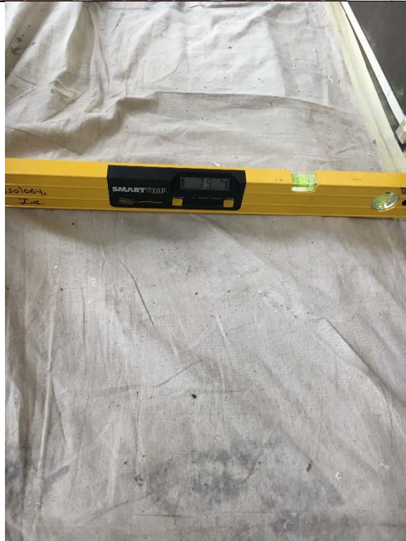
Violation 5 - The building entrance has a 7.9% sloped area at the building entrance.
