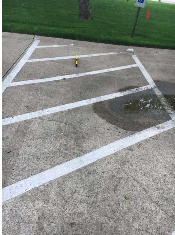
Violation 1 - The access aisle has slopes ranging from 2.4% to 4.4%.
