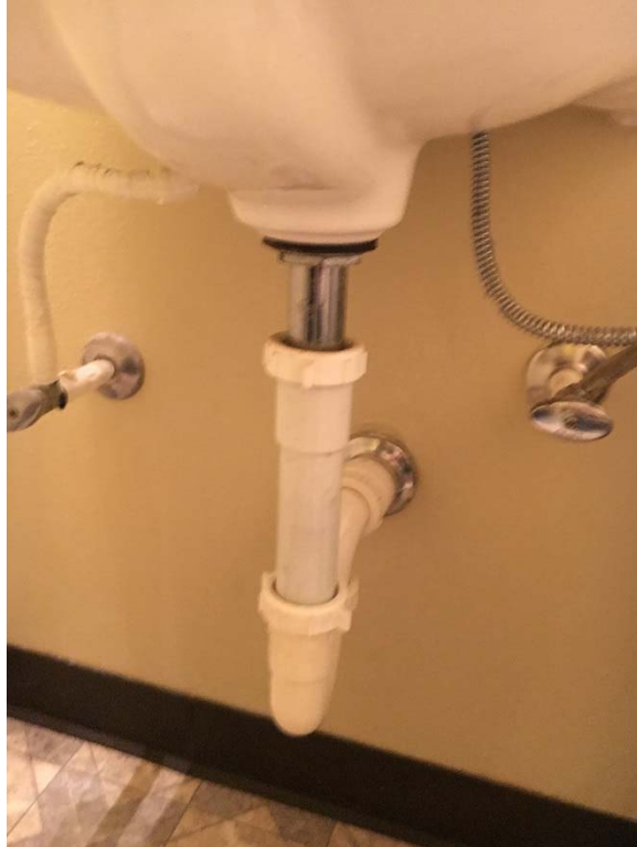
Violation 16 - Women's Restroom: Lavatory pipes and valves are not wrapped to protect against contact.
