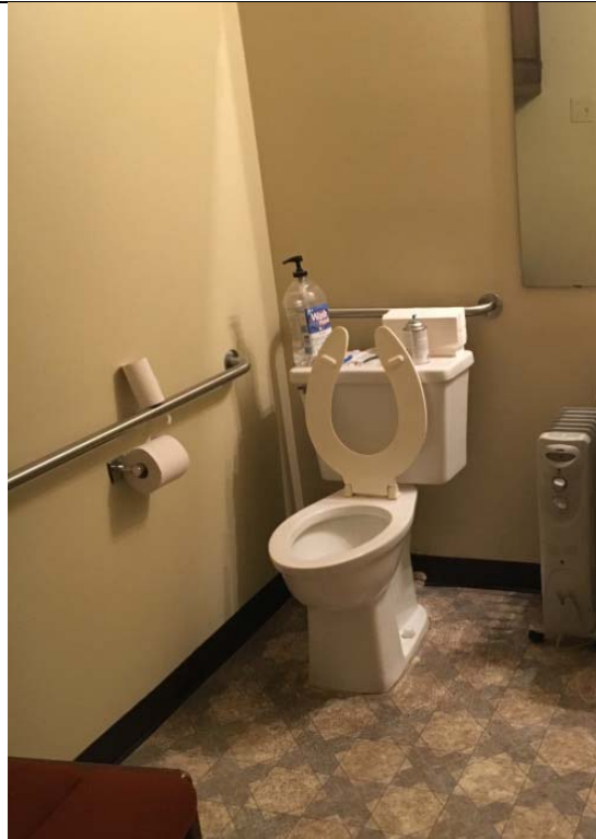
Violation 19 - Men's Restroom: The rear grab bar is only 24" long.
