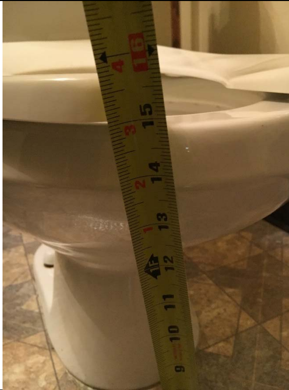
Violation 12 - Women's & Men's Restrooms: Water closet seats are 15.5" above finished floor.
