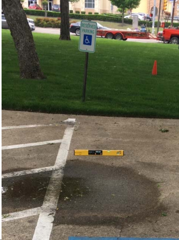
Violation 3 - The accessible signage is mounted too low.
