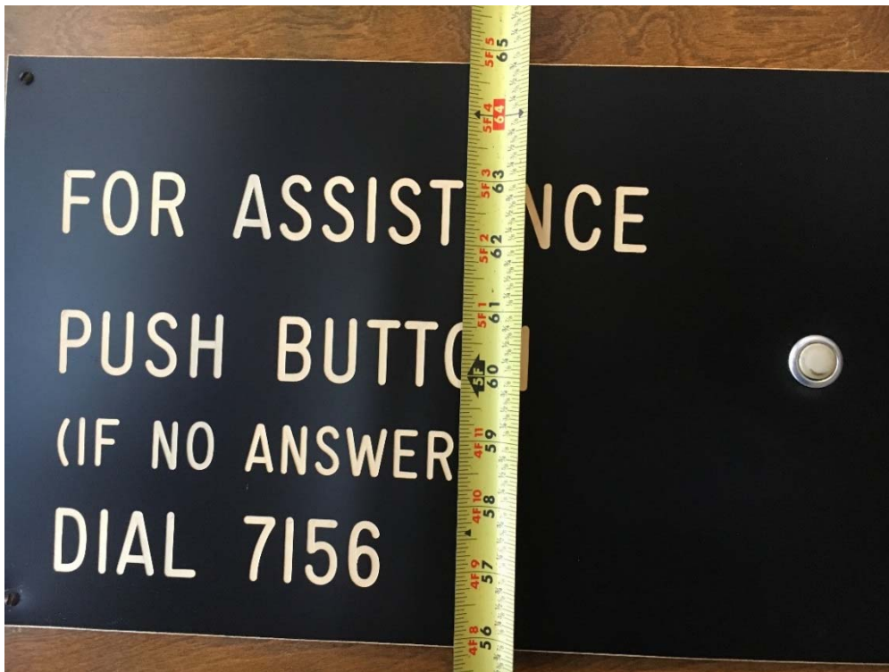
Violation 4 - The assistance signage and button in the vestibule at the main entrance is at 60-1/2" to the operable part.
