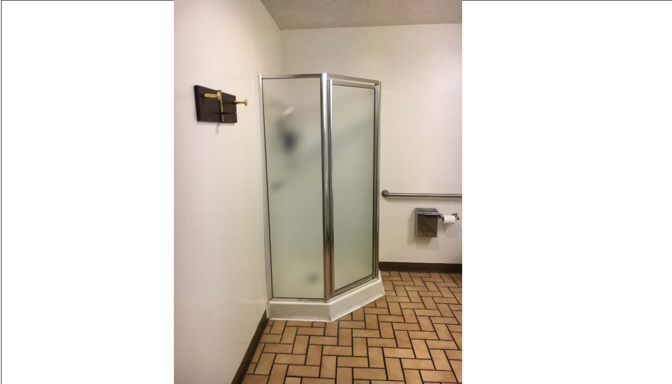
Violation 19 - Women's Restroom: Shower is not accessible.
