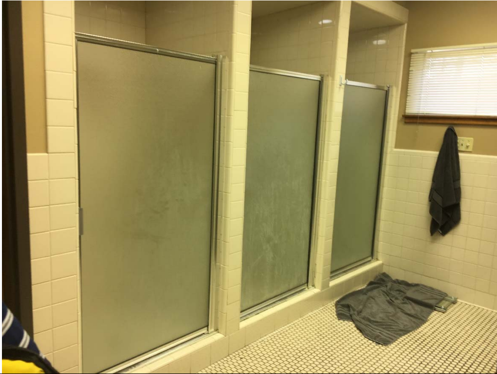
Violation 29 - The restroom in the sleeping area does not have any compliant showers.
