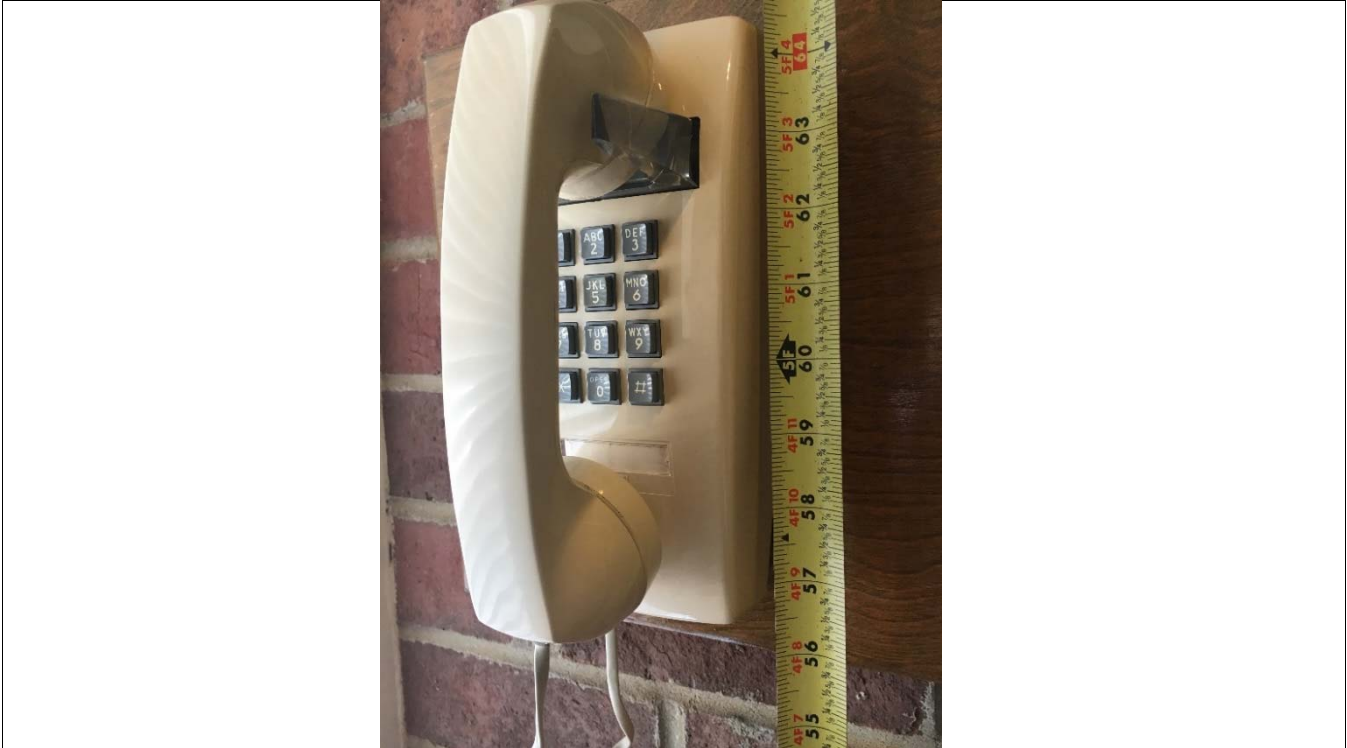
Violation 5 - The assistance phone in the entrance vestibule is mounted with the highest operable part at 63".
