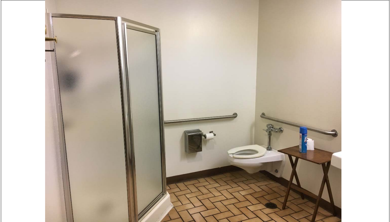
Violation 23 - Women's Restroom: The shower blocks the required clear floor space depth.
