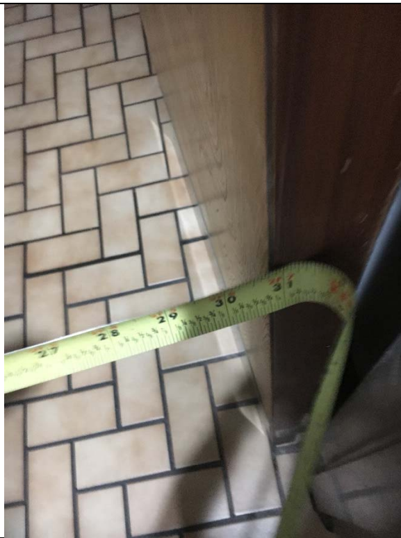
Violation 18 - Men's & Women's Restrooms: Doors only have a 31" wide opening.
