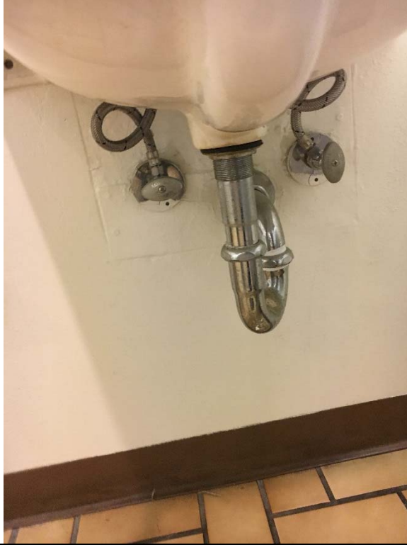
Violation 21 - The lavatory in the Men's and Women's restrooms have exposed pipes.
