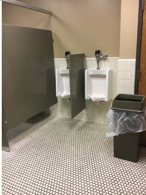
Violation 27 - The restroom in the sleeping area does not have any compliant urinals.
