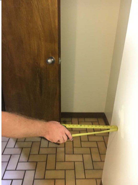
Violation 17 - Men's Restroom: There is not a 48" deep maneuvering clearance on the pull side.
