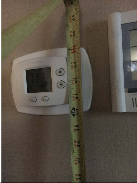
Violation 35 - The thermostat's highest operable part is at 62-3/4".
