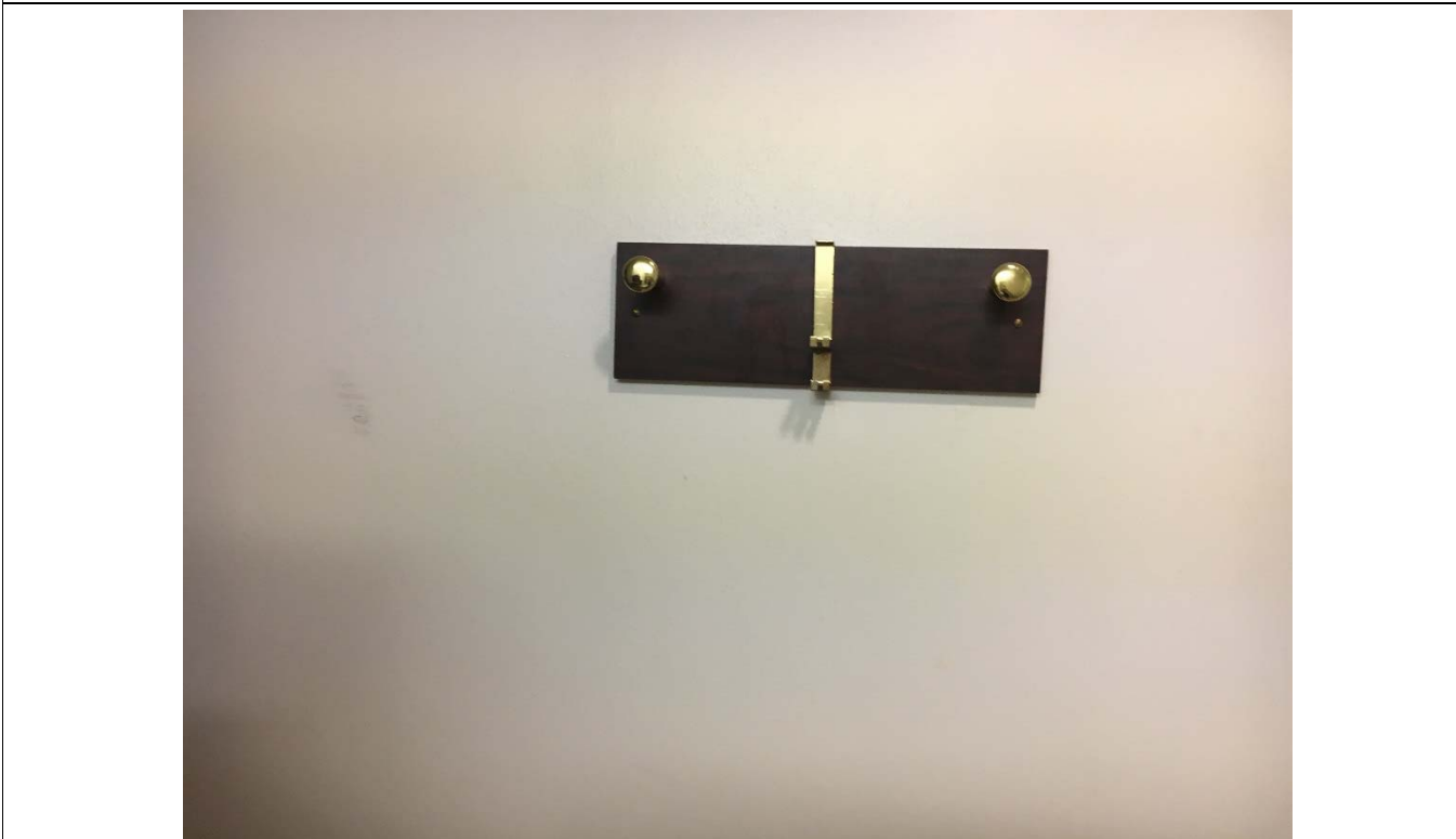
Violation 20 - Women's Restroom: Coat hooks are mounted at 65" where a maximum of 48" is required.
