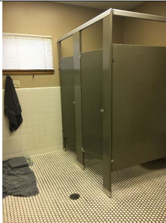
Violation 26 - The restroom in the sleeping area does not have any compliant stalls.
