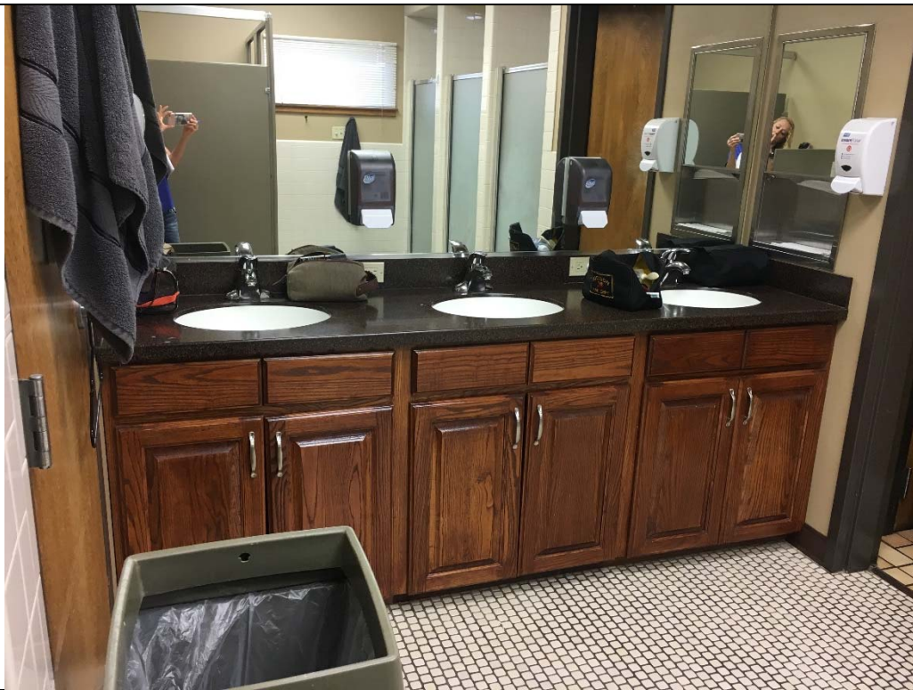
Violation 28 - The lavatories in the restroom in the sleeping area are mounted at 35-1/2" with no knee clearance.
