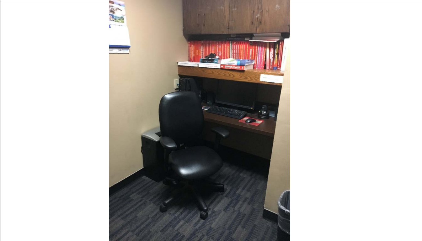
Violation 15 - The door into the office area only has a 7-1/2" maneuvering clearance on the pull side.
