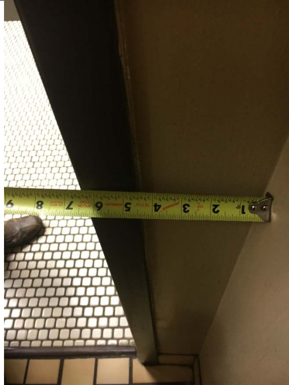
Violation 25 - The door to the restroom in the sleeping area does not have a minimum 18" maneuvering clearance on the pull side.
