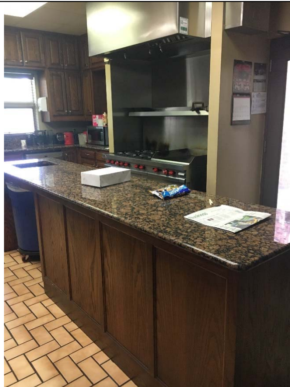
Violation 30 - The counters in the kitchenette are at 36-1/2" with no knee clearance provided.
