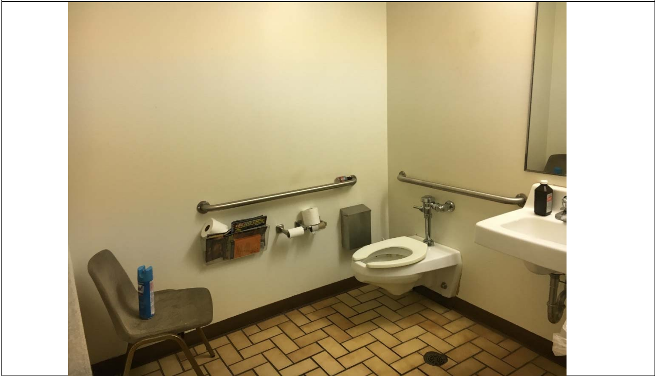
Violation 24 - Men's Restroom: The lavatory blocks the required clear floor space width.
