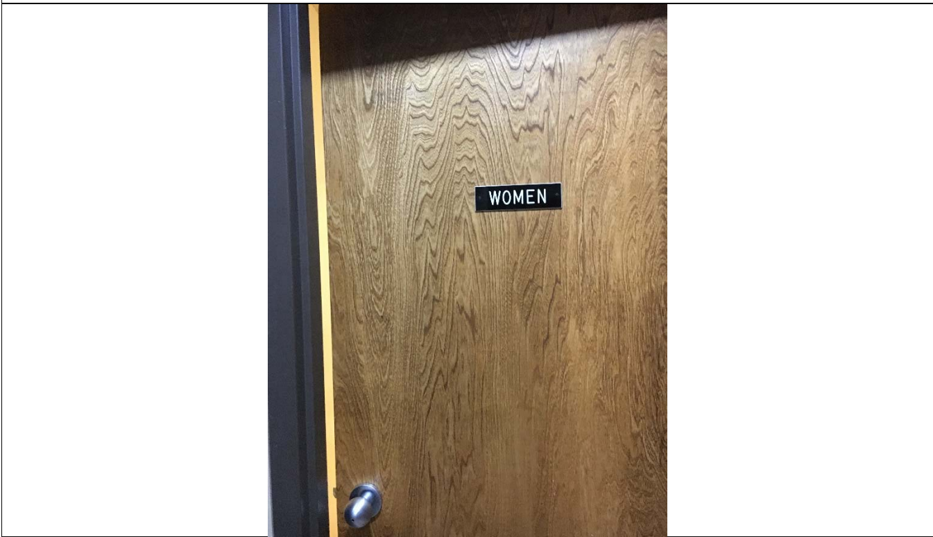
Violation 16 - Women's Restroom: Entrance door only has an 8" maneuvering clearance on the pull side where a minimum of 18" is required.
