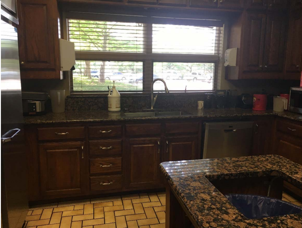
Violation 31 - The sink is mounted at 36-1/2" with no knee clearance provided.
