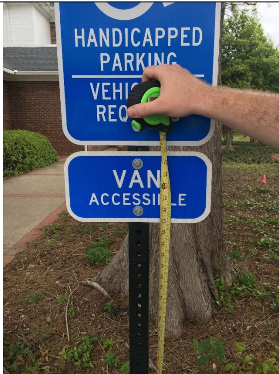
Violation 4 - Accessible parking signage is mounted too low.
