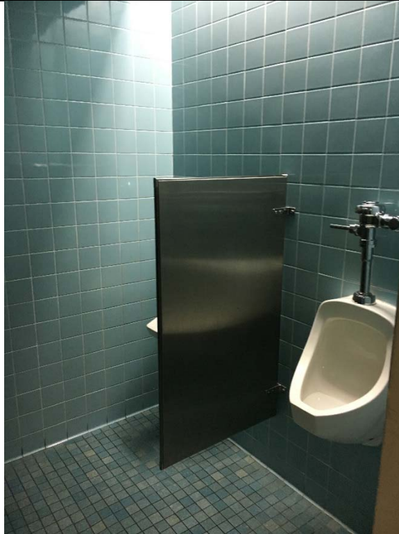
Violation 41 - Men's locker room does not have a compliant urinal.
