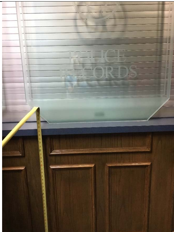
Violation 17 - The counter at the Police Records window is at 41.5" where 36" maximum is required.
