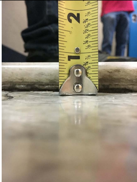
Violation 34 - There is a 3/4" change in level at the entrance door into the Women's locker room.
