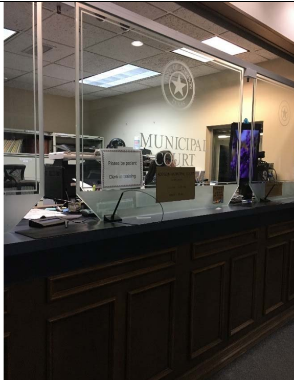
Violation 19 - The counter at the Municipal Court window is at 47 1/4" where 36" maximum is required.
