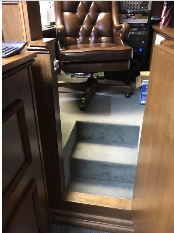
Violation 73 - There is no accessible route up to the Judge's bench, access is by stairs only.
