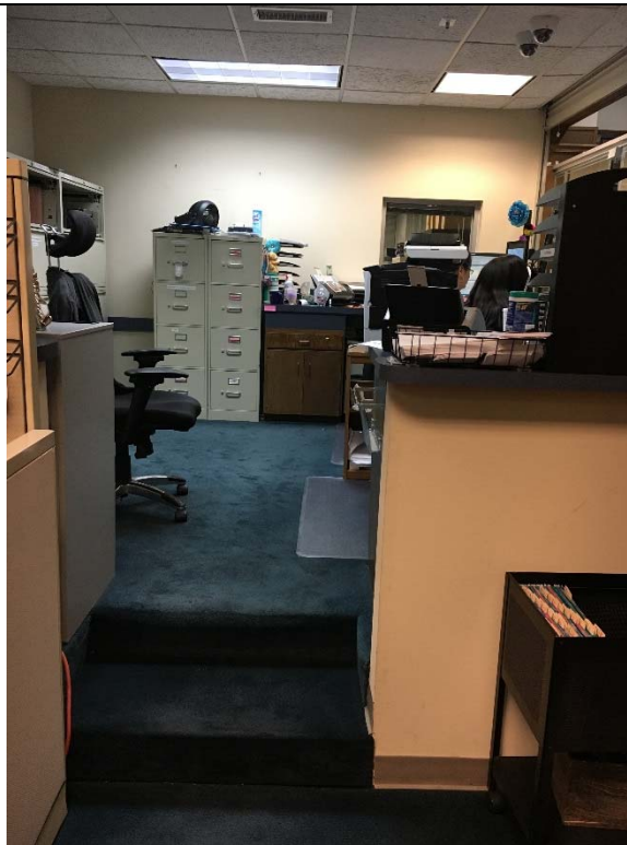
Violation 9 - There is no accessible route to the cashier work area in the Municipal Court area.
