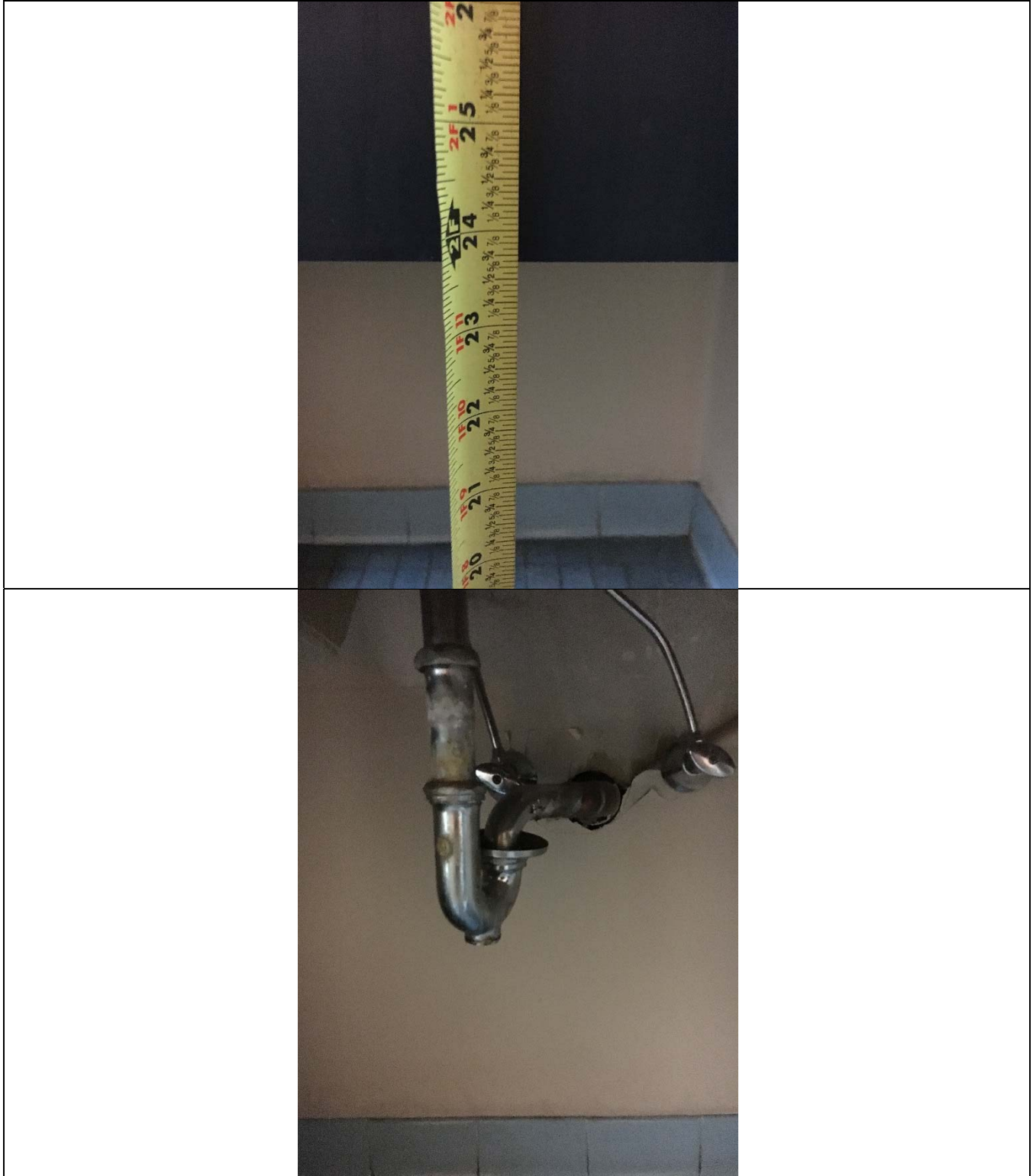
Violation 33 - The Men's restroom outside Courts and Records - The lavatory is mounted at 36" with a 24-1/16" knee clearance, the pipes are not wrapped and it has knob style handles.
