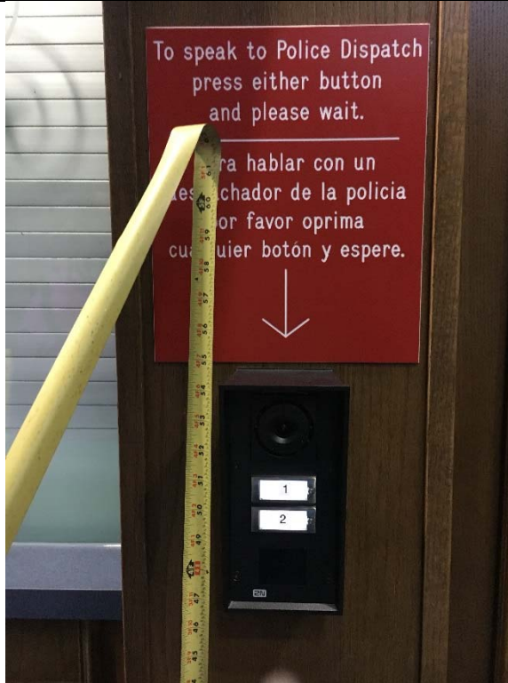
Violation 18 - The call button for Police Dispatch is mounted between 50"-51", the maximum required is 48".
