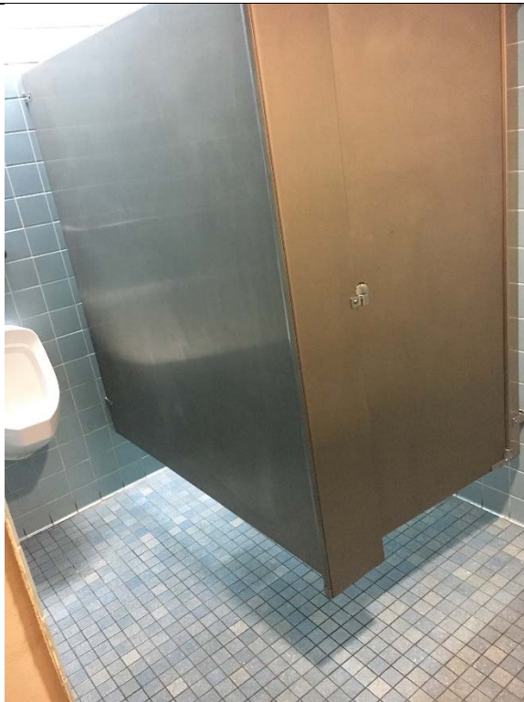
Violation 32 - The Men's restroom outside Courts and Records does not have an accessible stall.
