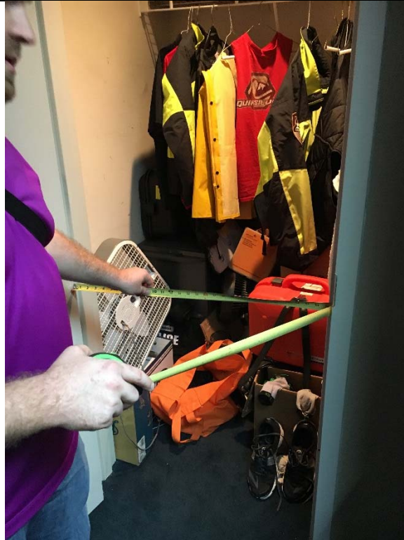
Violation 68 - The door to the storage closet has an opening of only 30" where a minimum of 32" is required.
