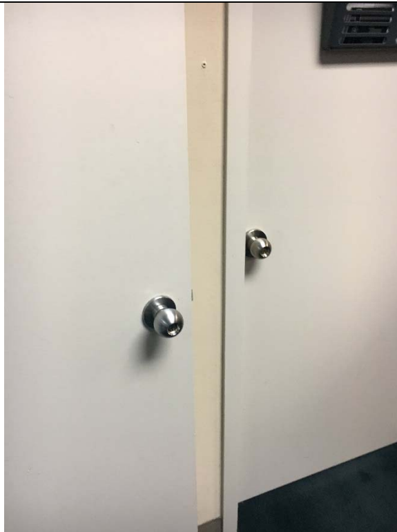
Violation 13 - All existing knob hardware requires twisting of the wrist to operate. There are approximately 45 doors throughout the facility that are equipped with knob hardware.
