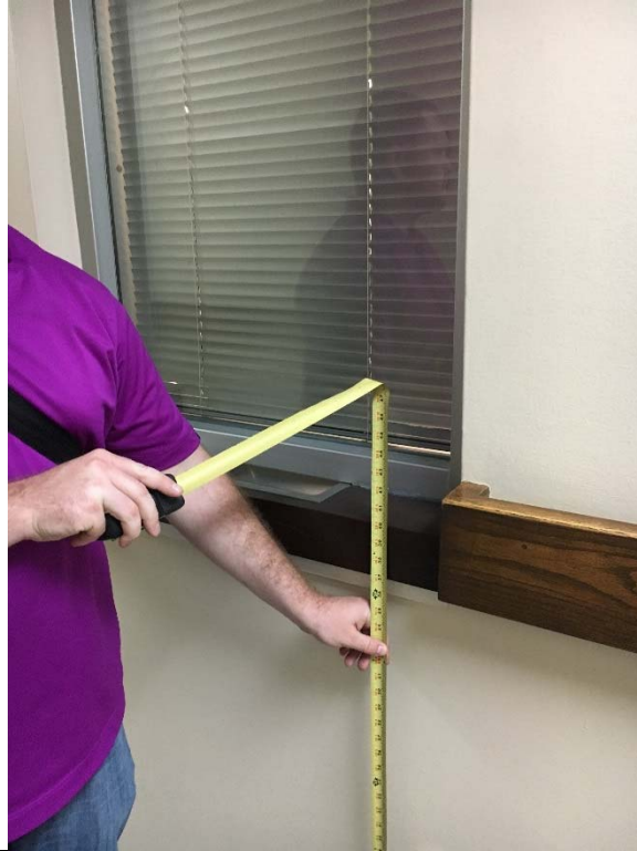
Violation 64 - The transaction window counter is at 40" where a max of 36" is required.
