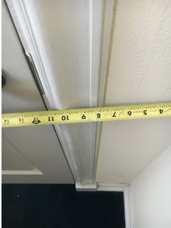
Violation 24 - Janitorial supply room on the second floor only has an 11" maneuvering clearance on the pull side where a minimum of 18" is required.
