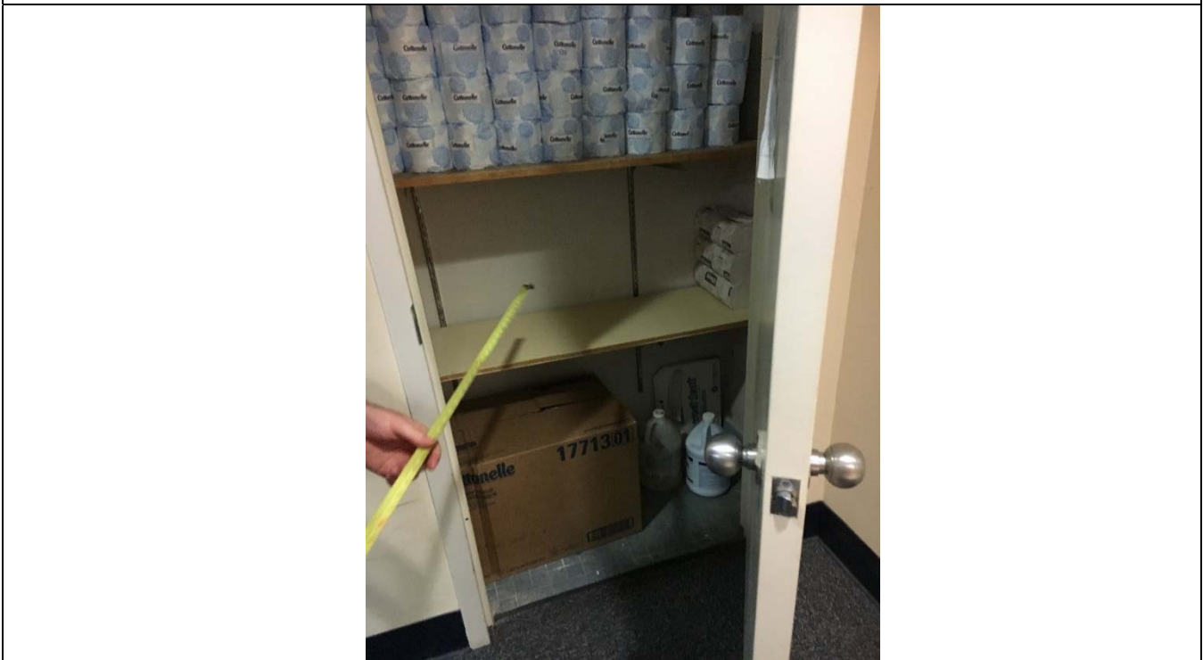
Violation 63 - The storage room in the Men's locker room has a door width of only 29", a minimum of 32" is required.
