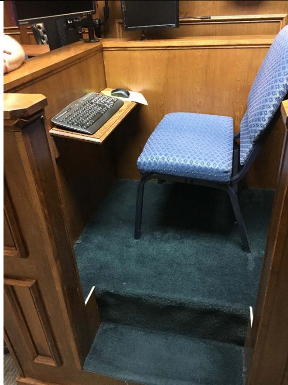
Violation 72 - An accessible route is not provided up to the witness stand and it does not have a clear floor space provided within its defined area
