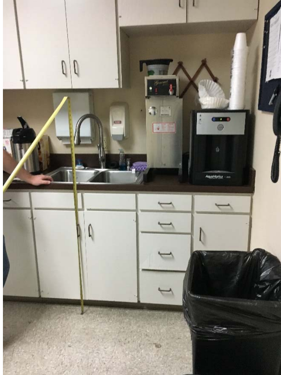
Violation 52 - Second floor break room sink/counter is at 36-1/4" where the maximum height is 34".
