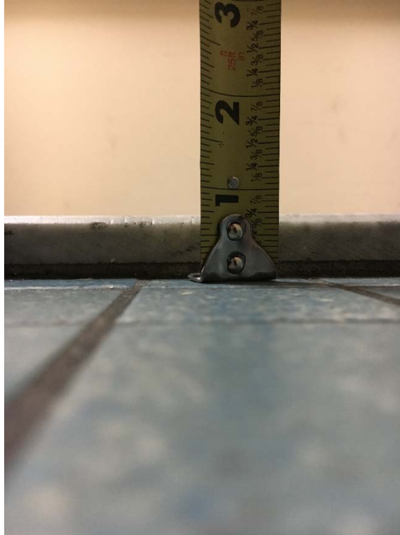
Violation 31 - The Men's restroom outside Courts and Records has a 5/8" change in level to enter the restroom.
