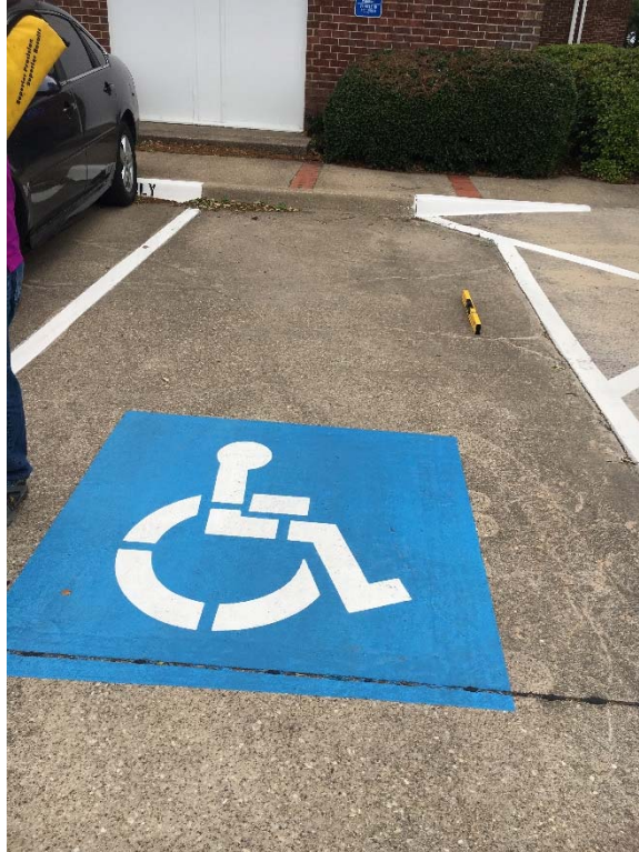
Violation 3 - The far left accessible parking space has a running slope of 2.6%.
