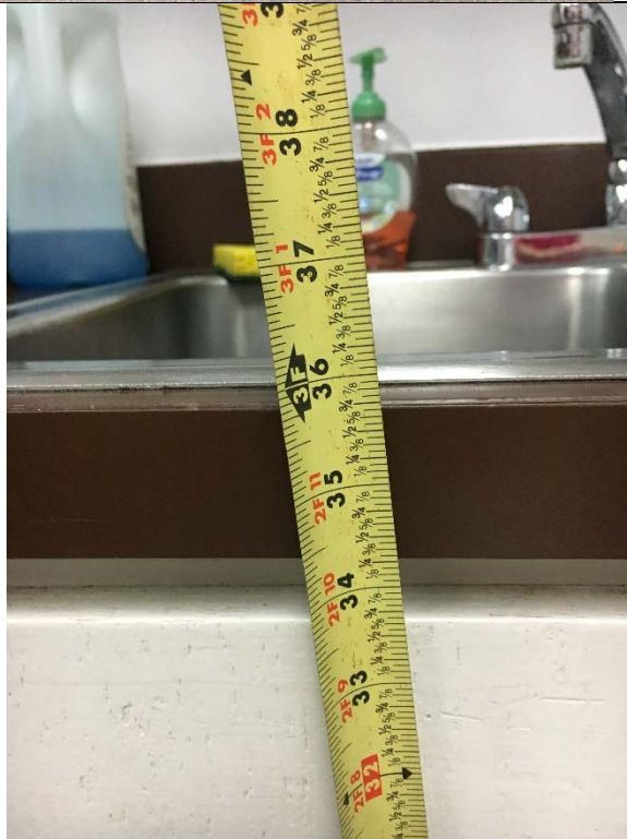
Violation 51 - First floor break room sink/counter is at 35-3/4" where the maximum height is 34".
