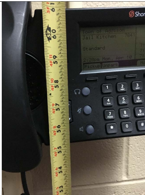
Violation 53 - The phone provided in the jail kitchen has the highest operable part at 59" where a maximum of 48" is required.
