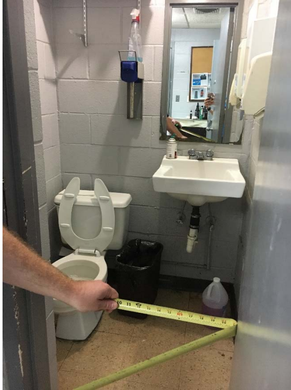
Violation 26 - The restroom in the gun range is not large enough to accommodate a wheelchair turning space.
