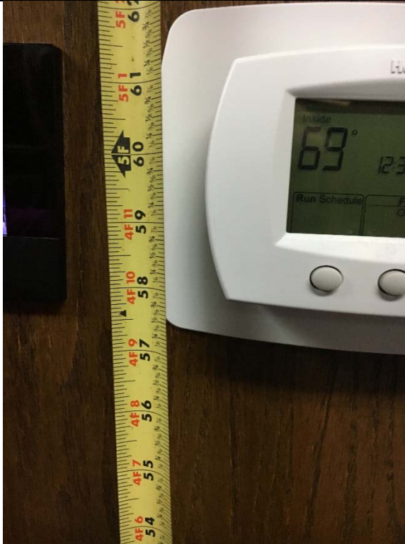
Violation 70 - The thermostat in the court room is mounted with the highest operable part at 58" where a maximum of 48" is required.
