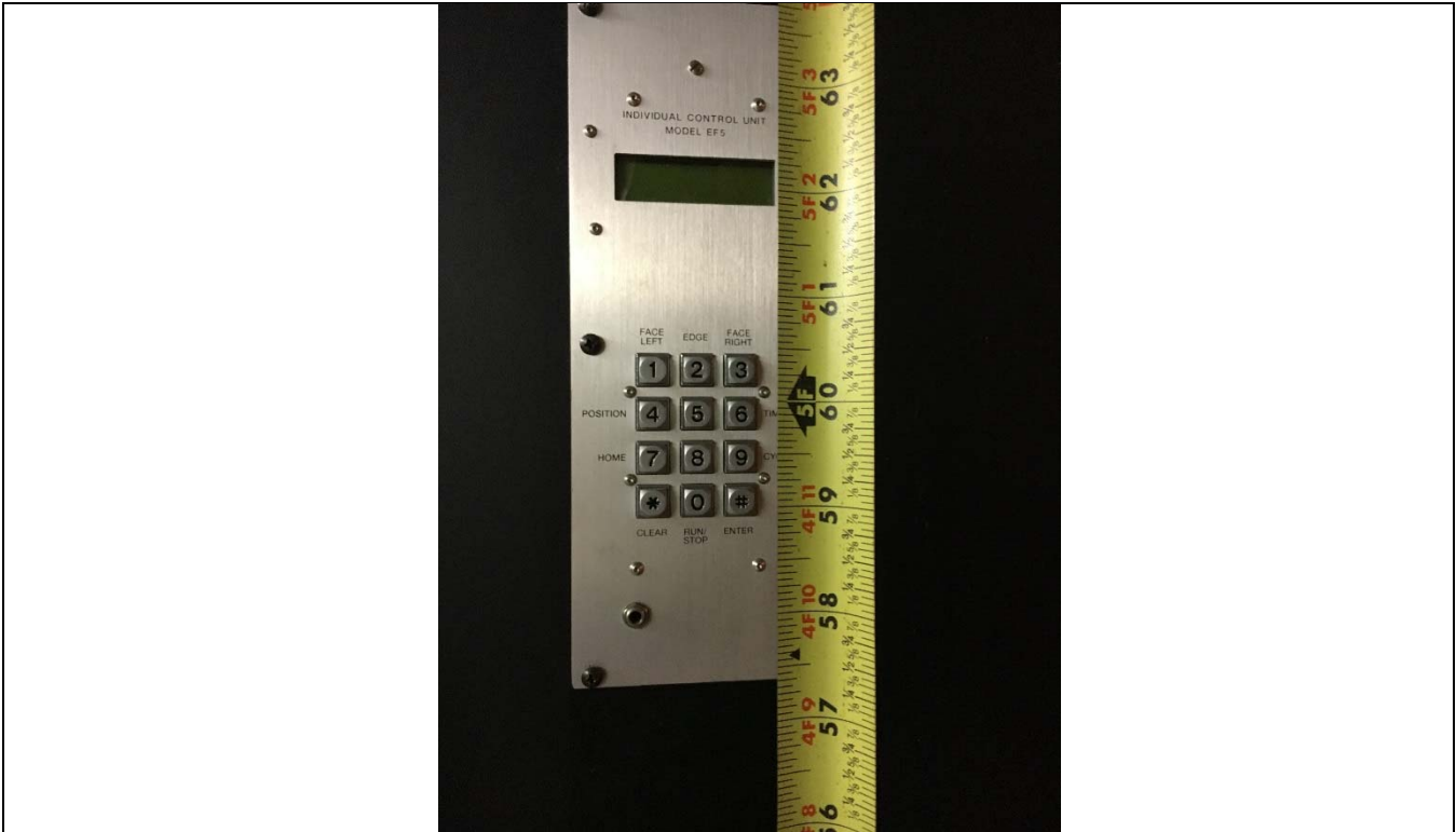
Violation 62 - The keypad in the gun range has the highest operable part over 60" where a maximum of 48" is required.
