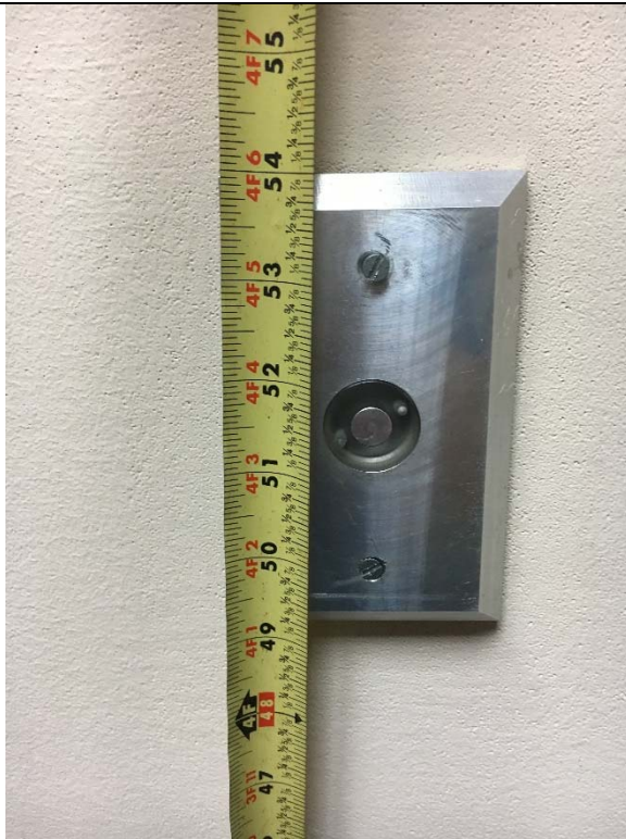
Violation 69 - Height of the button in court room is at 51.5" where a maximum of 48" is required.
