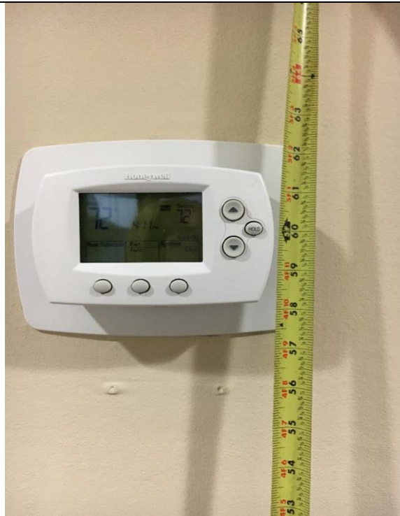
Violation 71 - The thermostat on the second floor is mounted with the highest operable part at 60.5" where a maximum of 48" is required.
