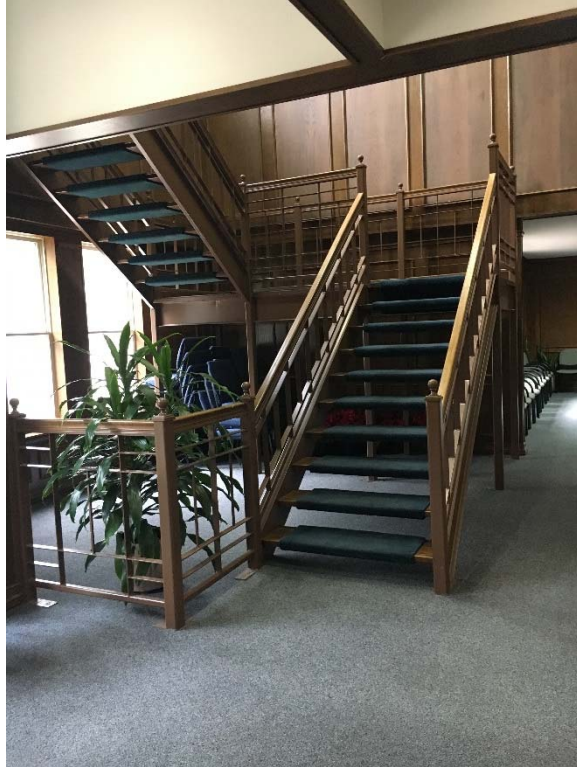
Violation 5 - There is no accessible route to the 2nd floor of the facility.
