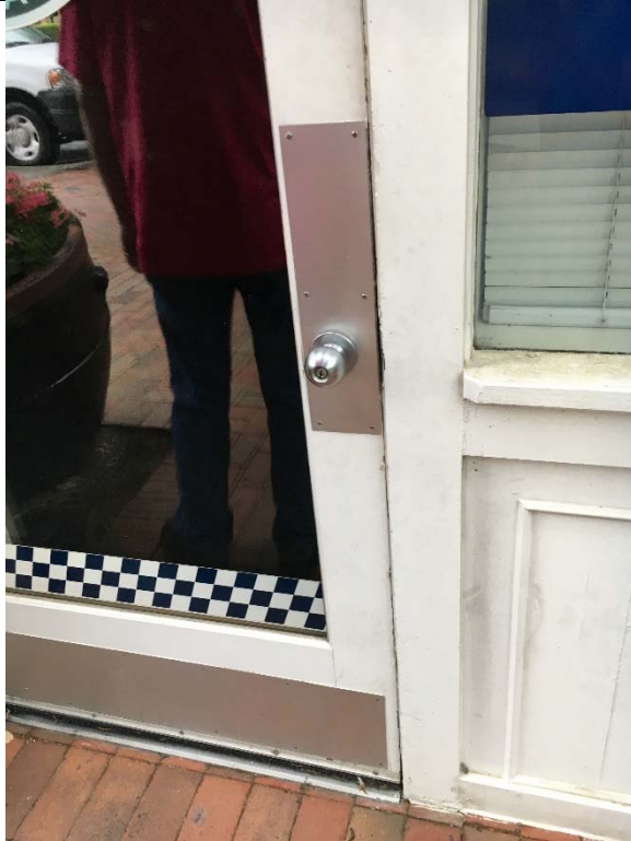
Violation 1 - The entrance door has knob hardware requiring grasping and twisting to operate.
