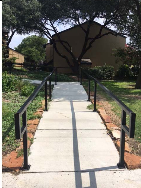
Violation 2 - The ramp leading to the building entrance has no edge protection.
