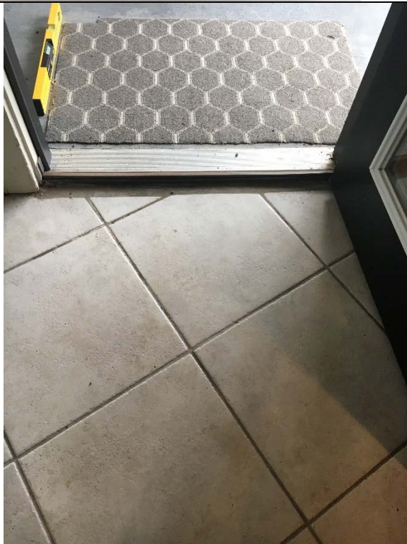
Violation 5 - There is a 3/8" threshold at the entrance door.
