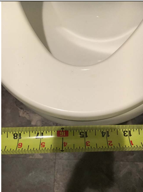
Violation 10 - The centerline of the water closet is only at 15".
