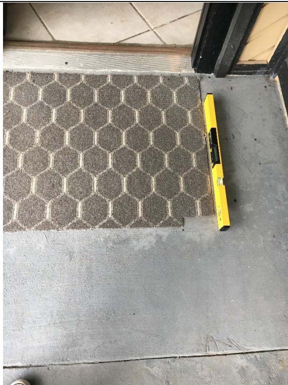
Violation 4 - There is a 5.5% running slope up to the entrance door.
