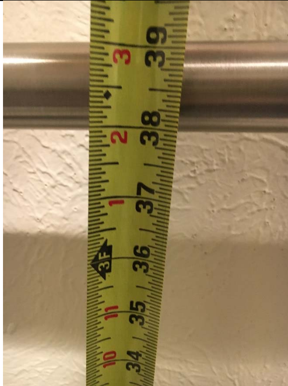
Violation 11 – The grab bars are mounted at 39" above finished floor to the top of the gripping surface.
