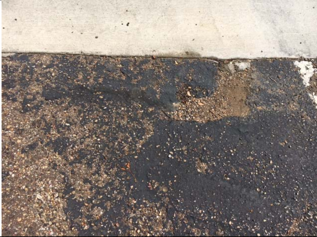
Violation 3 - The bottom section of the ramp where it connects to the parking lot has uneven and broken concrete.
