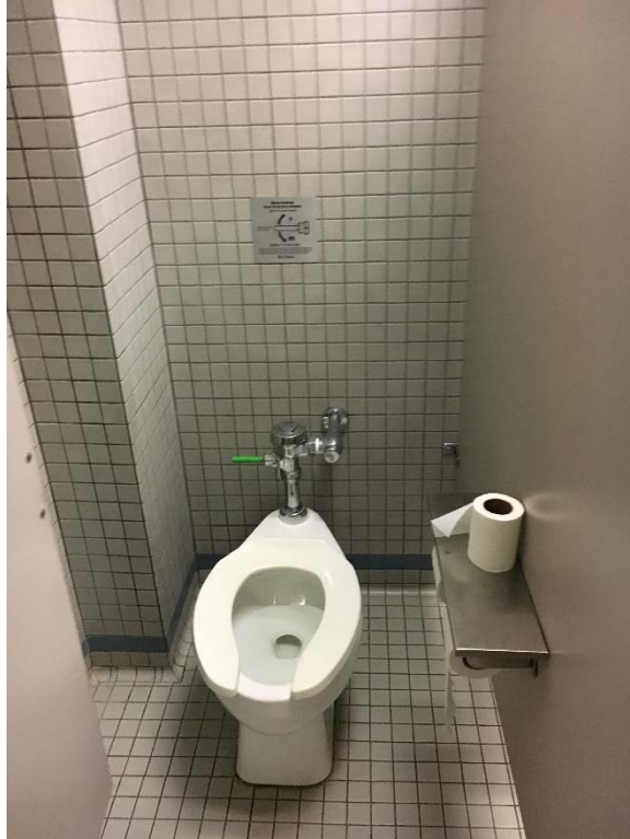
Violation 25 - Breakroom Area: Women's restroom does not have an accessible toilet compartment.
