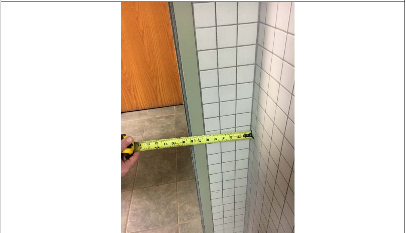
Violation 32 - 1st floor lobby: Men's restroom door only has 8" maneuvering clearance on the pull side and the door requires more than 5lbs of pressure to operate.
