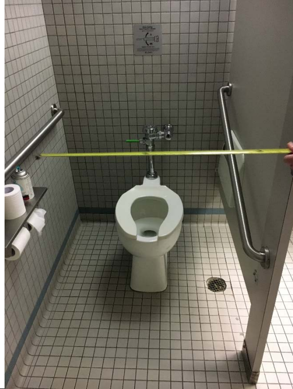
Violation 39 - 2nd floor: Men's restroom does not have an accessible toilet compartment.
