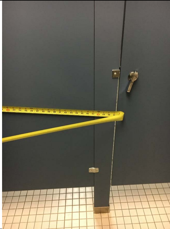
Violation 35 - 1st floor lobby: Men's restroom stall door swings into the stall and only has a 30" wide opening.
