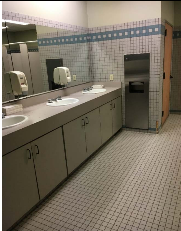
Violation 18 - Breakroom Area: Men's room lavatory does not have the required knee clearance provided and the counter is too high at 36-1/4" above finished floor.
