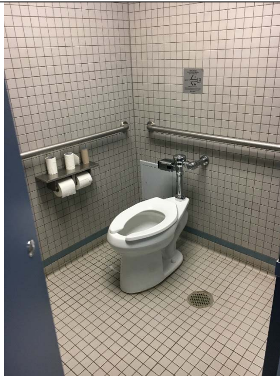
Violation 34 - 1st floor lobby: Men's restroom accessible toilet compartment is only 51-1/2" deep.
