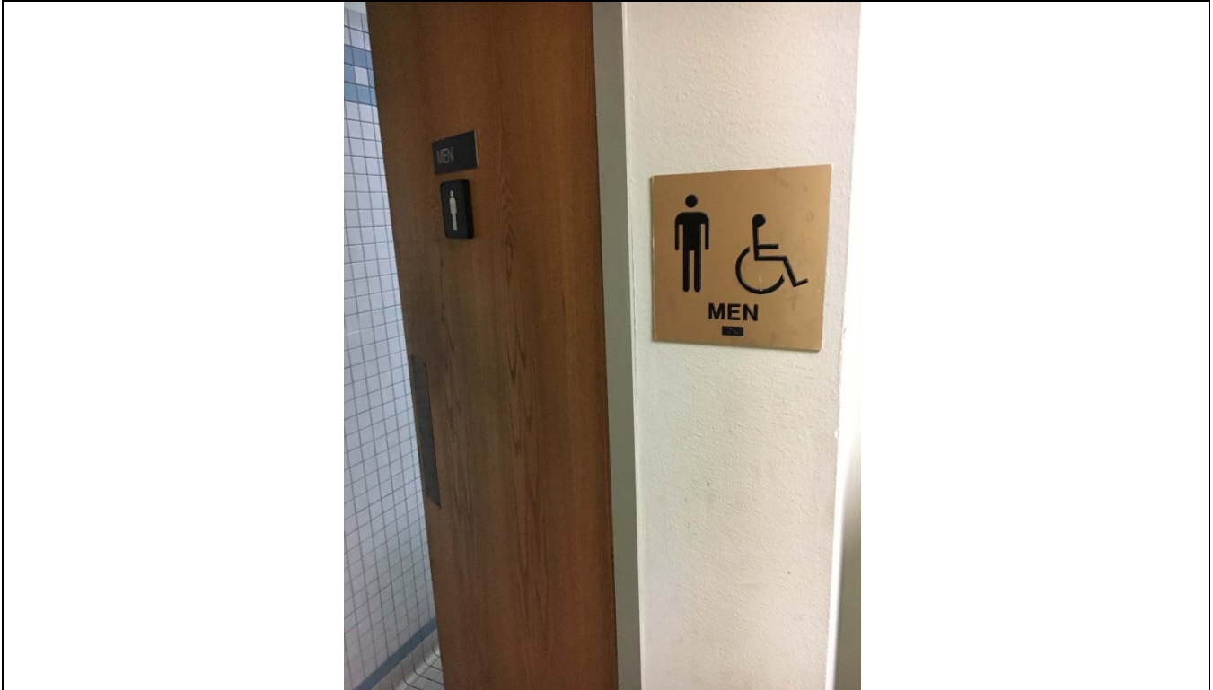
Violation 31 - 1st floor lobby: Men's room signage is mounted on the hinge side of the door.
