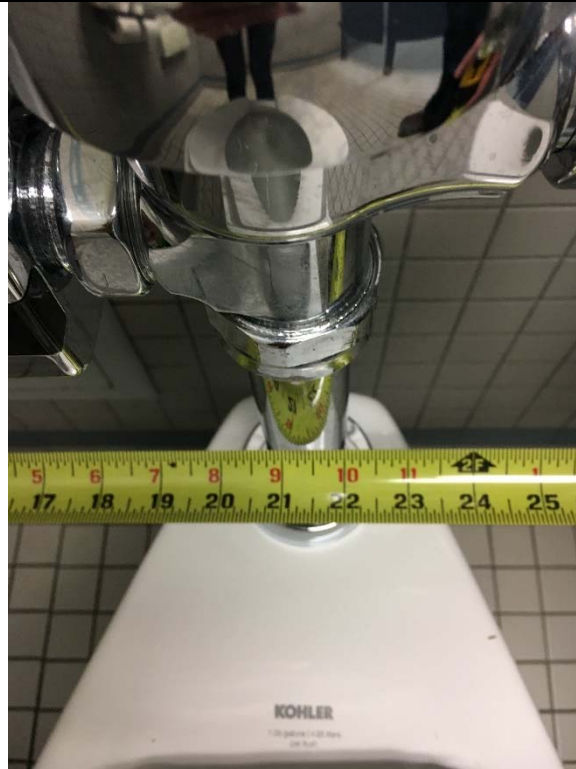
Violation 33 - 1st floor lobby: Men's room water closet in accessible stall is 21-1/2" to its centerline.
