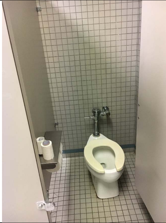
Violation 21 - Breakroom Area: Men's restroom does not have an accessible toilet compartment.
