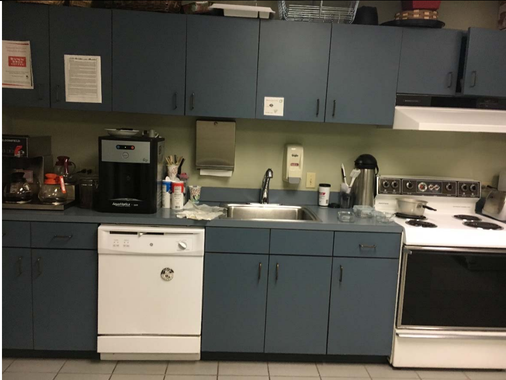
Violation 45 - The counter/sink in the 2nd floor break room is at 36" above finished floor.
