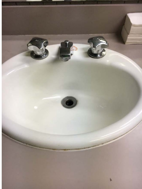
Violation 19 - Breakroom Area: Men's room lavatory faucets require grasping and twisting to operate.
