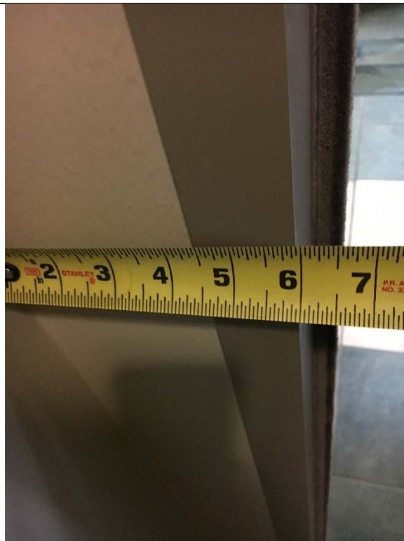
Violation 28 - 1st floor lobby: Women's room door only has a 6" maneuvering clearance on the pull side and the door requires more than 5lbs of pressure to operate.
