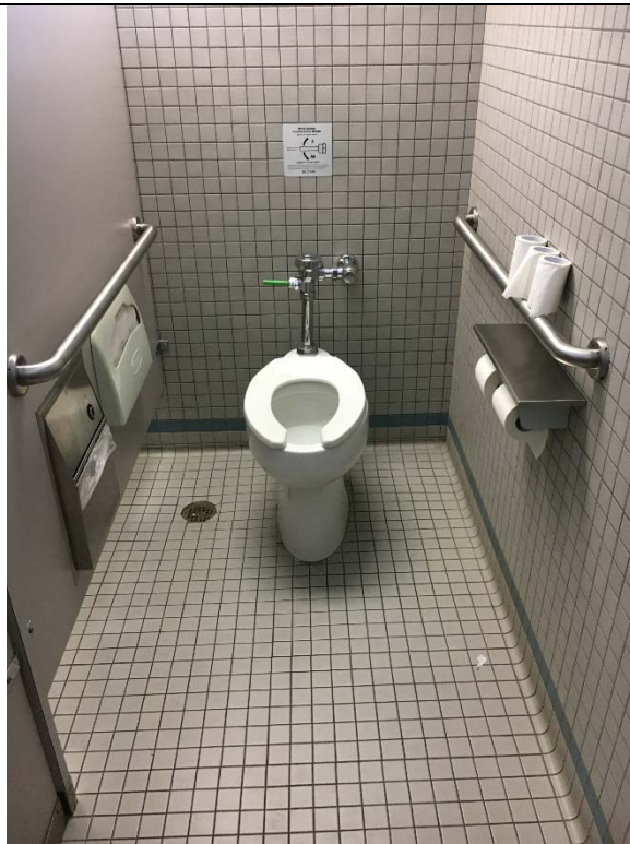
Violation 42 - 2nd floor: Women's restroom does not have an accessible toilet compartment.
