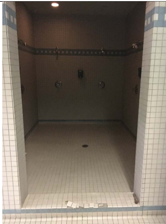
Violation 22 - Breakroom Area: Men's restroom does not have an accessible shower compartment.
