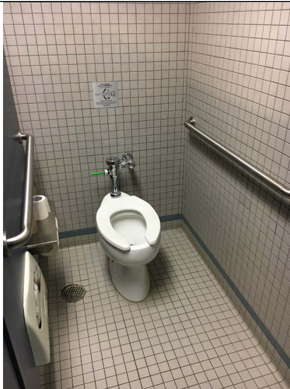
Violation 30 - 1st floor lobby: Women's room does not have an accessible toilet compartment.
