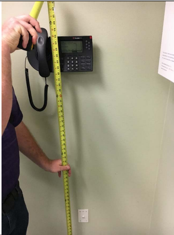
Violation 46 - The phone provided in the break room on the 2nd floor is mounted at 56" to the highest operable part.
