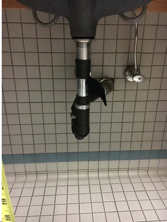
Violation 41 - 2nd floor: Women's restroom lavatory pipes are not protected against contact.
