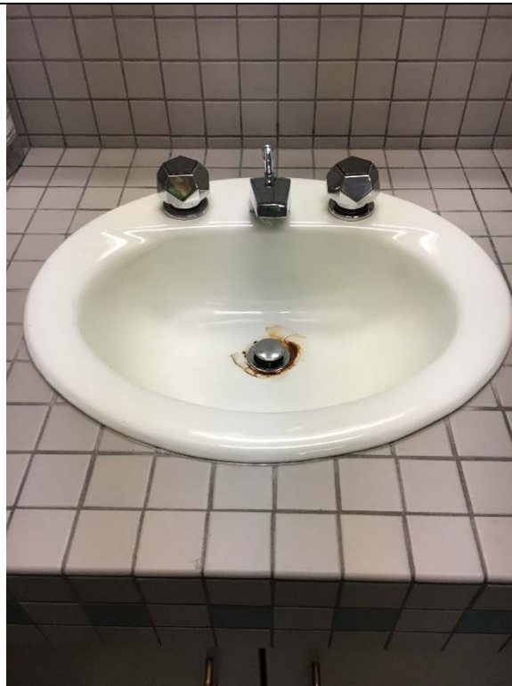
Violation 24 - Breakroom Area: Women's restroom lavatory faucets require grasping and twisting to operate and it does not have the required knee clearance.
