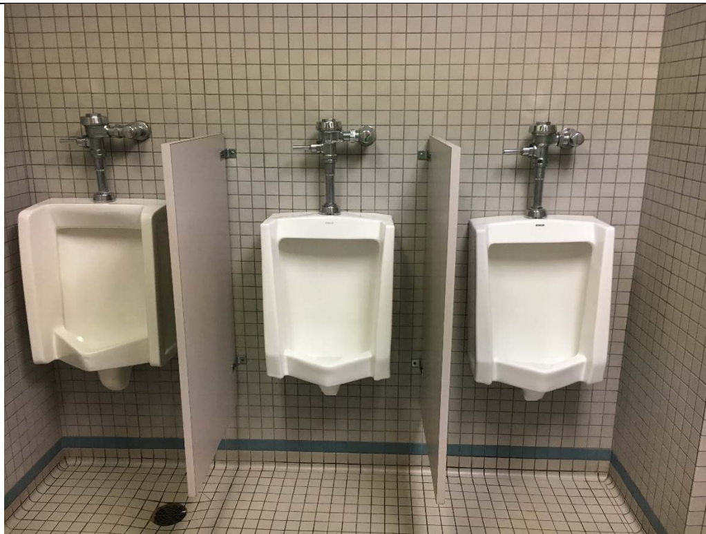
Violation 20 - Breakroom Area: Men's room has 3 urinals and no accessible urinal is provided.
