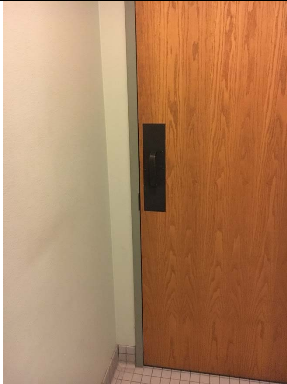
Violation 17 - Breakroom area: Men's and Women's restroom doors require more than 5lbs of pressure to operate.
