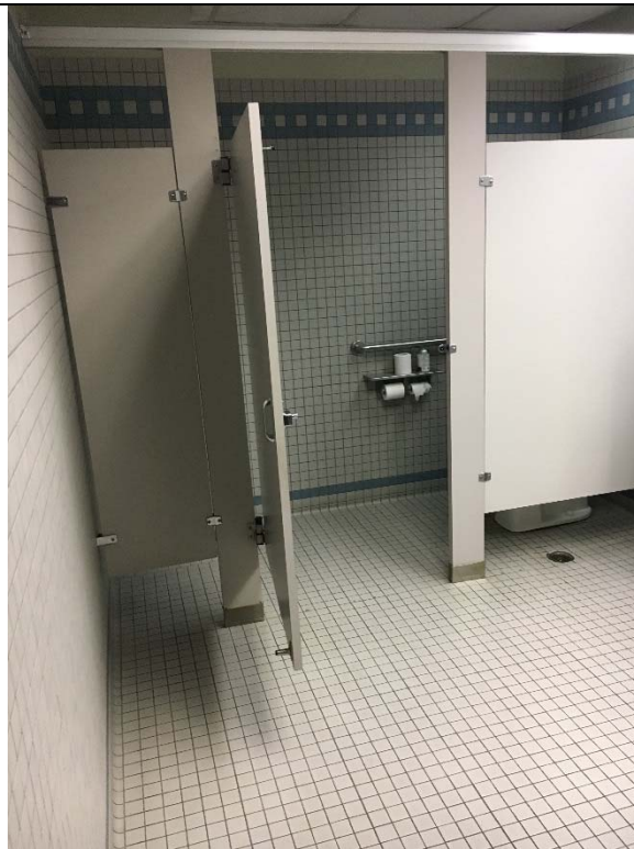
Violation 40 - 2nd floor: Men's restroom accessible toilet compartment door is not self-closing.
