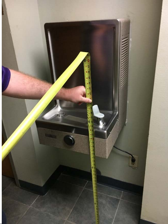
Violation 51 - There is only one drinking fountain provided in the front lobby area, two are required.
