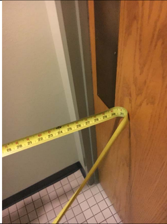
Violation 29 - 1st floor lobby: Women's room has 2 doors in a series to enter with only 31" between each door.
