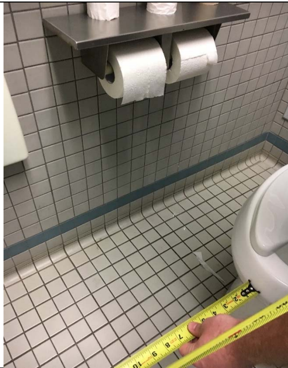
Violation 36 - 1st floor lobby: Men's restroom toilet paper dispenser is mounted too close to the back wall.
