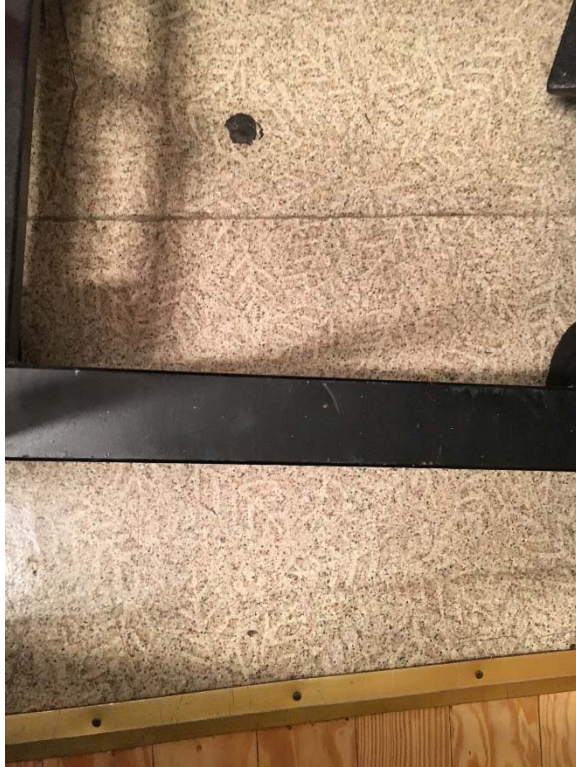
Violation 7 - The storage room at the back has a small ramped area at the threshold as you exit the room.
