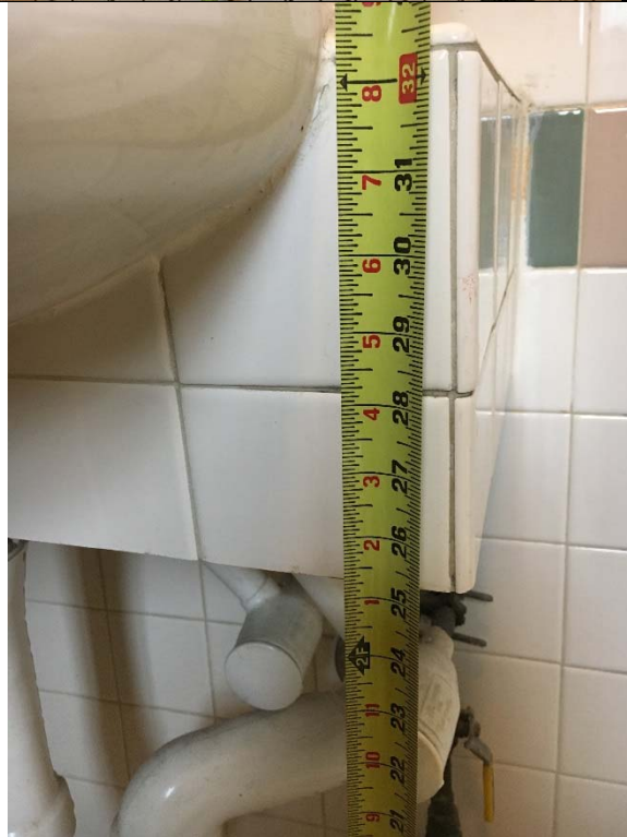
Violation 6 - The lavatory is sitting on a ceramic shelf resulting in a knee clearance of only 25" where a minimum of 27" high knee clearance is required.
