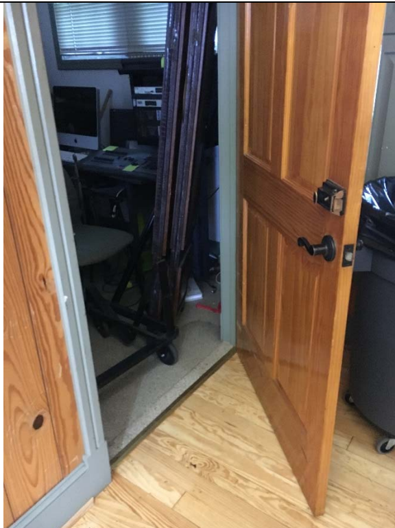
Violation 8 - The storage room door does not have an 18" maneuvering clearance on the pull side.
