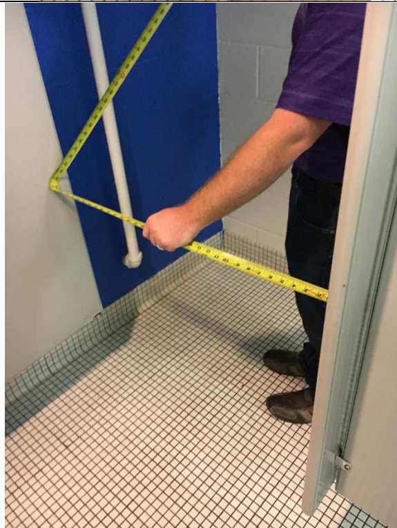
Violation 12 - Men's Restroom - Accessible stall is only 36.5" wide.
