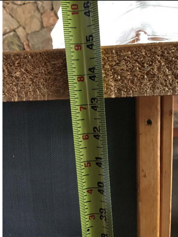
Violation 5 - The concessions stand counter is at 45" above finished floor to the counter.
