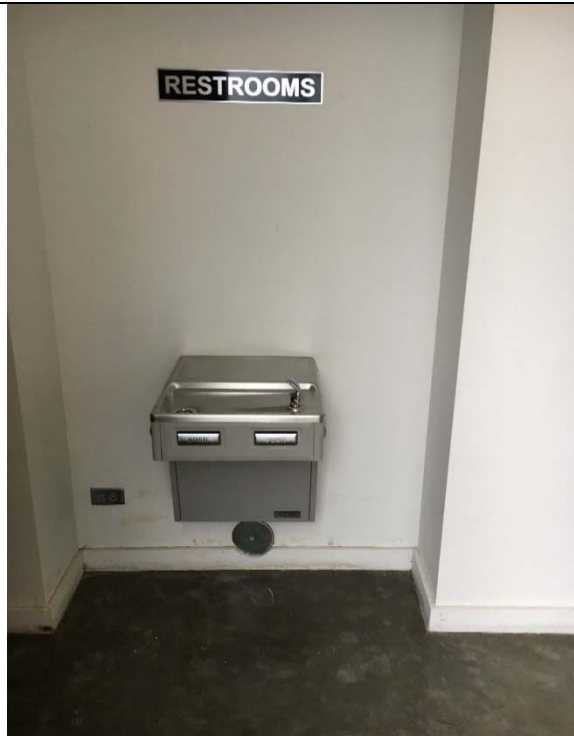
Violation 18 - There is only one drinking fountain provided on the second floor, two are required.
