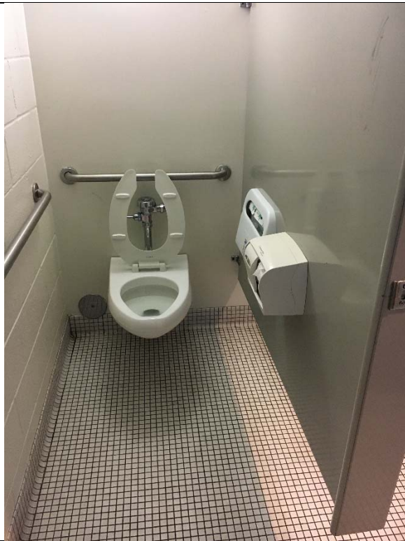
Violation 14 - Men's Room - Flush control is on the closed side of the stall.
