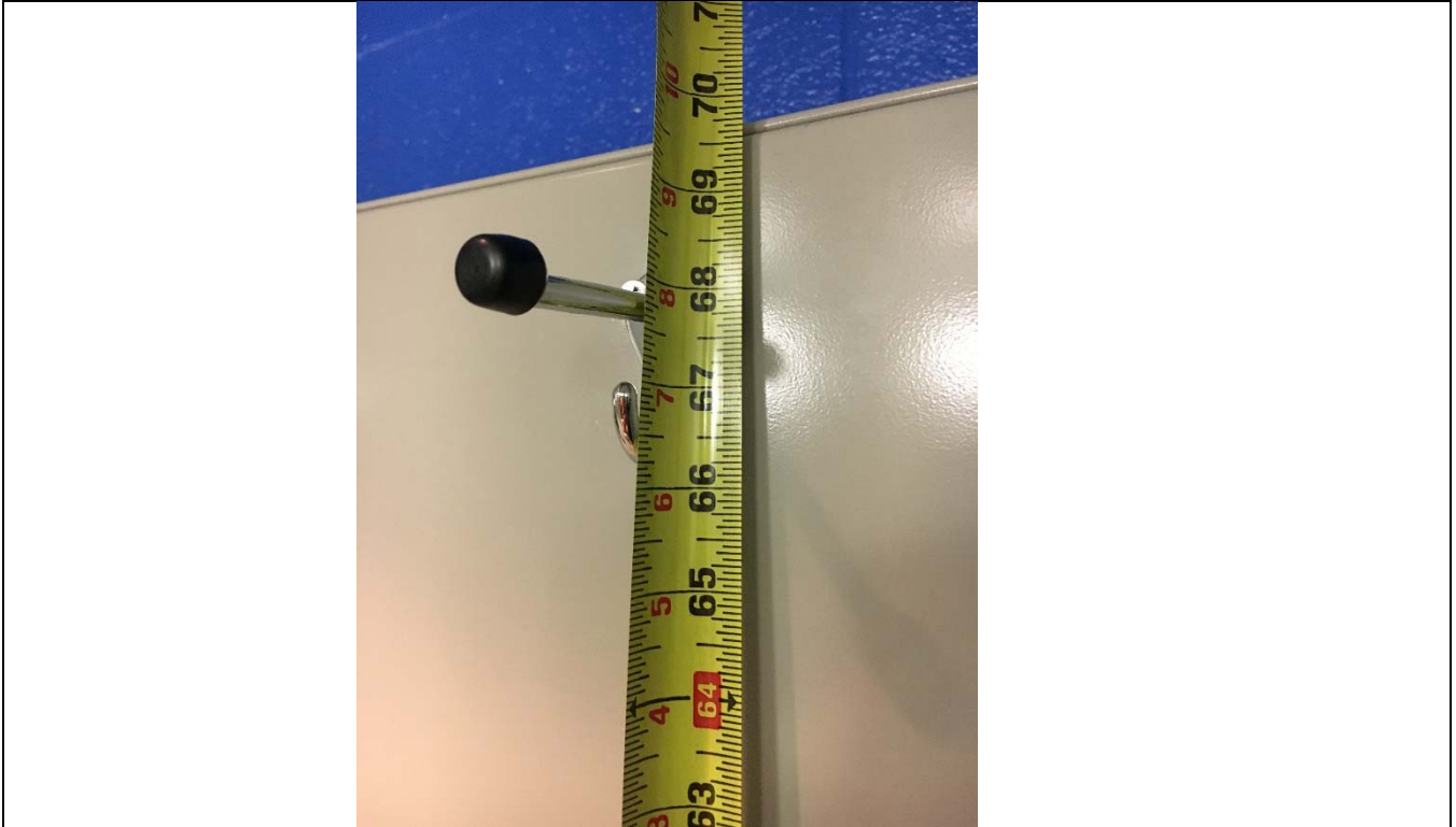
Violation 15 - Men's Restroom - Coat hook is mounted at 66.5" above finished floor.
