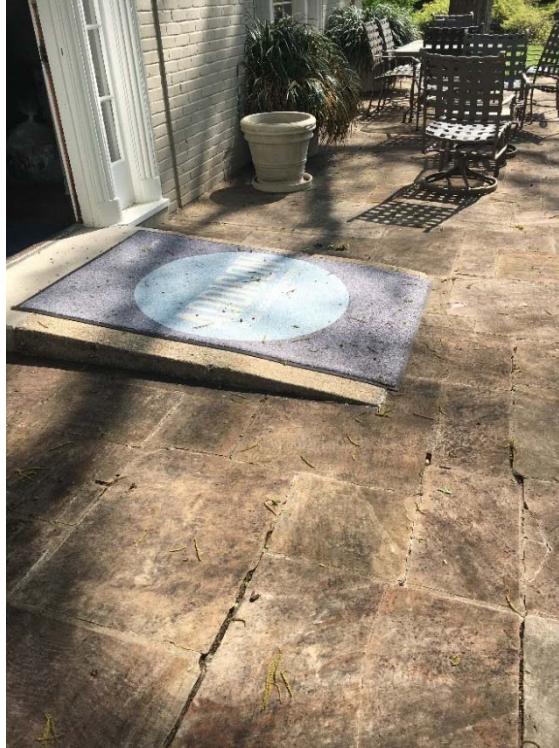
Violation 13 - The far right entrance at the back is ramped to the entrance and does not have a level landing.
