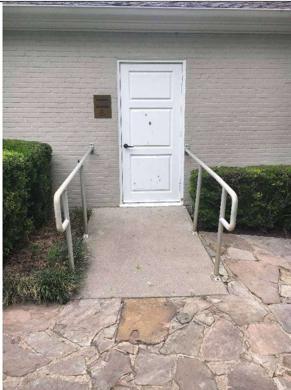
Violation 6 - The entrance leading into the Council of Chambers has a ramp with a running slope from up to 9.9%.
