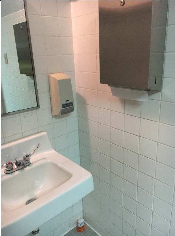
Violation 38 - Men's Room: The operation portion of the paper towel dispenser is at 50" above finished floor.
