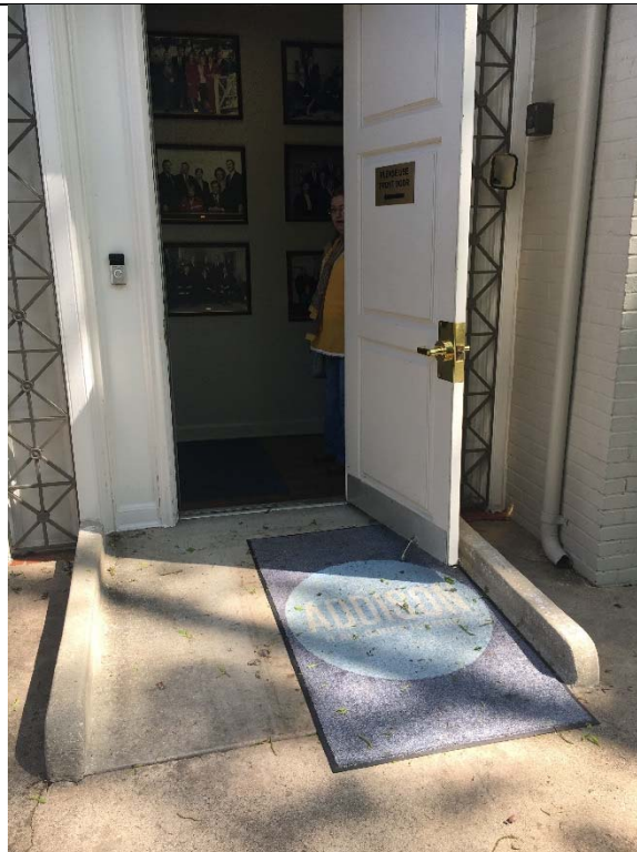
Violation 12 - The back middle entrance door does not have a minimum of 18" on the pull side.
