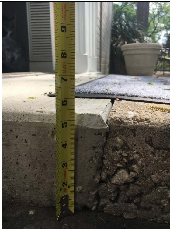
Violation 14 - The ramp up to the far right back entrance has a 5-3/8" drop off with no edge protection.
