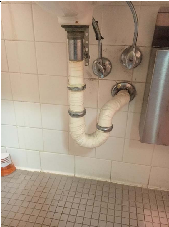
Violation 24 - Women's Room: Lavatory pipes and controls are not protected against contact.
