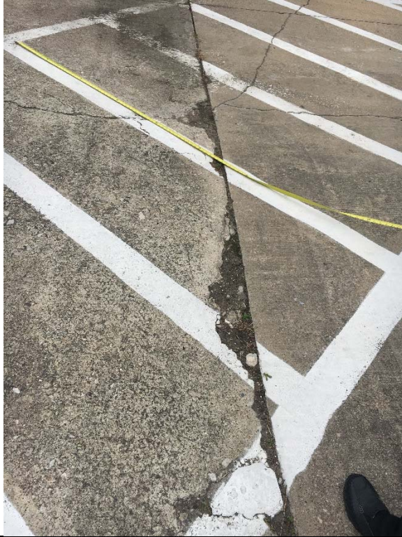
Violation 3 - The access aisle has broken concrete.
