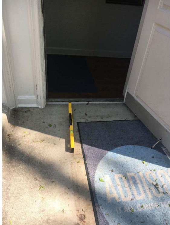
Violation 11 - The middle entrance at the back that leads to the restrooms has an 8% running slope at the landing. Additionally, the floor mat at the door is not secured to the ground.
