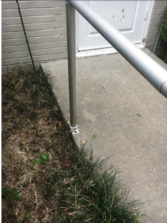
Violation 7 - The ramp at the Council of Chambers entrance does not have edge protection.
