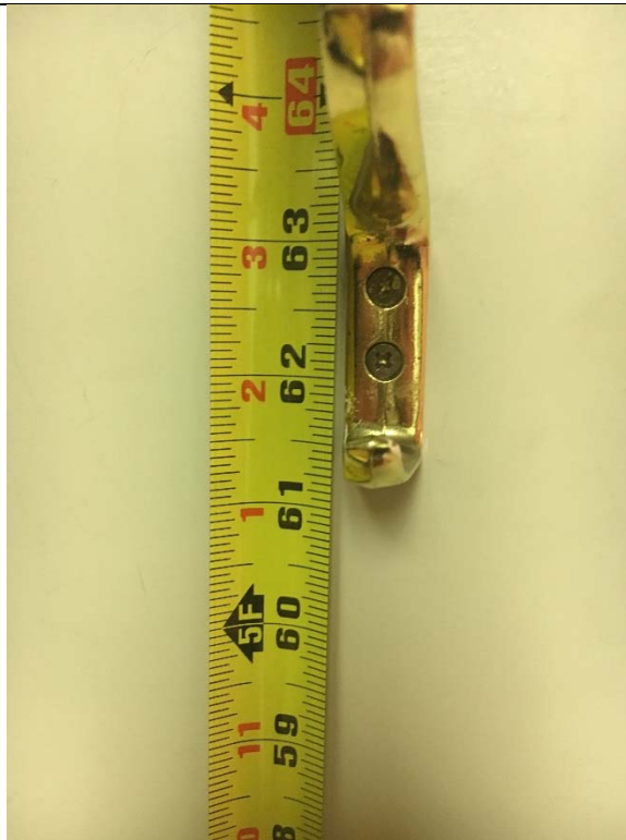
Violation 31 - Women's Room: Coat hook is mounted at 61-1/2" above finished floor.
