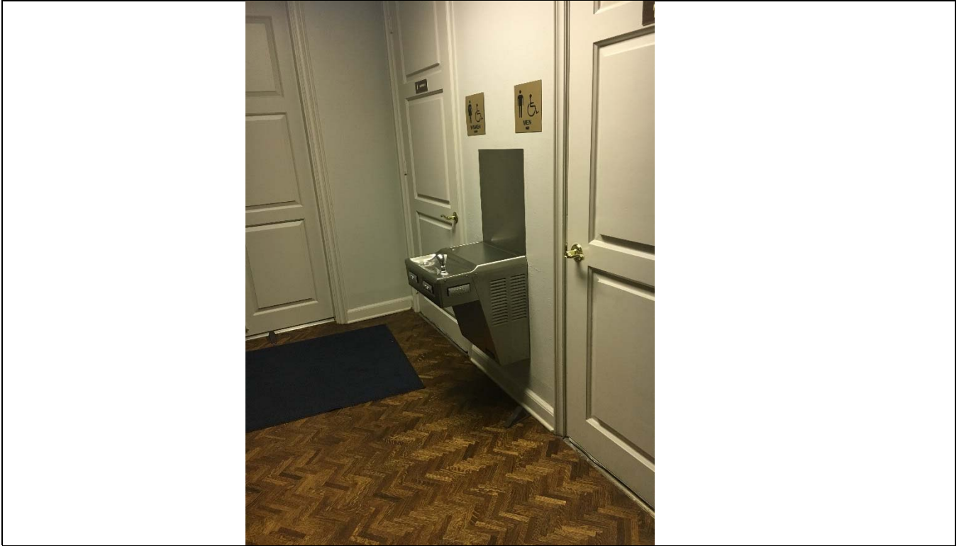
Violation 49 - The drinking fountain is a protruding object.
