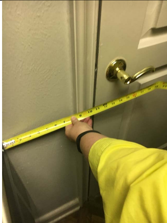
Violation 34 - Men's Room: There is only an 11" maneuvering clearance provided on the pull side of the door.
