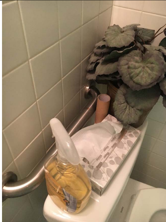
Violation 28 - Women's Room: The side grab bar has over a 2" space between the grab bar and the wall. The rear grab bar is only 12" long.
