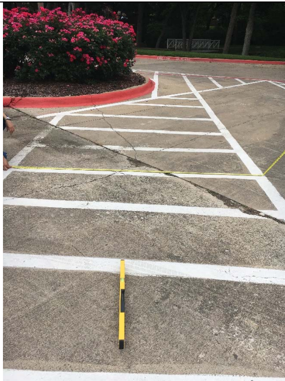
Violation 2 - The access aisle has slopes from 2.6% to 3%.
