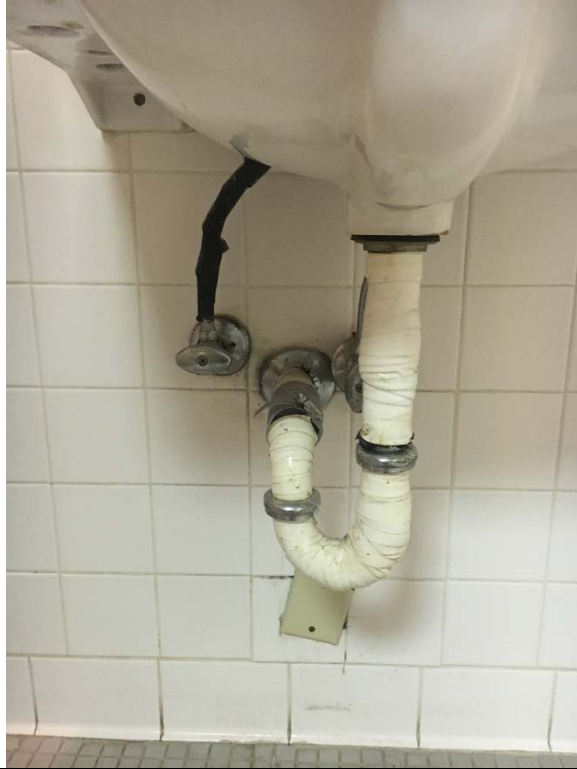
Violation 36 - Men's Room: Lavatory pipes and controls are not protected against contact.
