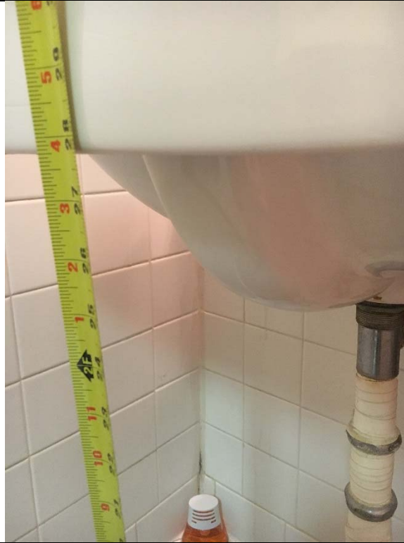
Violation 25 - Women's Room: The required knee clearance depth is not provided at the lavatory.
