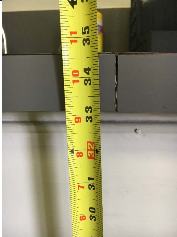
Violation 47 - Break room sink is 34-9/16" high with no knee clearance, where 34" maximum is required.
