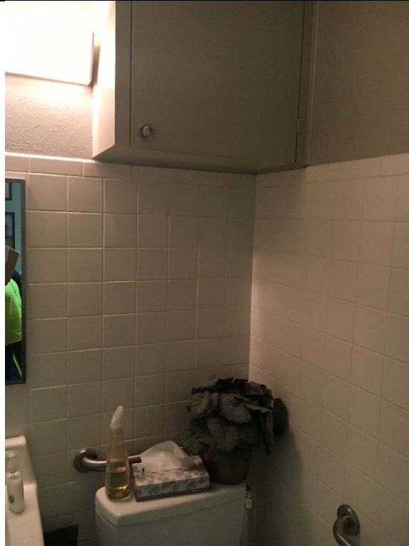
Violation 32 - Women's Room: Cabinet provided over the water closet is an overhead protrusion.
