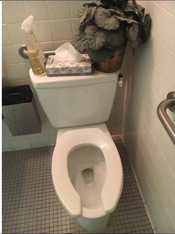
Violation 30 - Women's Room: Water closet flush control is on the closed side.
