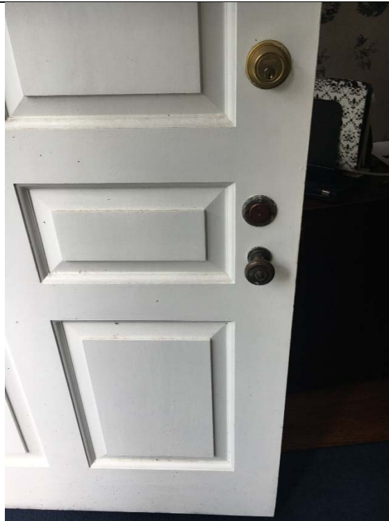
Violation 16 - There are approximately 7 doors throughout the facility with door hardware that requires grasping and twisting to operate.
