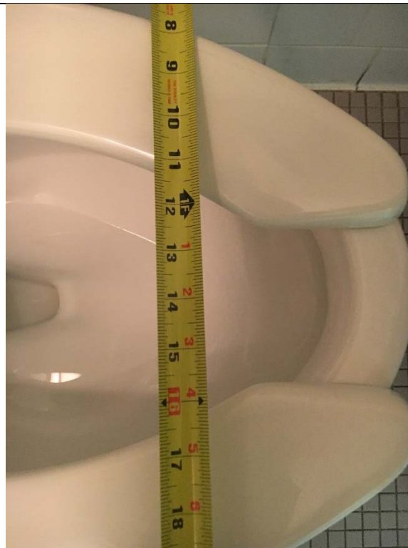
Violation 29 - Women's Room: Water closet centerline is at 14".
