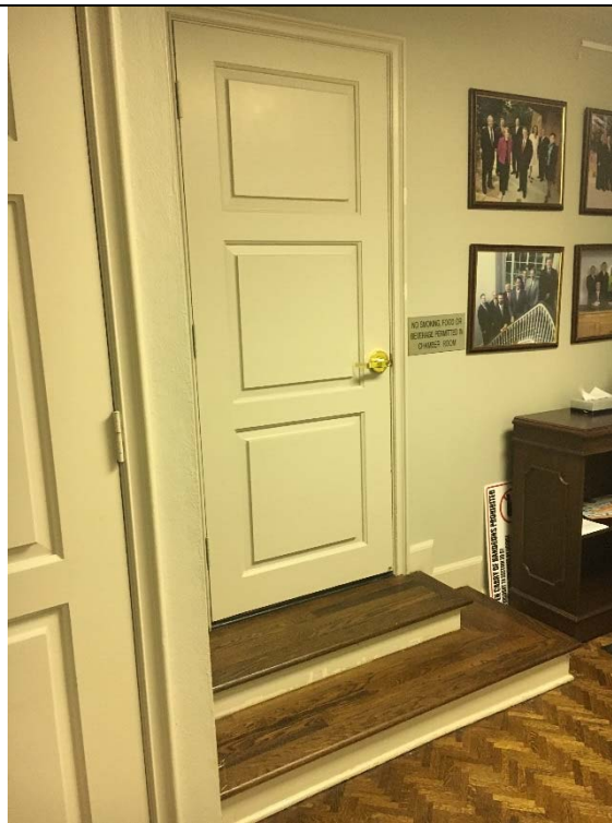
Violation 20 - Entrance into the Council of Chambers room from the office area requires steps to enter the room.
