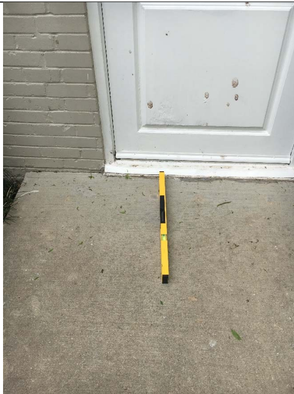
Violation 8 - The landing at the entrance to the Council of Chambers has a 10.5% running slope.
