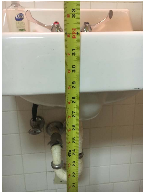
Violation 37 - Men's Room: The required knee clearance depth is not provided at the lavatory.
