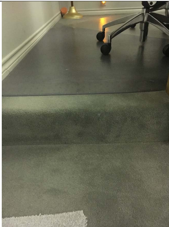
Violation 18 - There is a 6" step up to the bench seating in the council of chambers.
