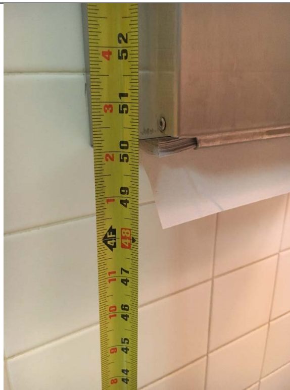
Violation 26 - Women's Room: The operation portion of the paper towel dispenser is at 50" above finished floor.
