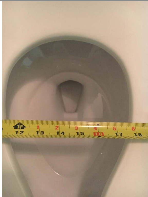
Violation 41 - Men's Room: Water closet centerline is at 14-1/2".
