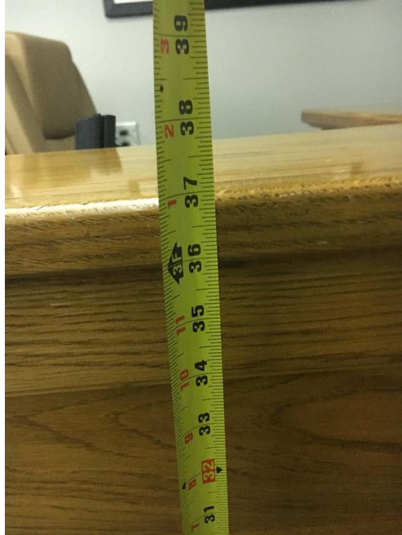
Violation 19 - The counter in the council of chambers room is too high at 37".
