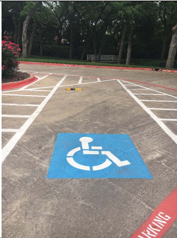
Violation 4 - There is no accessible parking signage provided.
