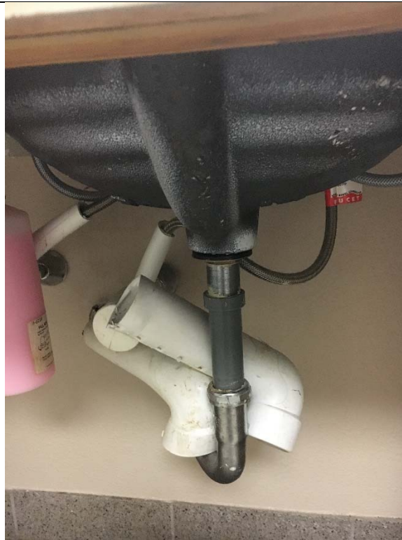
Violation 14 - Women's restroom lavatory pipes are not wrapped.
