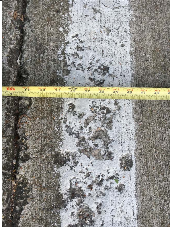
Violation 2 - The access aisle is only 38" wide and has a built up curb ramp in it.
