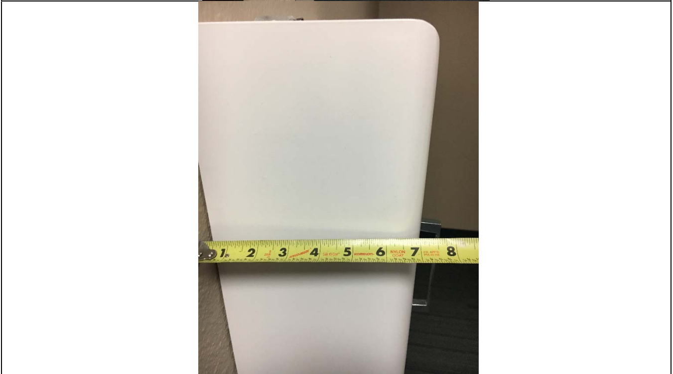
Violation 8 - The Lifepak AED box in the hallway is a protruding object protruding out 7" into the walkway at 37-5/16" above finished floor.
