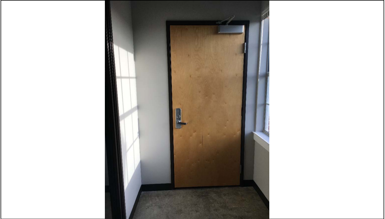
Violation 11 - Interior hallway door only has 16" maneuvering clearance on the pull side.
