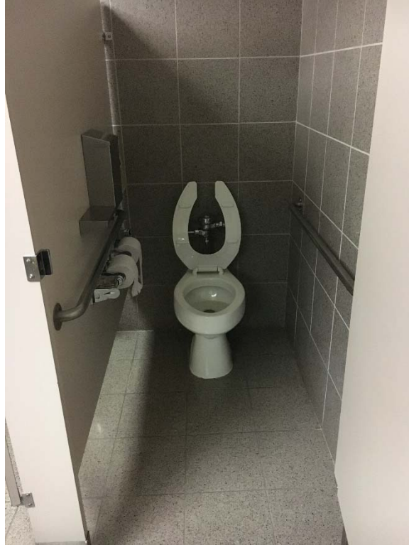
Violation 13 - There is no accessible stall provided in the Women's restroom.
