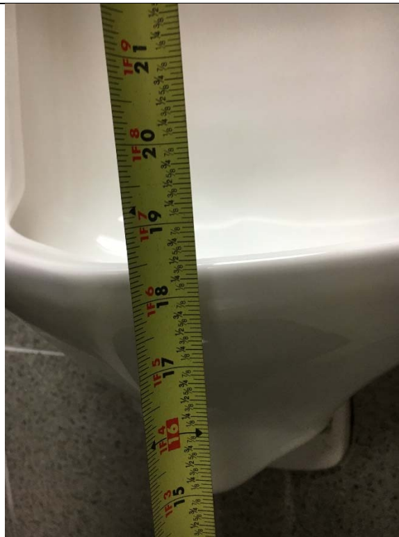
Violation 18 - Men's restroom accessible urinal is mounted at 18-1/2" to the rim where a maximum of 17" is required.
