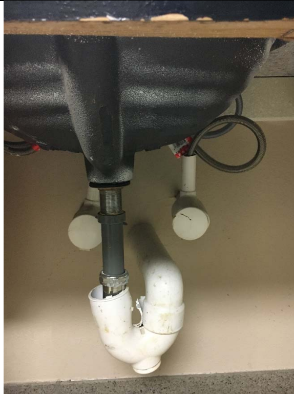
Violation 17 - Men's restroom lavatory pipes are not wrapped.
