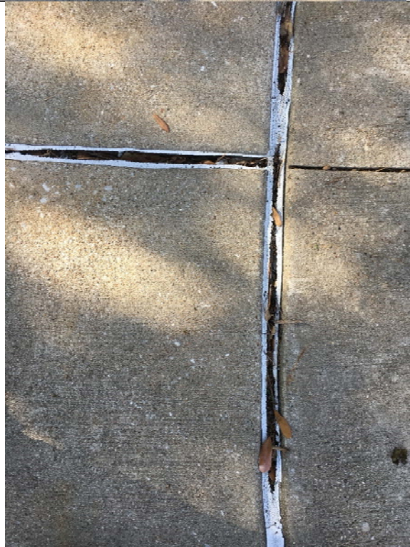
Violation 7 - The caulking around the joint of the gazebo is cracked and causes level changes exceeding 1/2".
