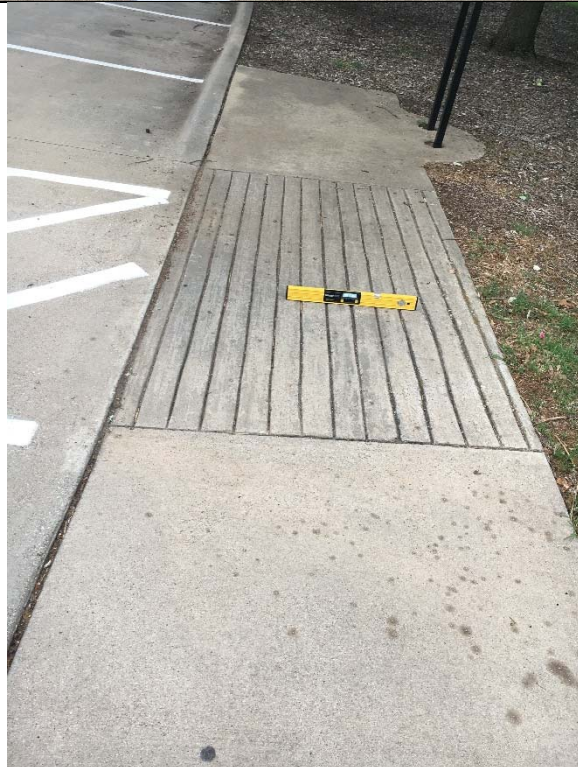
Violation 5 - Neither curb ramp has a level landing at the top.
