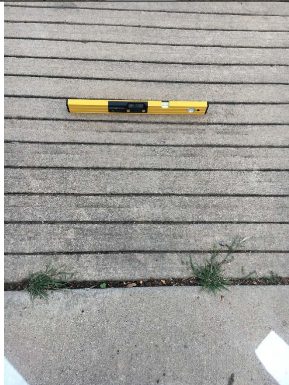
Violation 4 - Both curb ramps have gaps where the ramp meets the access aisle.
