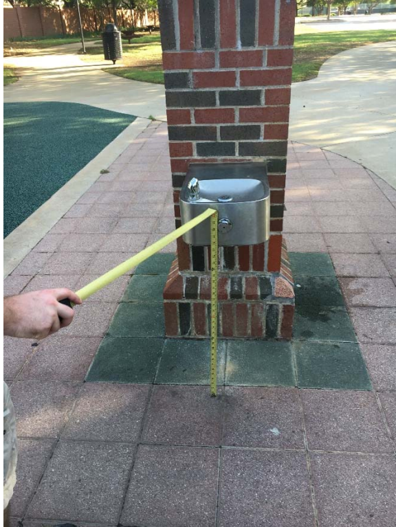
Violation 8 - There is no drinking fountain provided for standing persons.
