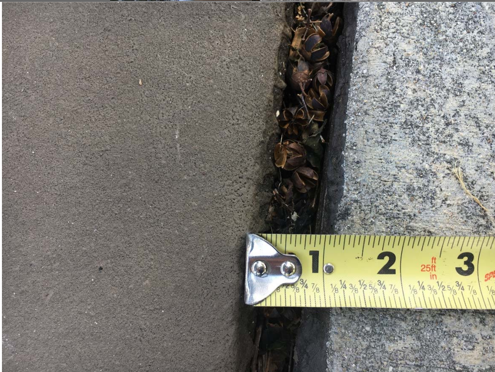
Violation 11 - There is a 1" gap at the transition from the sidewalk to the tennis court.
