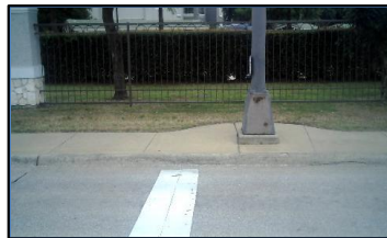
Corner 4 No Ramp (4z)
