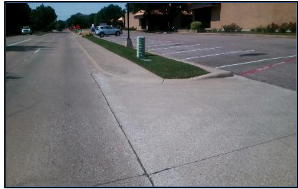
Corner 4 No Ramp (4z)
