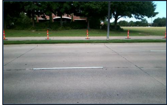
Corner 4 No Ramp (4z)
