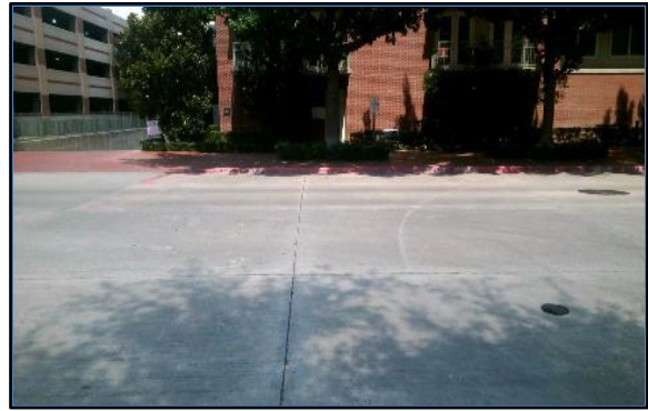
Corner 2 No Ramp (2z)
