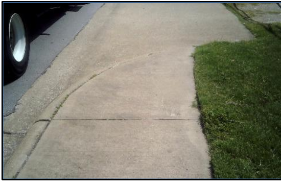
Corner 1 No Ramp (1z)
