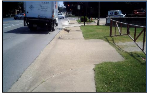
Corner 4 No Ramp (4z)
