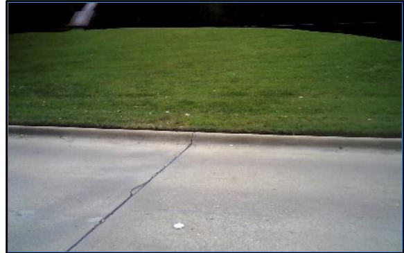
Corner 4 No Ramp (4z)
