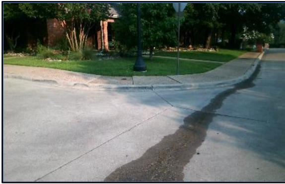
Corner 1 No Ramp (1z)
