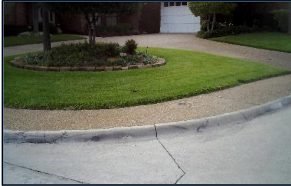
Corner 3 No Ramp (3z)
