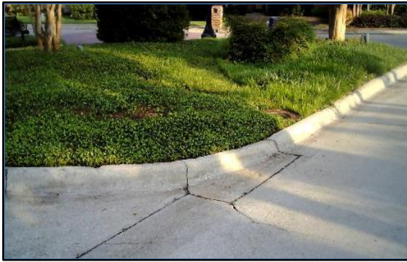
Corner 1 No Ramp (1z)
