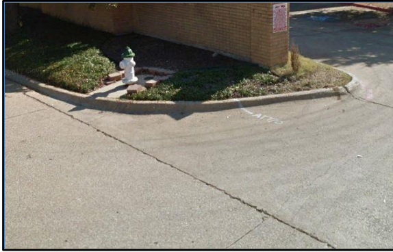
Corner 3 No Ramp (3z)
