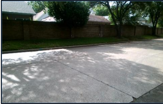
Corner 3 No Ramp (3z)
