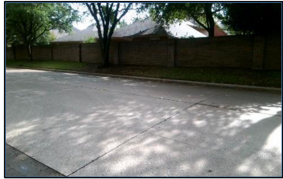
Corner 2 No Ramp (2z)
