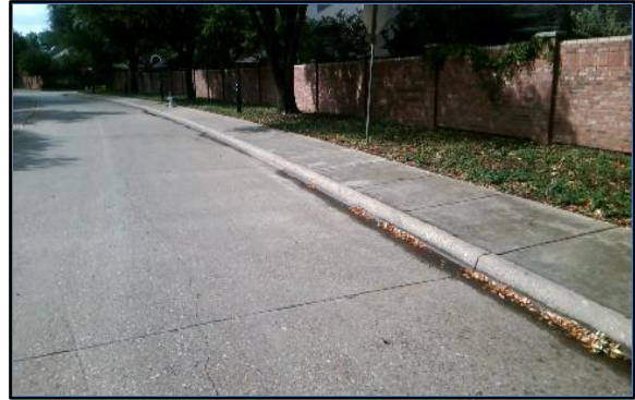
Corner 4 No Ramp (4z)
