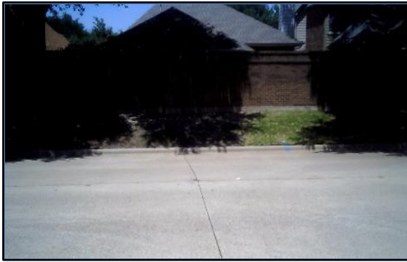
Corner 1 No Ramp (1z)
