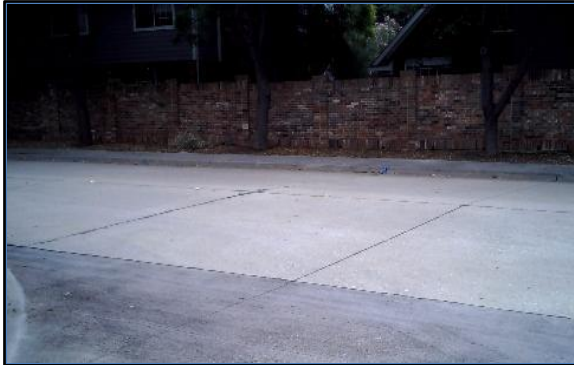
Corner 3 No Ramp (3z)
