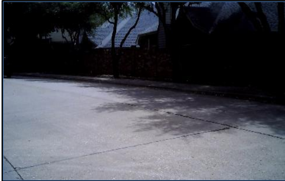
Corner 3 No Ramp (3z)
