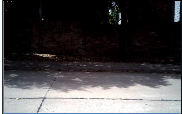
Corner 4 No Ramp (4z)
