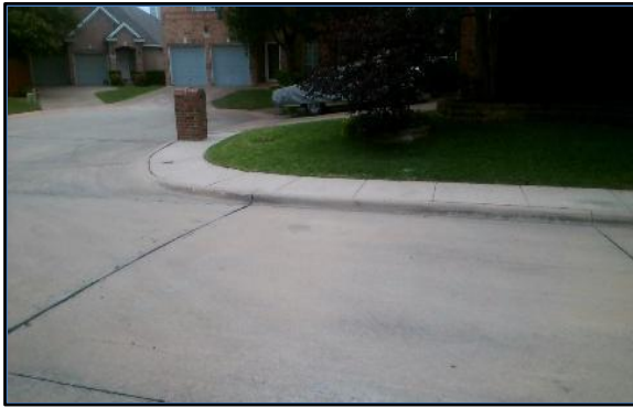
Corner 1 No Ramp (1z)
