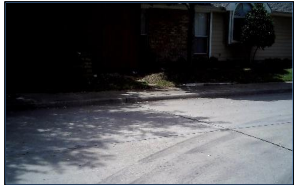
Corner 4 No Ramp (4z)
