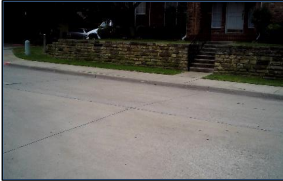
Corner 3 No Ramp (3z)
