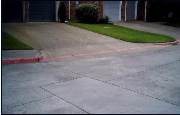
Corner 3 No Ramp (3z)
