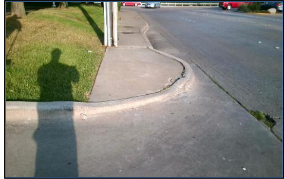
Corner 4 No Ramp (4z)
