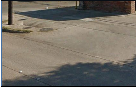
Corner 3 No Ramp (3z)
