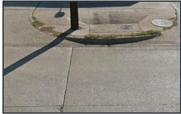
Corner 4 No Ramp (4z)
