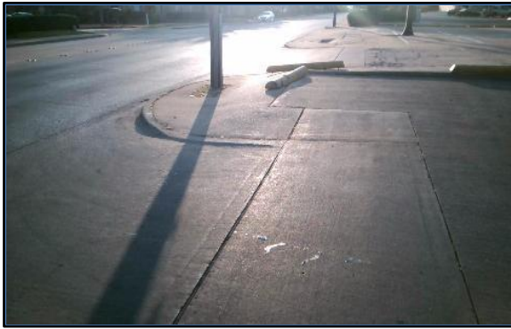
Corner 3 No Ramp (3z)
