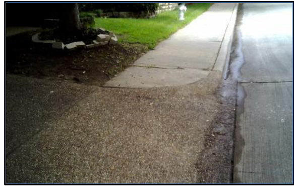
Corner 2 No Ramp (2z)
